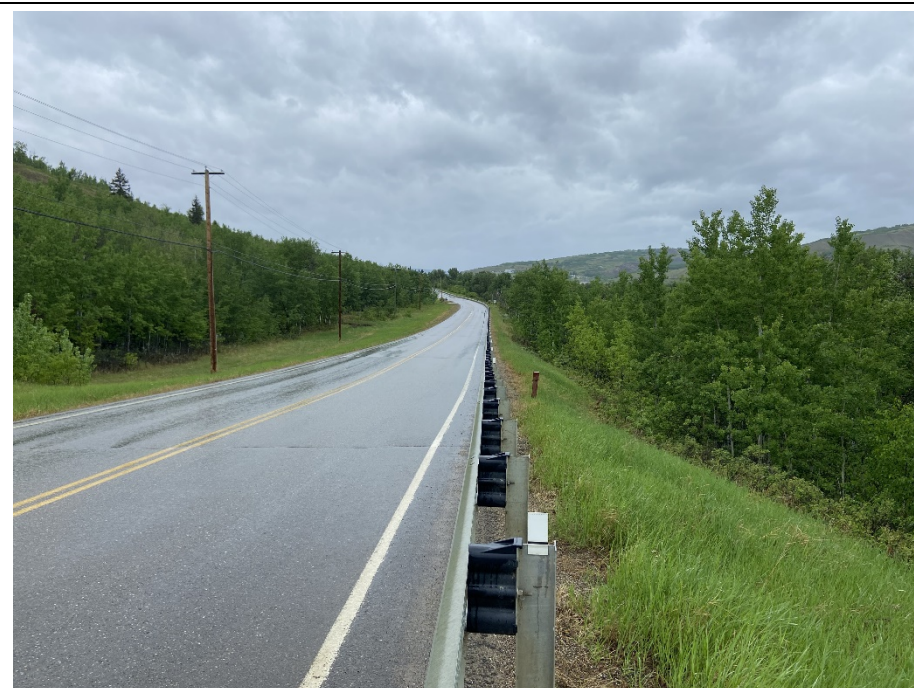
Photo 4. Looking north at the slide at km 28.6. No visible changes to the slope below the road. No change to pavement damage or dip at the guardrail except for a new transverse crack noted south of the road section with previous cracking prior to the 2021 overlay.
