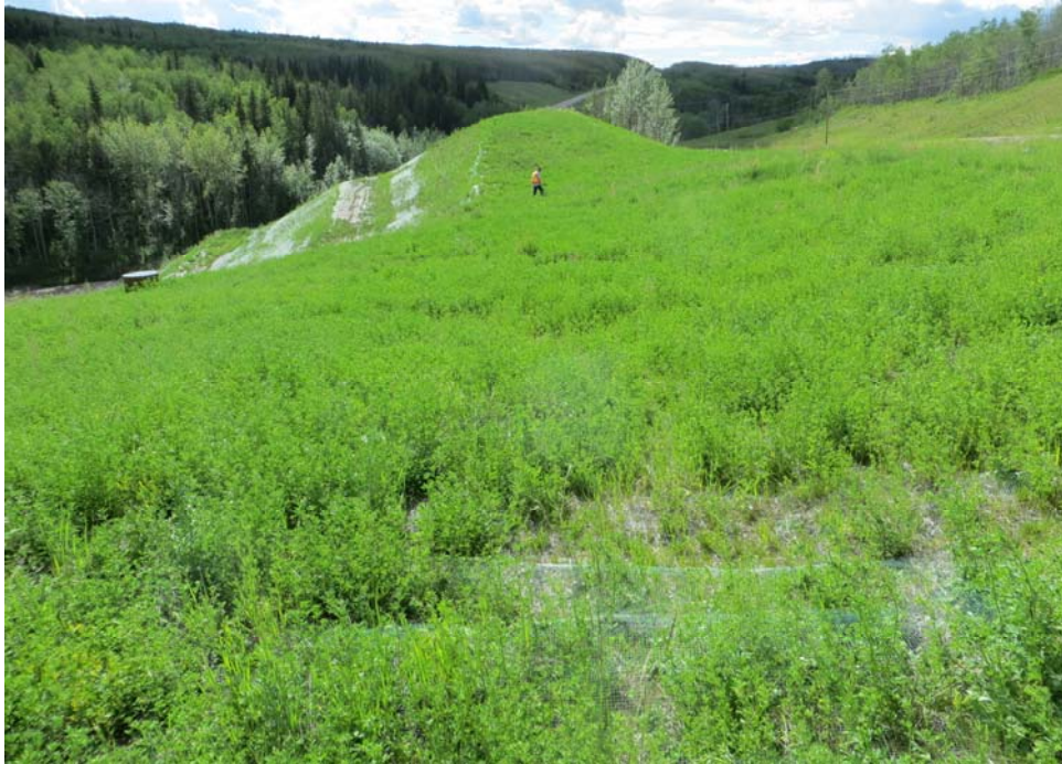
Photo 9 – Looking west along the south embankment of Site B. Note the benched hillside in the background and the subsidence near to the highway over the culvert.
