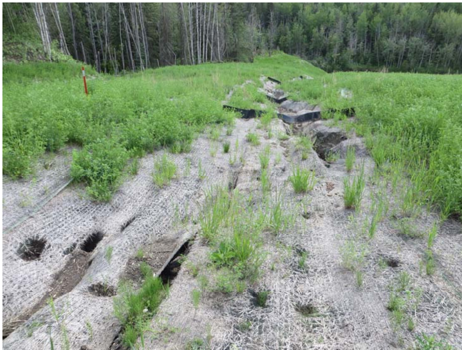
Photo 8 - Looking at the surface erosion through the existing erosion control soil covering and ditch barriers on the south embankment of Site B.
