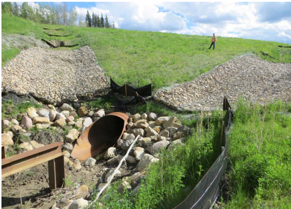
Photo 14 - Looking south at the culvert inlet area north of the highway at Site B. Note the severe ditch erosion up-gradient of the gabions.
