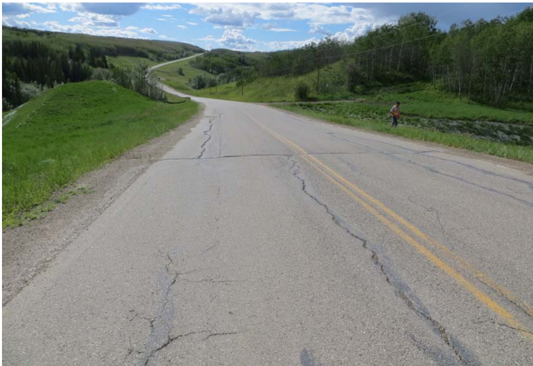
Photo 12 - Looking west along the highway at the dip and cracks of Site B.
