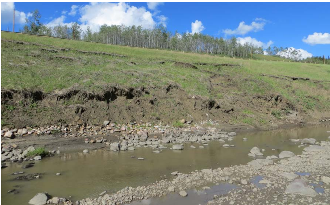
Photo 2 – Looking northeast from the Creek up at the slide at Site A in the south highway embankment.
