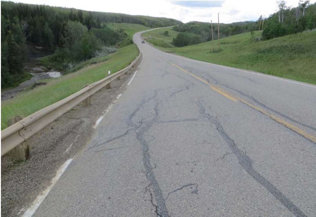
Photo 5 – Looking west along the highway at the crack/dip in the highway above Slide A.
