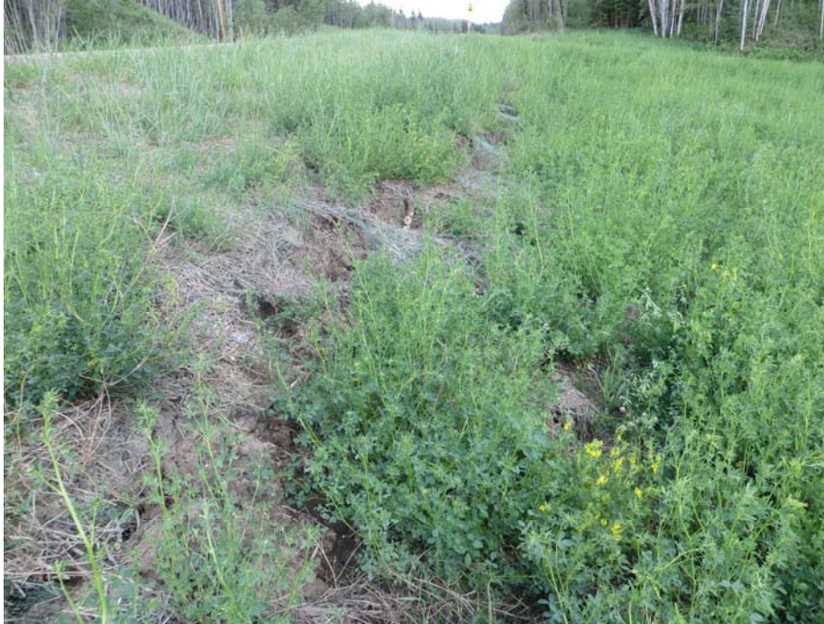
Photo 7 – Looking east at the slide scarp adjacent to the highway in the south embankment of Site B.
