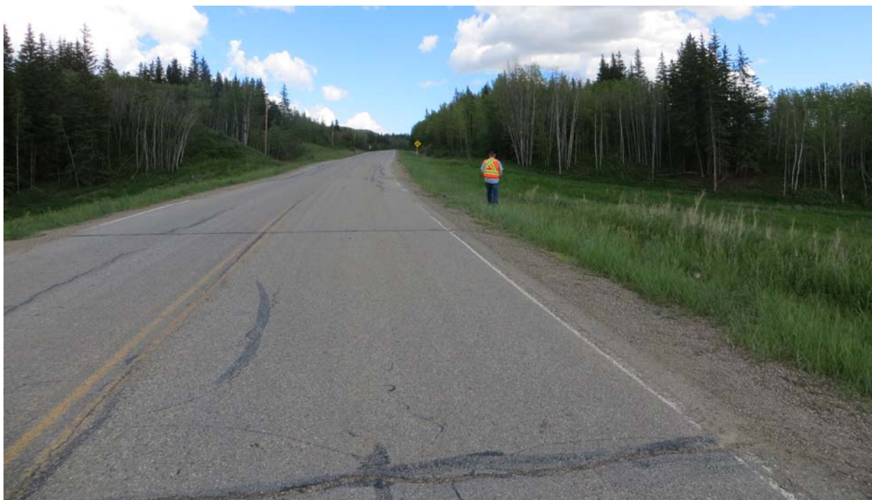
Photo 6 - Looking east along the highway and south embankment Site B. Note the settlement in both the highway and the embankment.
