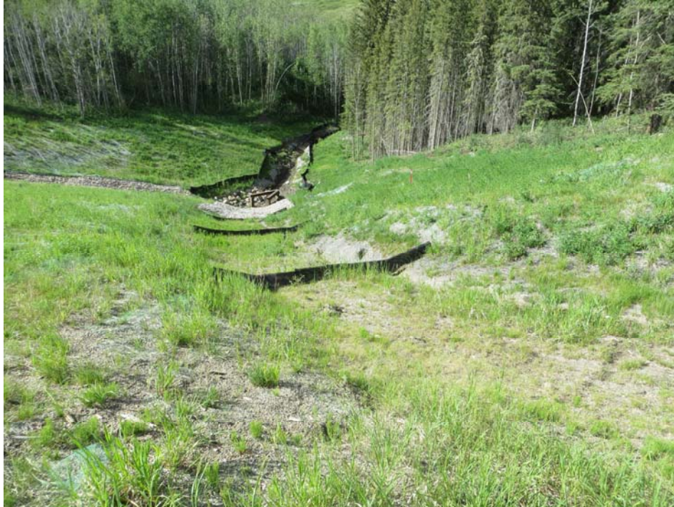
Photo 13 – Looking north along the east ditch of the north embankment of Site B.
