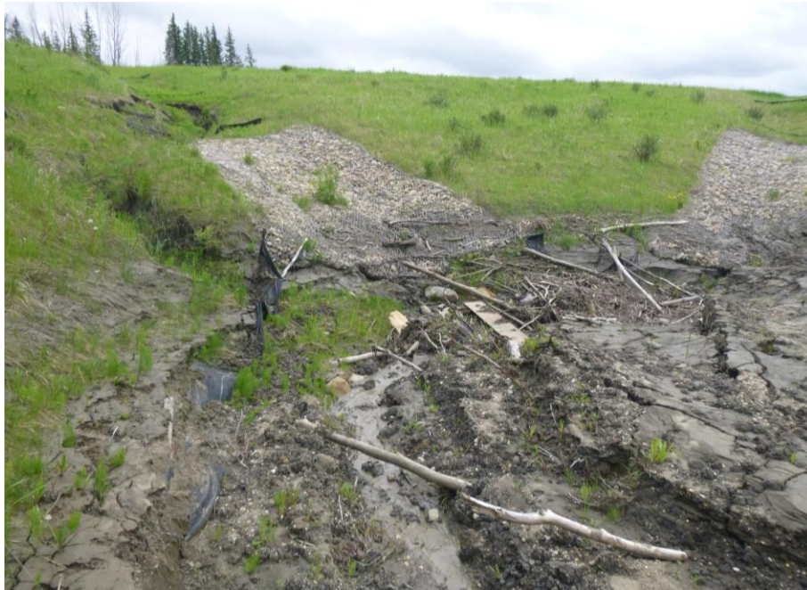
Photo 11 – Looking south at the culvert inlet area of the north embankment of PH77-2. Note the infilled channel with logs and debris, which has completely covered the trash rack and culvert inlet.
