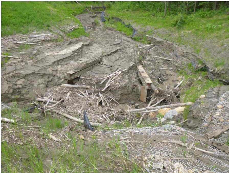
Photo 12 - Looking north along the infilled channel leading into the culvert inlet north of the highway at PH77-2.
