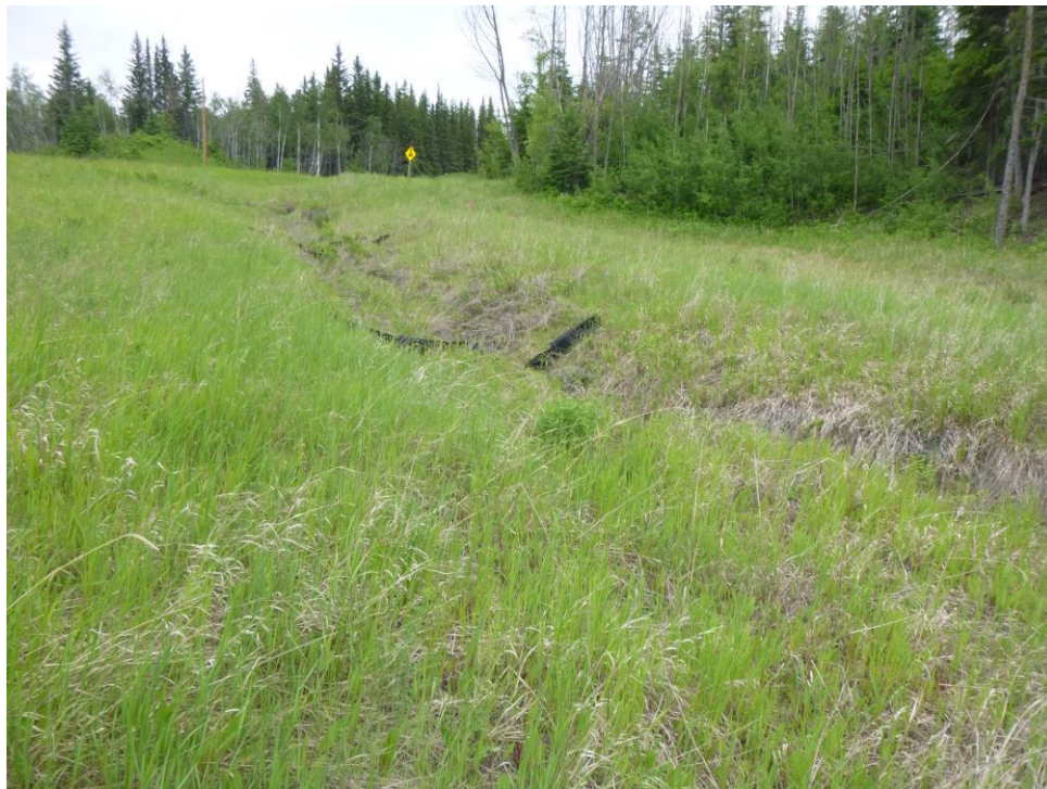
Photo 6 – Looking north along the eroded TRM ditch channel of PH77-2.
