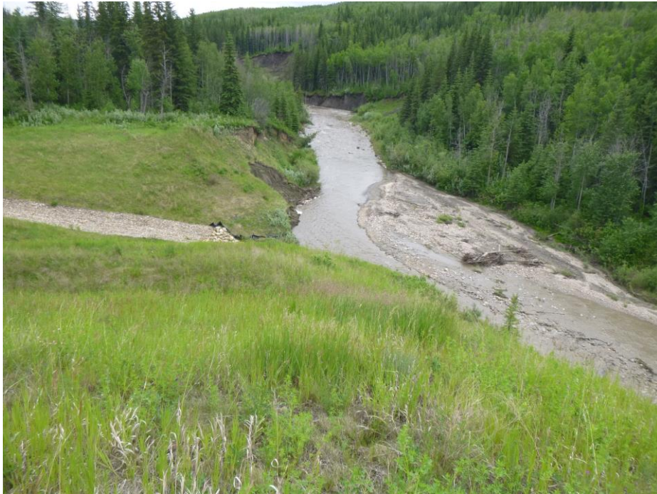
Photo 9 - Looking southeast at the culvert outlet area of PH77-2. Note the riverbank slumping east of the culvert outlet.
