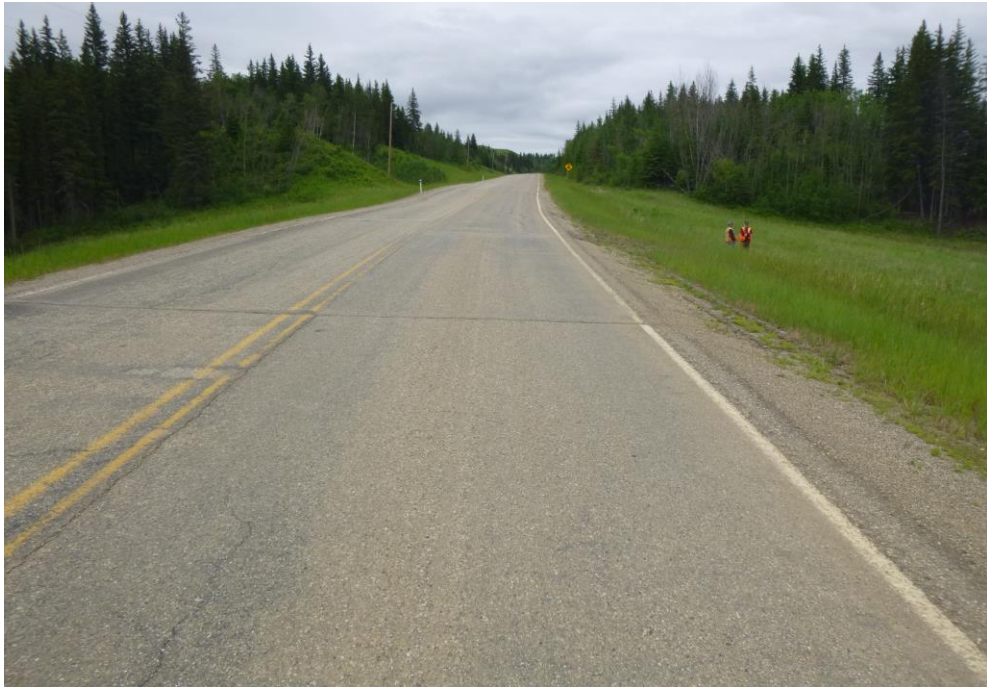
Photo 5 - Looking east along the highway across PH77-2. Note the settlement and cracking in the highway.
