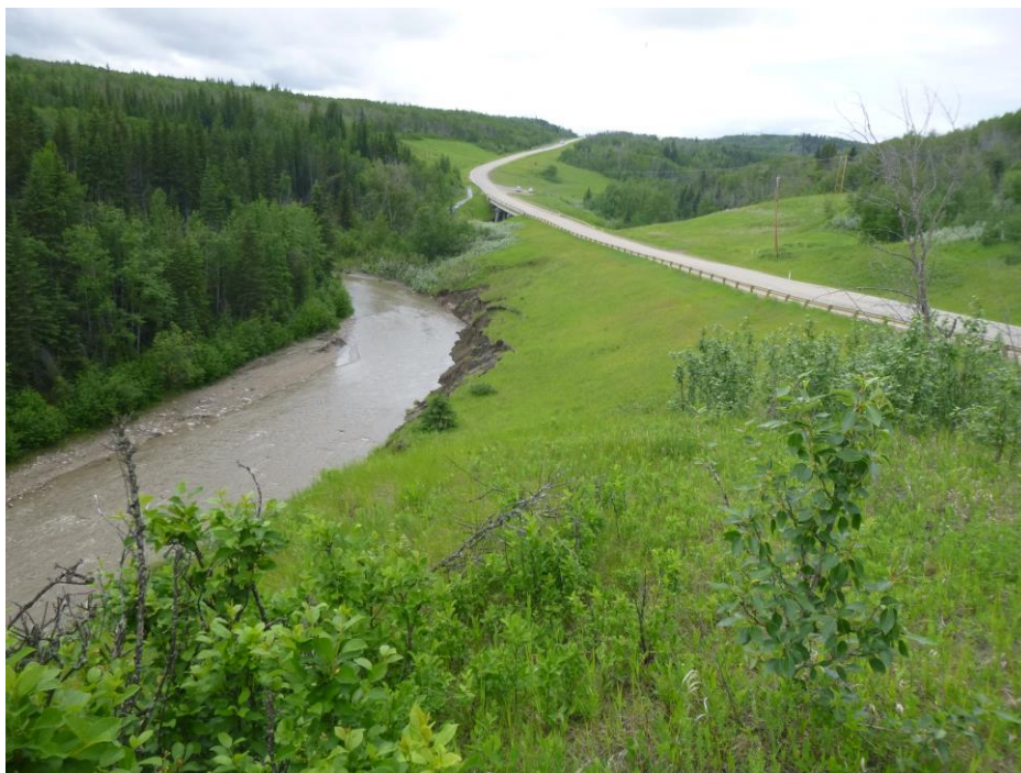
Photo 2 – Looking west at the fresh toe slumping above the creek at PH77-1 in the south highway embankment.
