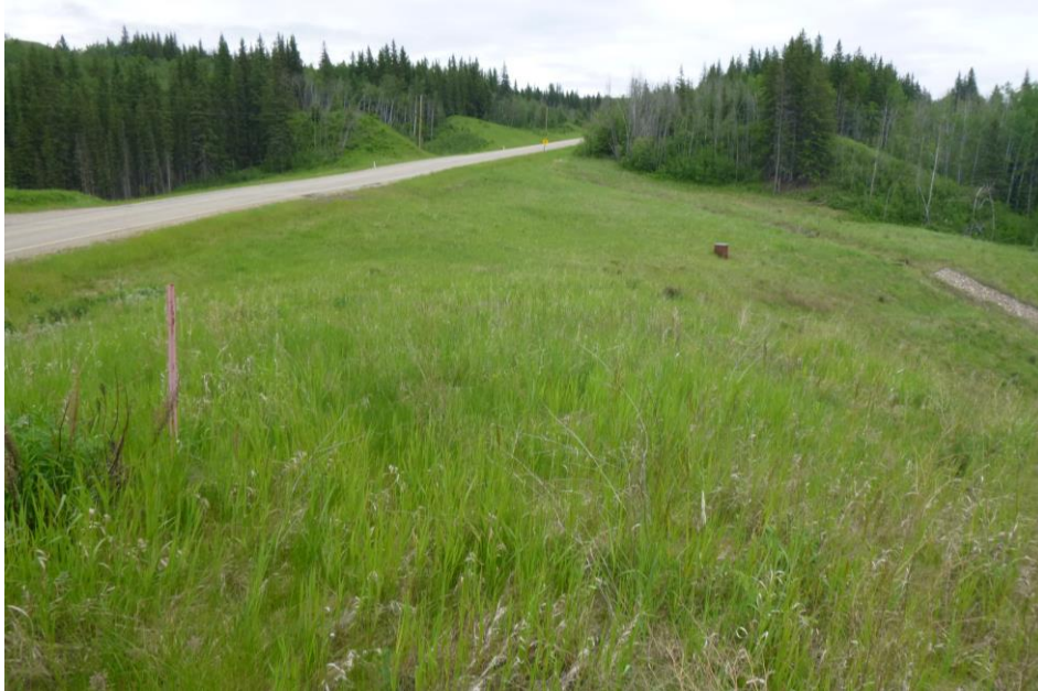
Photo 7 - Looking east along the south hwy embankment and southeast ditch drainage channel of PH77-2, Hines Creek.
