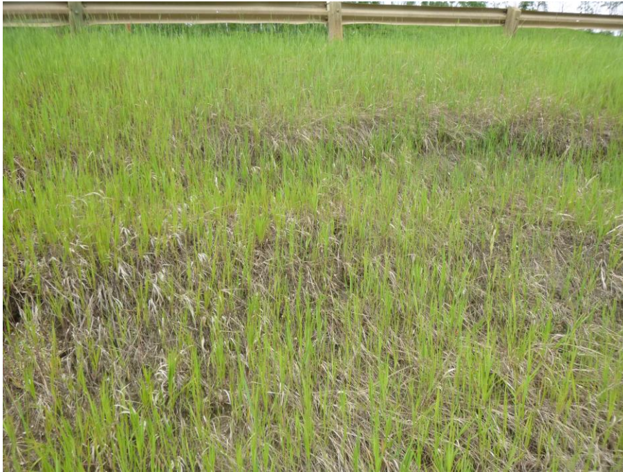
Photo 3 – Looking north upslope at the slide scarp adjacent to the highway at PH77-1.
