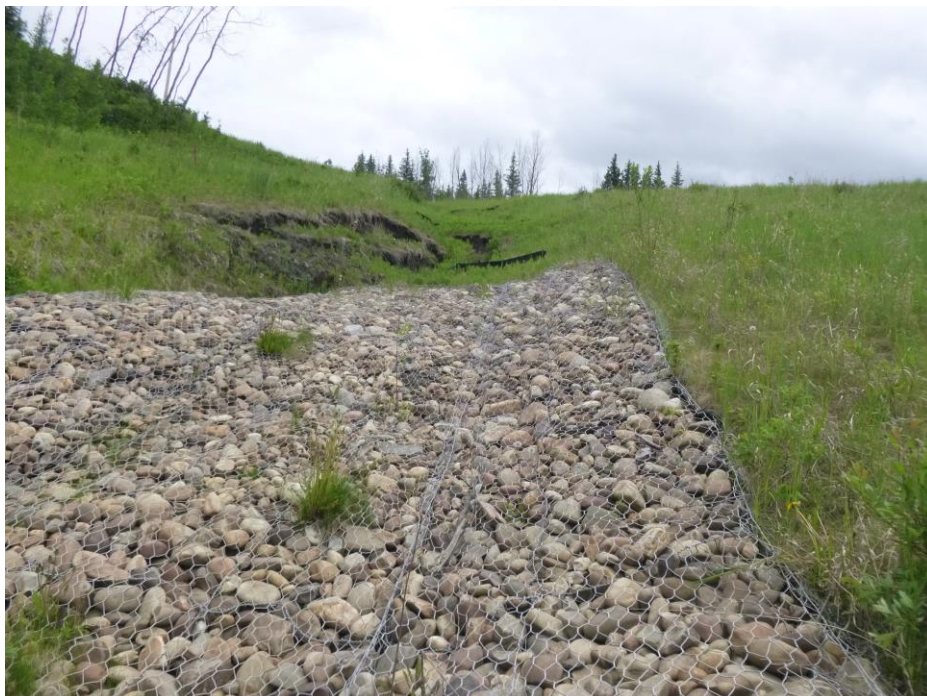
Photo 10 – Looking south at the erosion along the northeast ditch crotch leading to the culvert inlet area of the north embankment of PH77-2.
