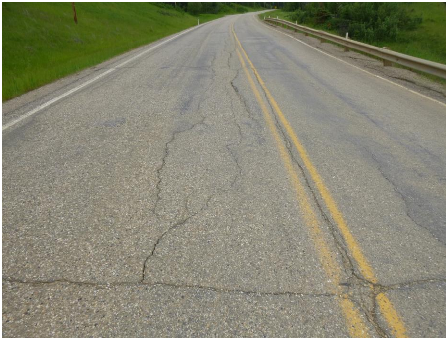
Photo 4 - Looking east along the highway at the crack/dip in the highway above the Slide at PH77-1.
