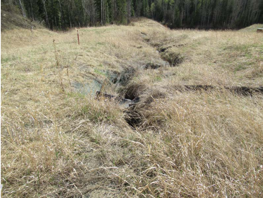
Photo 7 – Looking south along the eroded TRM ditch channel of PH77-2.
