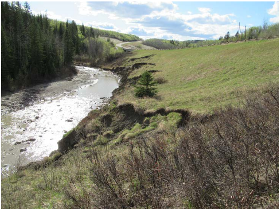
Photo 2 – Looking west at the slumping above the creek at PH77-1 in the south highway embankment.
