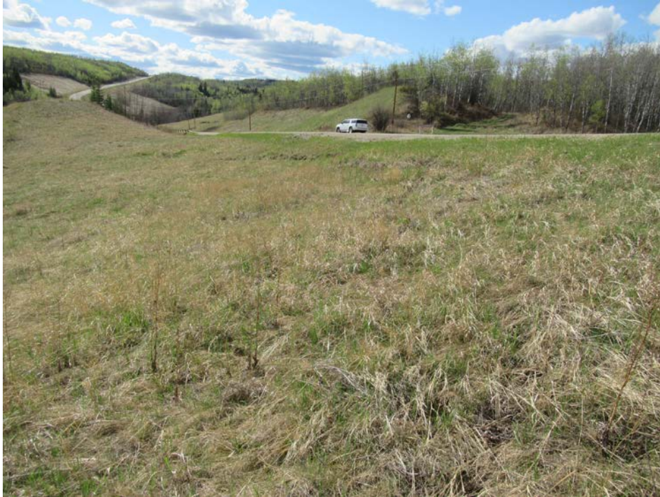
Photo 9 – Looking west across the south embankment of PH77-2, at the slide scarp in proximity to the highway.
