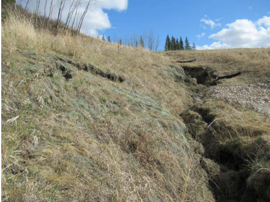
Photo 11 – Looking southeast at the erosion along the northeast ditch crotch leading to the culvert inlet area of the north embankment of PH77-2.
