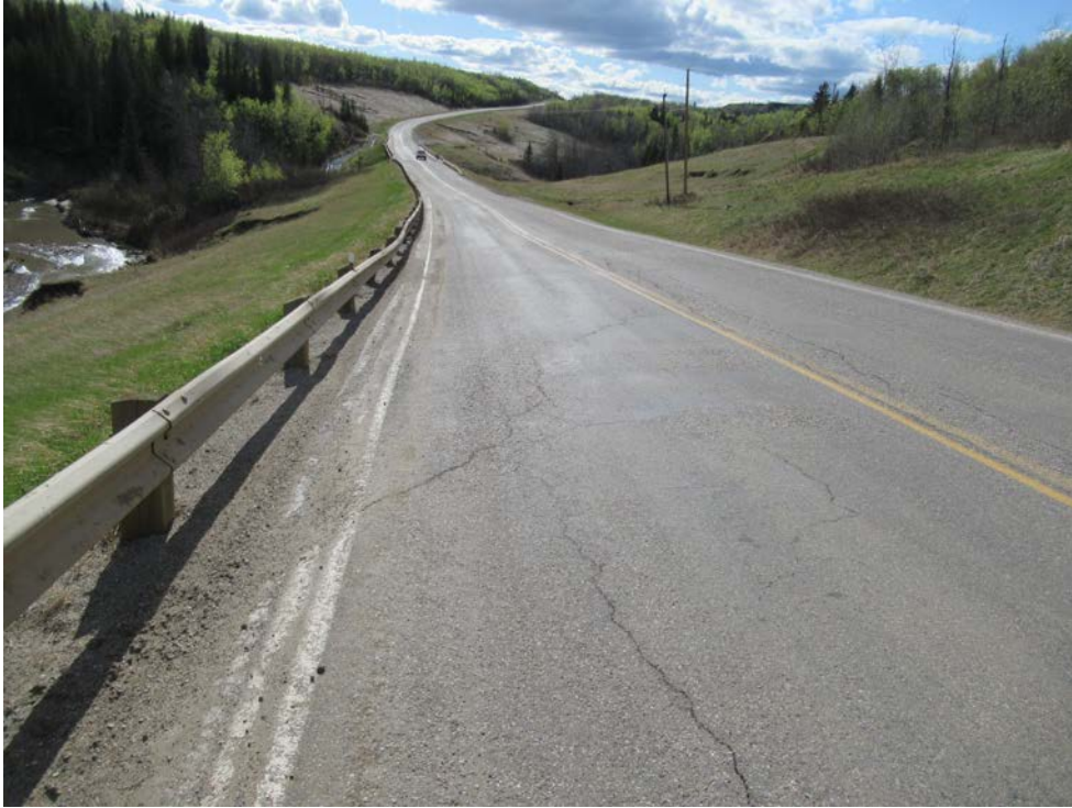
Photo 5 – Looking east along the highway at the crack/dip in the highway above the Slide at PH77-1.
