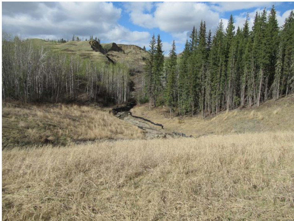
Photo 14 - Looking north at the severe channel erosion leading into the culvert inlet, and the eroded ditch crotch channels above the culvert inlet area north of the highway at PH77-2.
