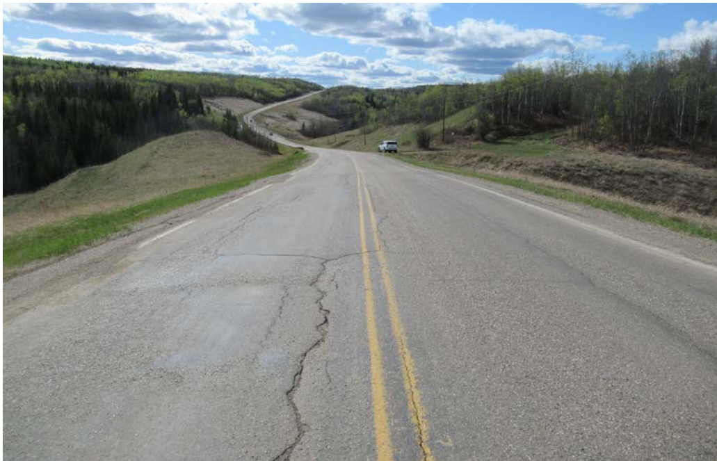
Photo 6 - Looking west along the highway across PH77-2. Note the settlement and cracking in the highway.
