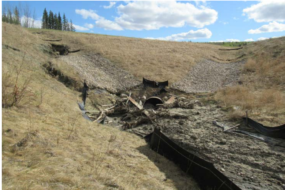
Photo 13 – Looking south at the culvert inlet area of the north embankment of PH77-2. Note the undermining of the end of the gabions and associated ditch channel slumping.
