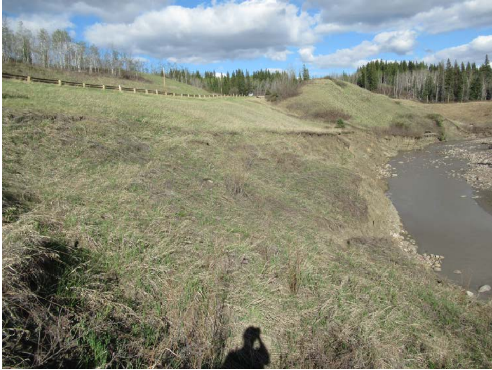
Photo 1 – Looking east at Slide PH77-1 at the active erosion along the north side of the Creek.
