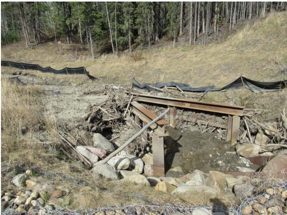
Photo 12 - Looking northeast at the culvert inlet area north of the highway at PH77-2. Note the debris accumulation around the trash rack that is nearly blocking flow.
