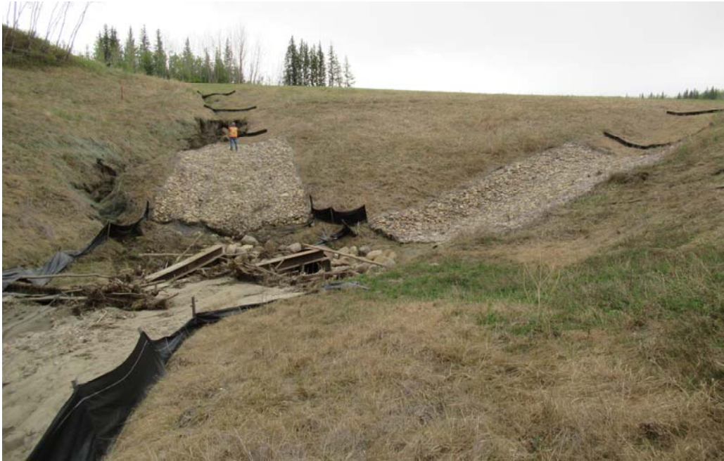
Photo 13 – Looking south at the culvert inlet area of the north embankment of PH77-2. Note the undermining of the end of the gabions and associated ditch channel slumping.
