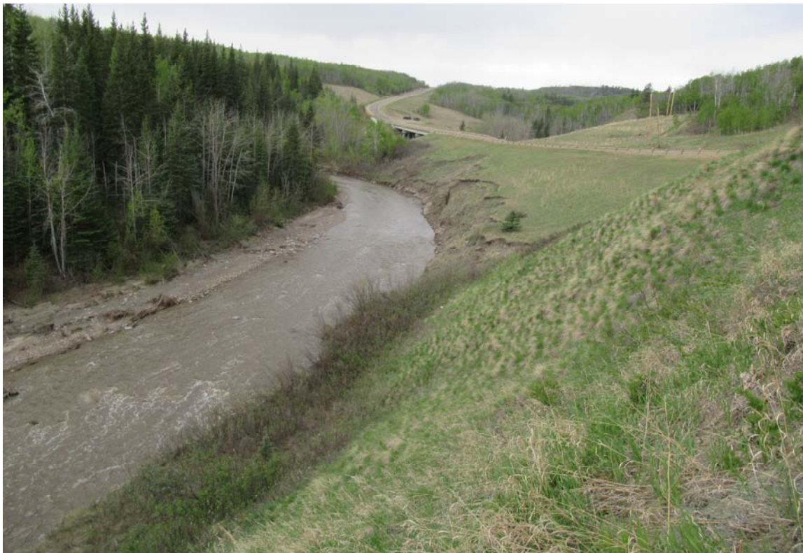
Photo 4 - Looking west along the Creek at the erosion at PH77-1.
