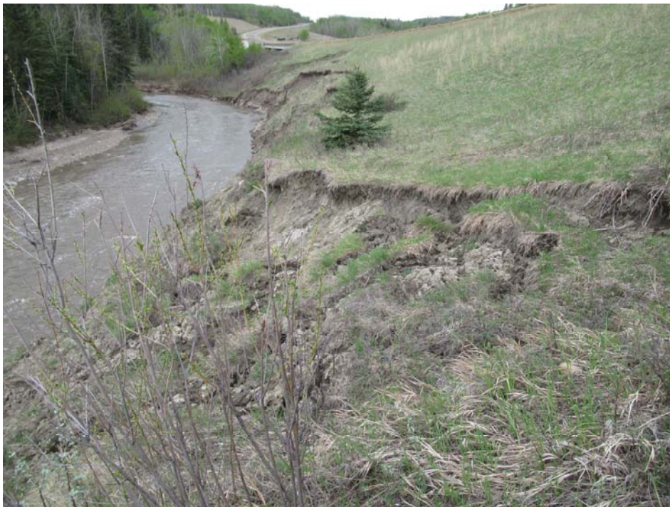
Photo 2 – Looking west at the slumping above the creek at PH77-1 in the south highway embankment.
