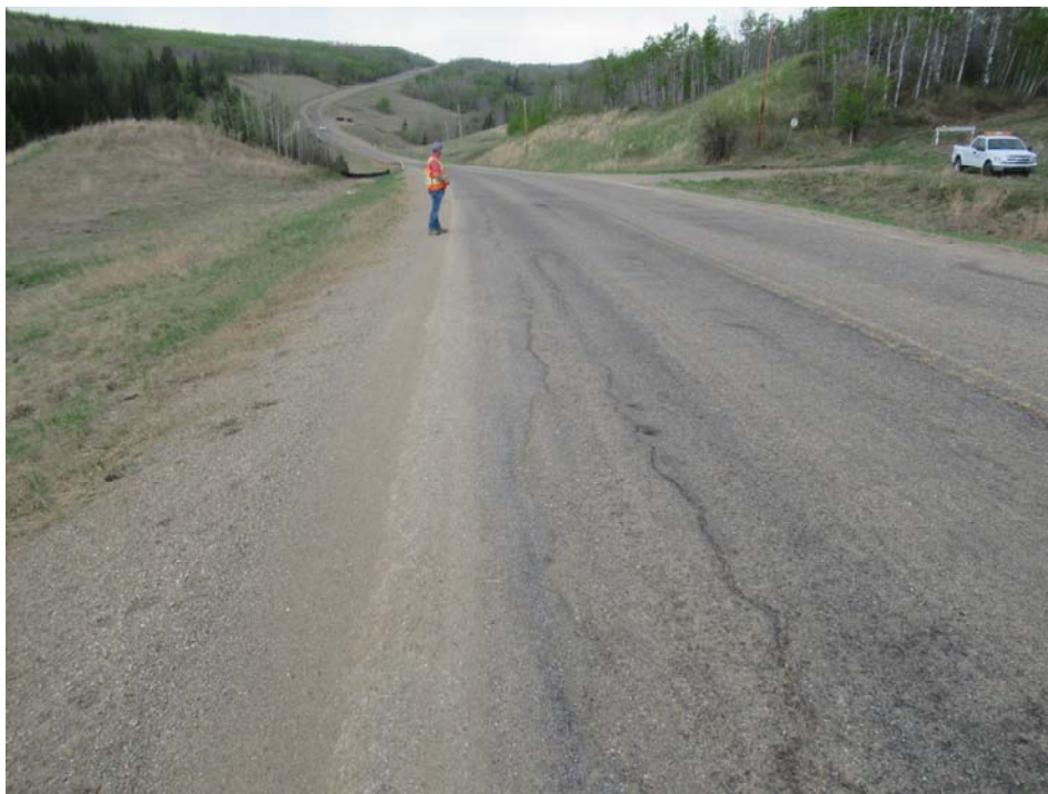
Photo 6 - Looking west along the highway and south embankment of PH77-2. Note the settlement in both the highway and the embankment.
