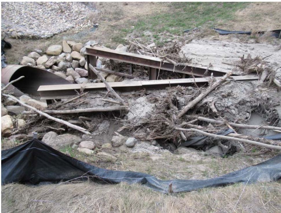
Photo 12 - Looking west at the culvert inlet area north of the highway at PH77-2. Note the debris accumulation around the trash rack from the extreme 2018 spring flow.
