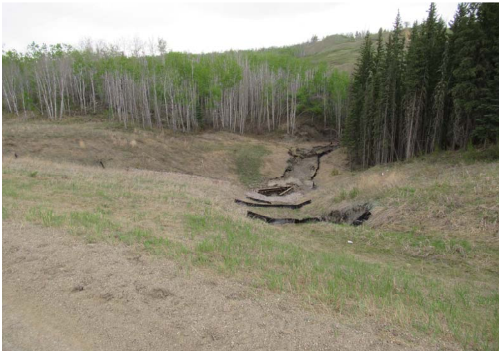
Photo 14 - Looking north along the eroded northeast TRM ditch crotch channel above the culvert inlet area north of the highway at PH77-2. Note the severe channel erosion leading into the culvert inlet in the background.
