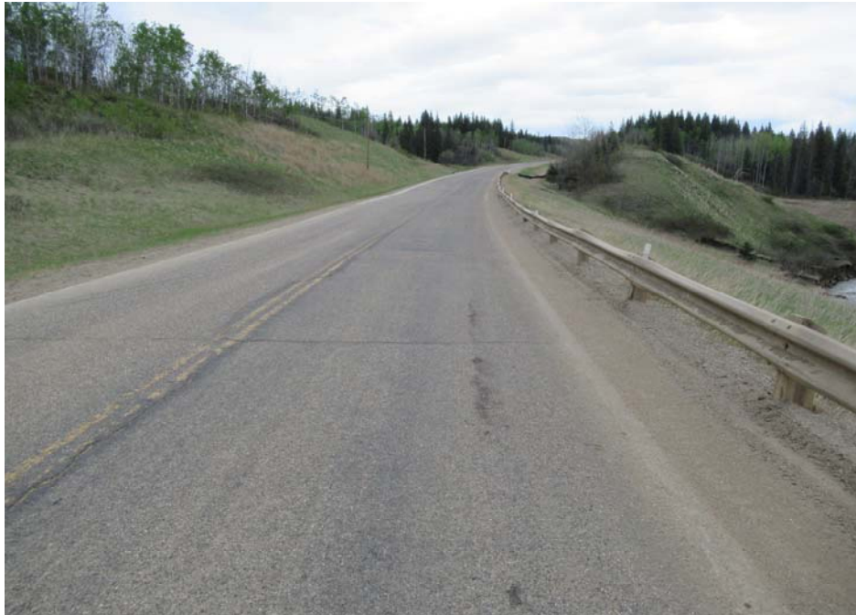
Photo 5 – Looking east along the highway at the crack/dip in the highway above the Slide at PH77-1.
