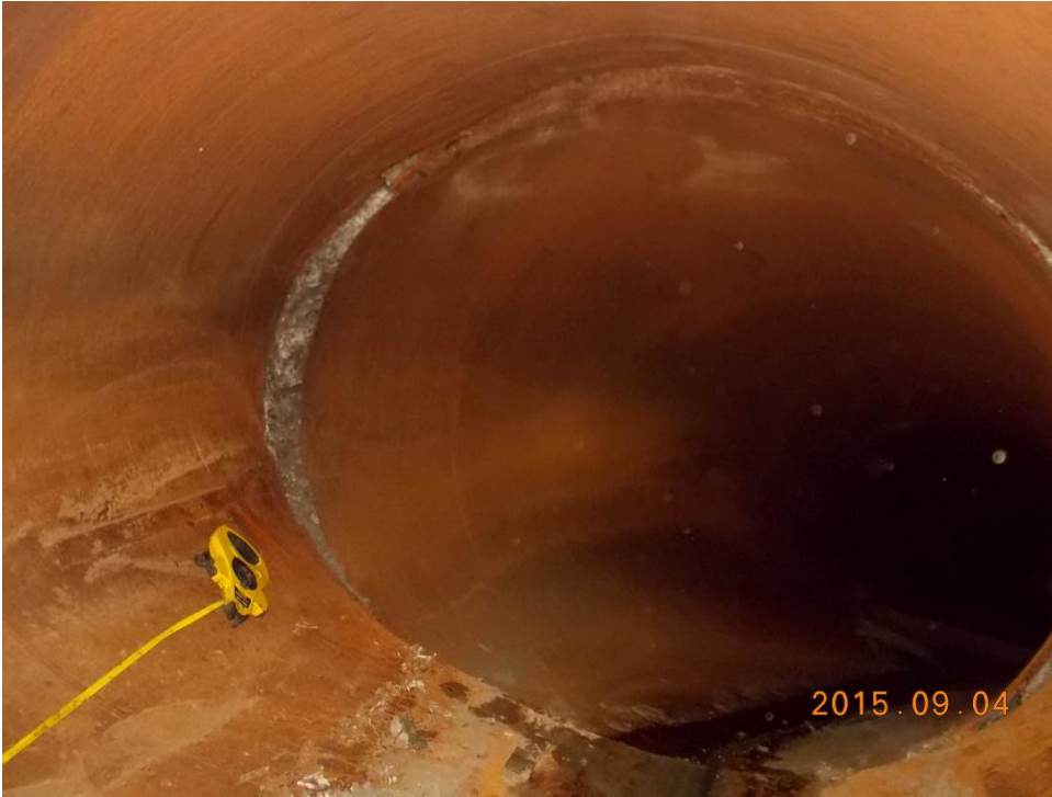
View of typical deflection 3 m d/s from access hole
