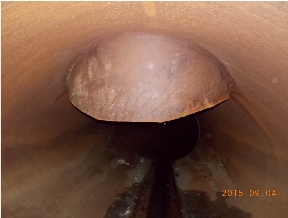
View of typical deflection looking at access hole
