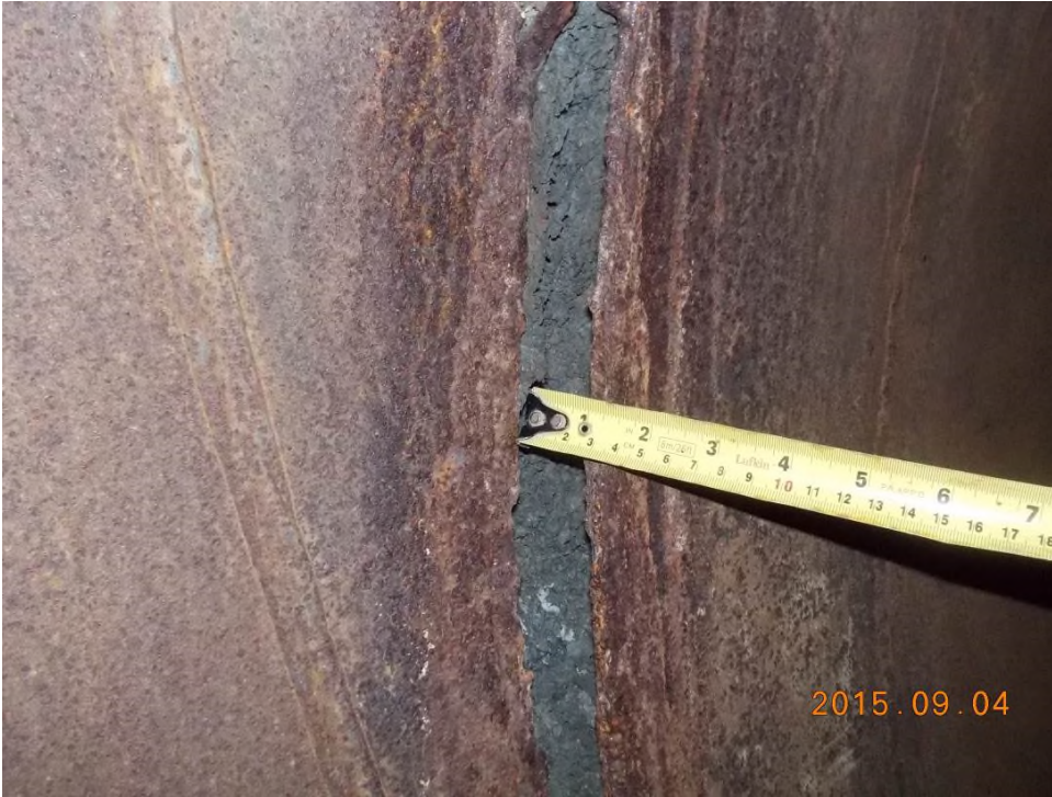
23 mm crack along circumferential seam approx. 67 m from u/s end
