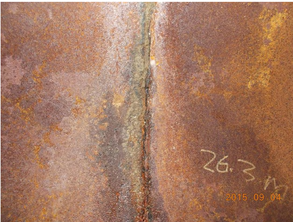
10 mm crack along circumferential seam approx. 26.3 m from u/s end
