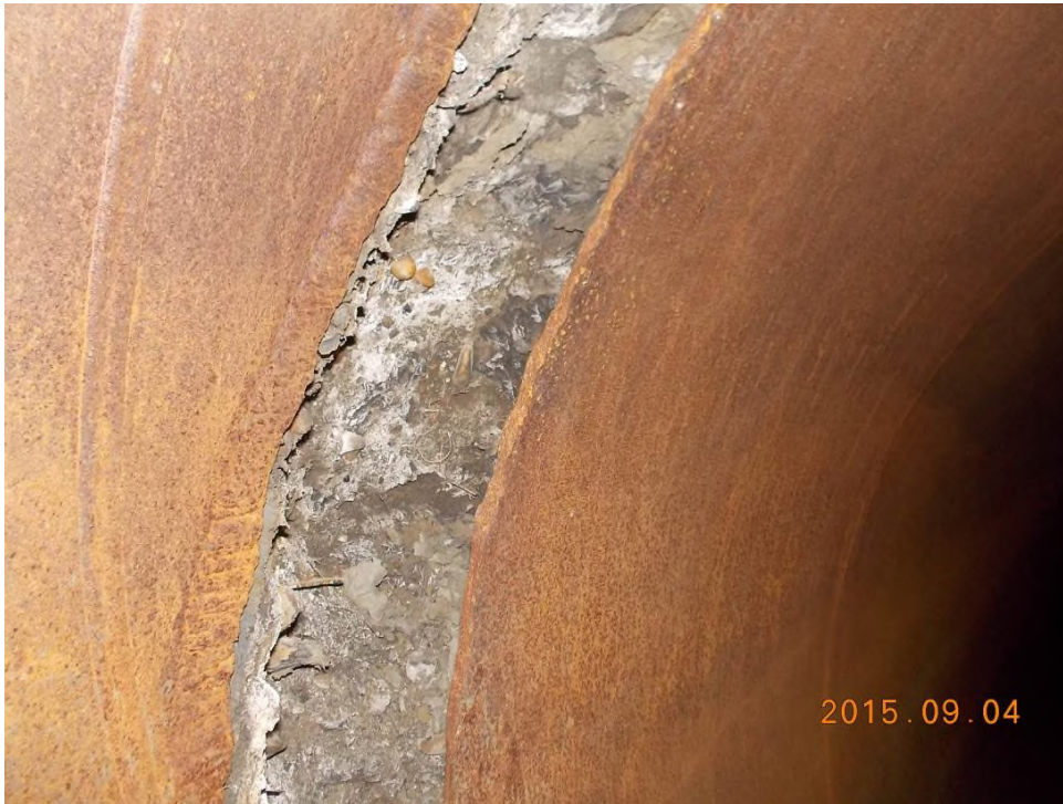
100 mm crack along circumferential seam approx. 93 m from u/s end
