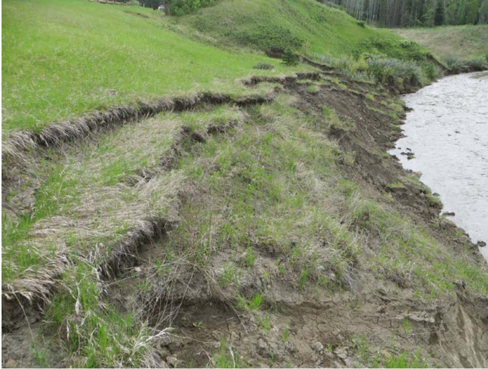
Photo 1 – Looking east at Slide site 1 at active erosion along the north side of the Creek.
