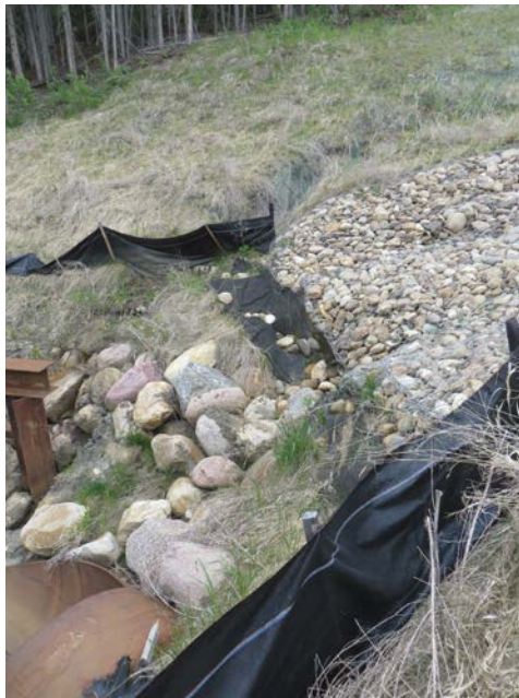
Photo 14 - Looking west at the culvert inlet area north of the highway at Site 2. Note the undermining of the end of the gabion ditch channel, and the slumping above.
