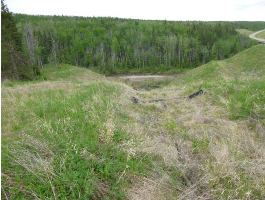
Photo 9 – Looking southwest down along the south embankment and ditch channel of Site 2. Note the erosion and the benched hillside to the west.
