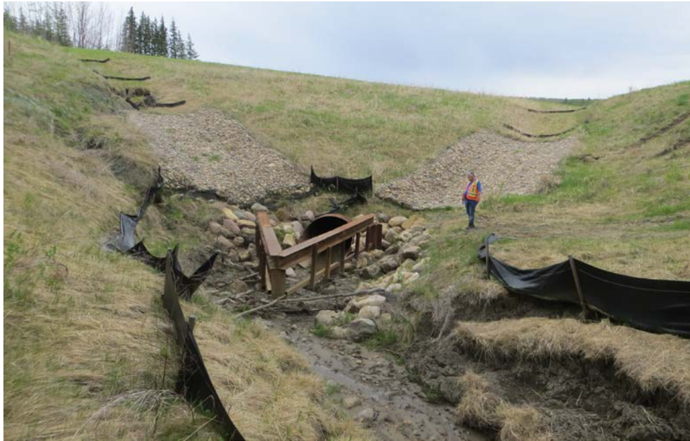
Photo 15 – Looking south across the culvert inlet area of the north embankment of Site 2. Note the undermining of the end of the gabions and associated ditch channel slumping.
