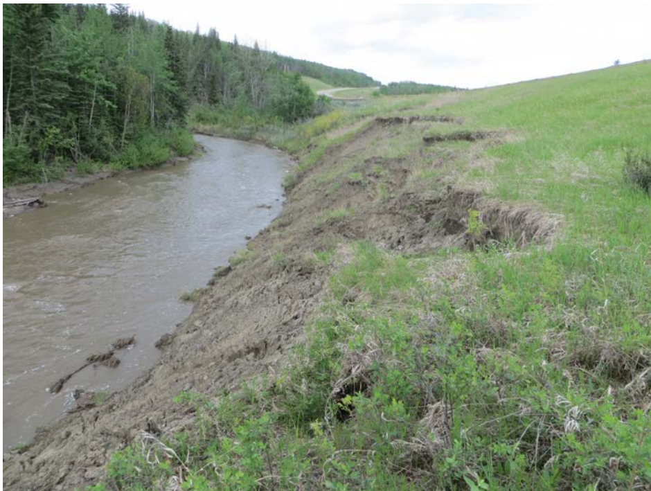
Photo 2 – Looking west at slumping above the creek at Site 1 in the south highway embankment.
