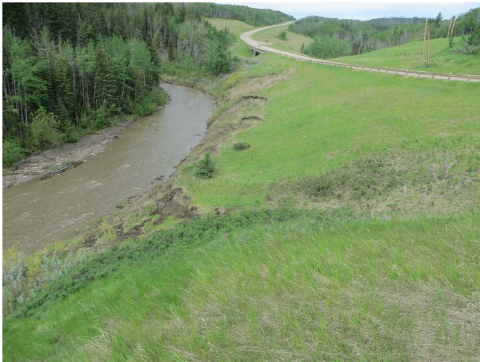
Photo 4 - Looking west along the Creek at the erosion at Site 1.
