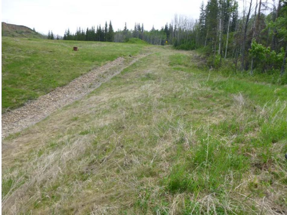
Photo 11 – Looking northeast along the ditch channel of the upper south embankment of Site 2.
