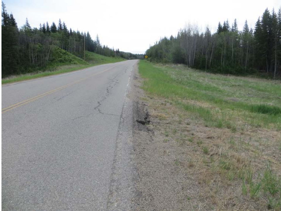
Photo 7 – Looking east along the highway at the cracks and dip overtop the culvert crossing at Site 2.
