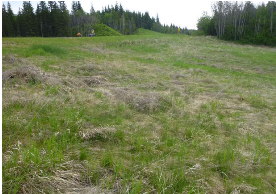
Photo 8 – Looking east at the slide scarp adjacent to the highway in the upper south embankment of Site 2.
