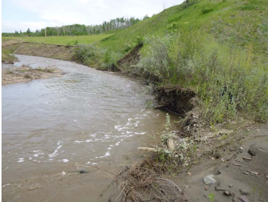
Photo 13 – Looking northwest at the erosion along the north edge of Hines Creek by the culvert outlet area of the south embankment of Site 2.
