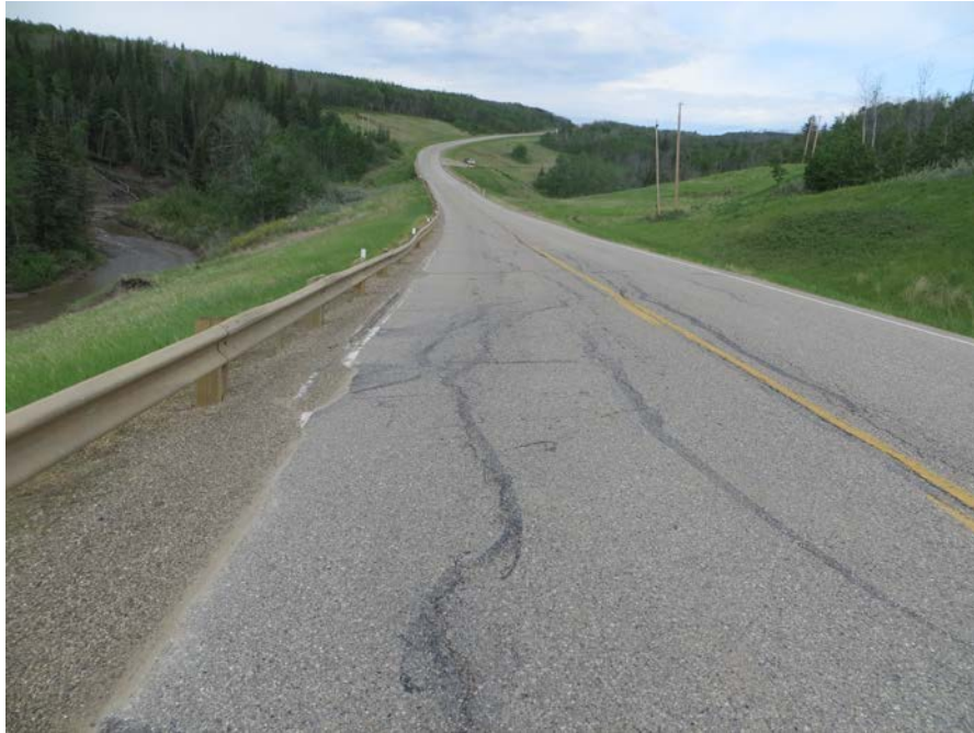
Photo 5 – Looking west along the highway at the crack/dip in the highway above the Slide at Site 1.
