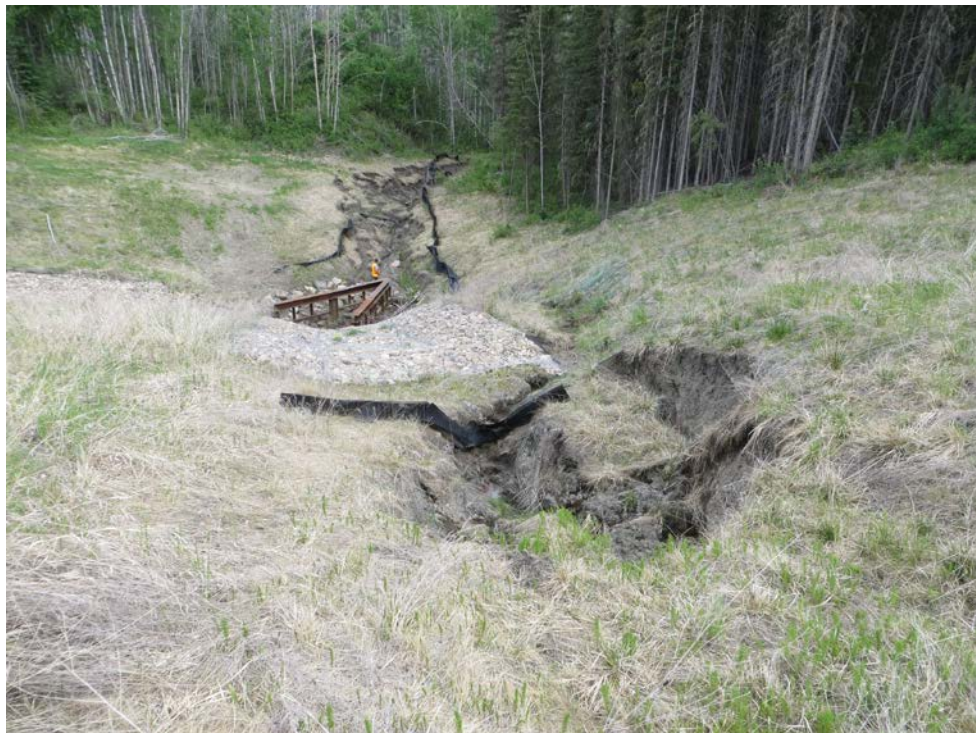
Photo 16 - Looking north at the eroded northeast TRM ditch above the culvert inlet area north of the highway at Site 2. Note the severe channel erosion leading into the culvert inlet.
