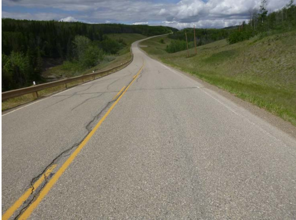
Photo 5 – Looking west along the highway at the crack/dip in the highway above Slide 1.
