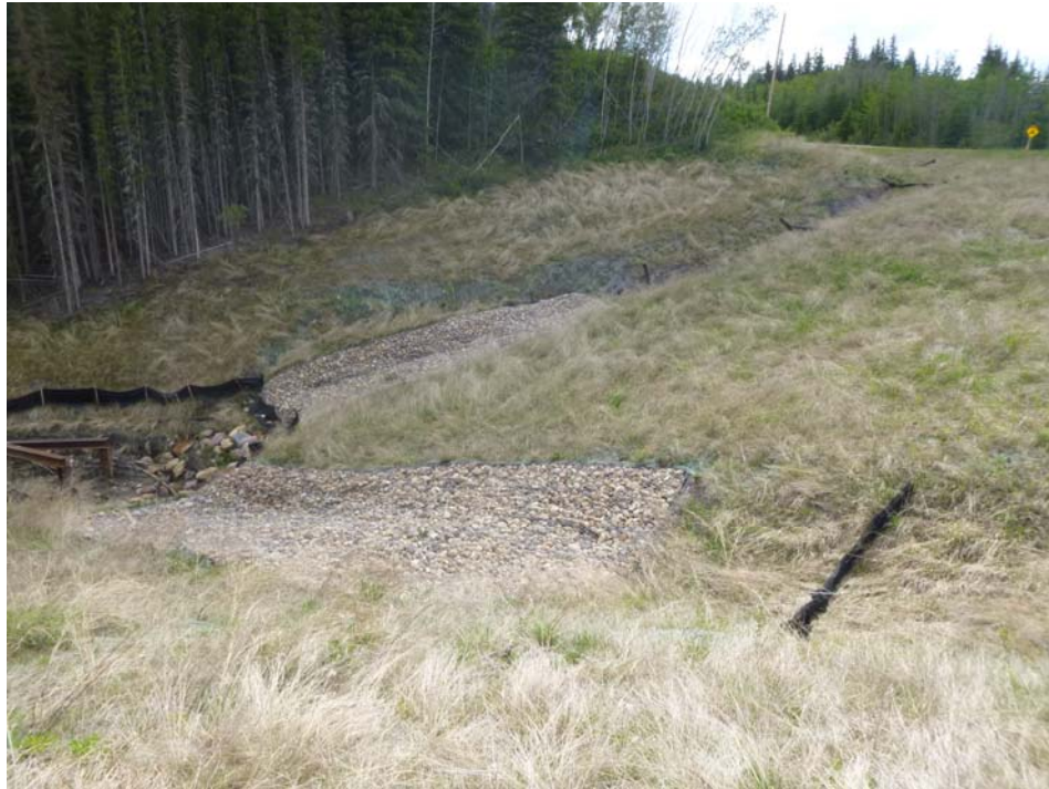
Photo 13 – Looking east across the culvert inlet area of the north embankment of Site 2.
