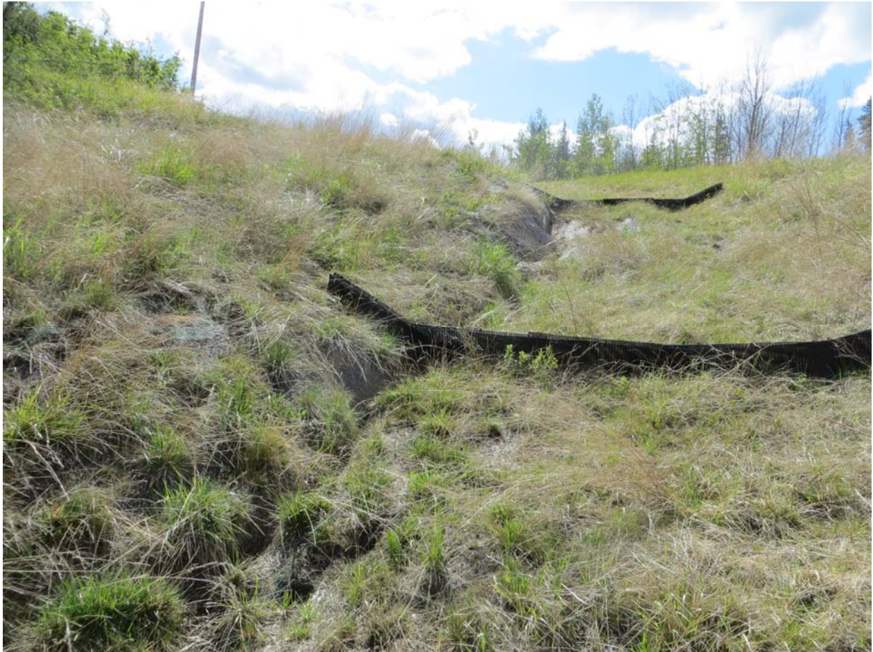
Photo 17 - Looking up at the eroded northeast TRM ditch of Site 2.
