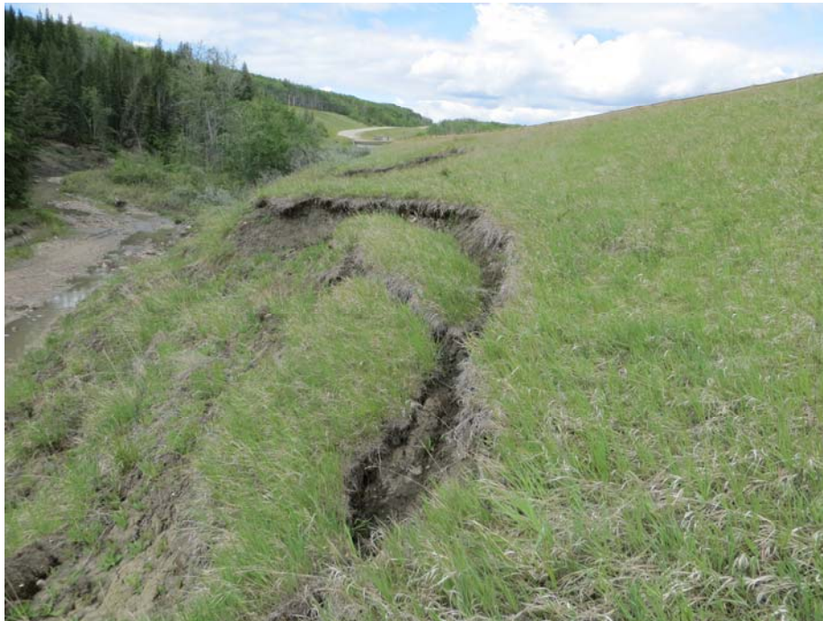
Photo 2 – Looking west at slumping above the creek at Site 1 in the south highway embankment.
