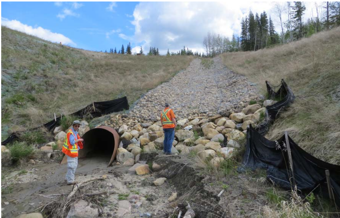
Photo 12 - Looking northeast at the culvert outlet area and south embankment of Site 2.
