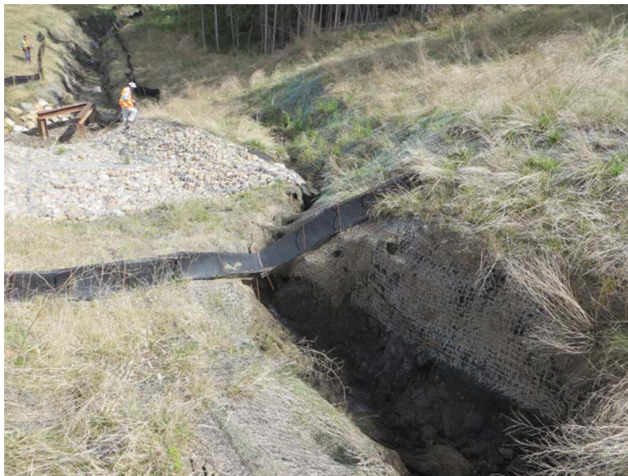
Photo 16 - Looking north at the eroded northeast TRM ditch above the culvert inlet area north of the highway at Site 2. Note the severe ditch erosion up-gradient of the gabions.
