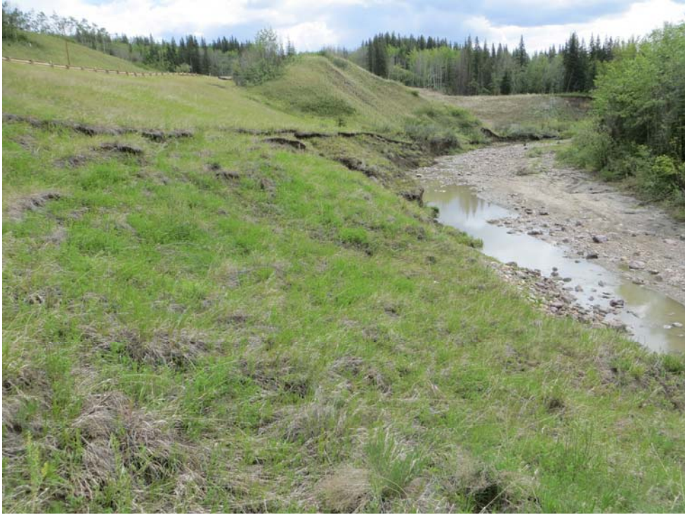
Photo 1 – Looking east at Slide site 1 along the north side of the Creek.
