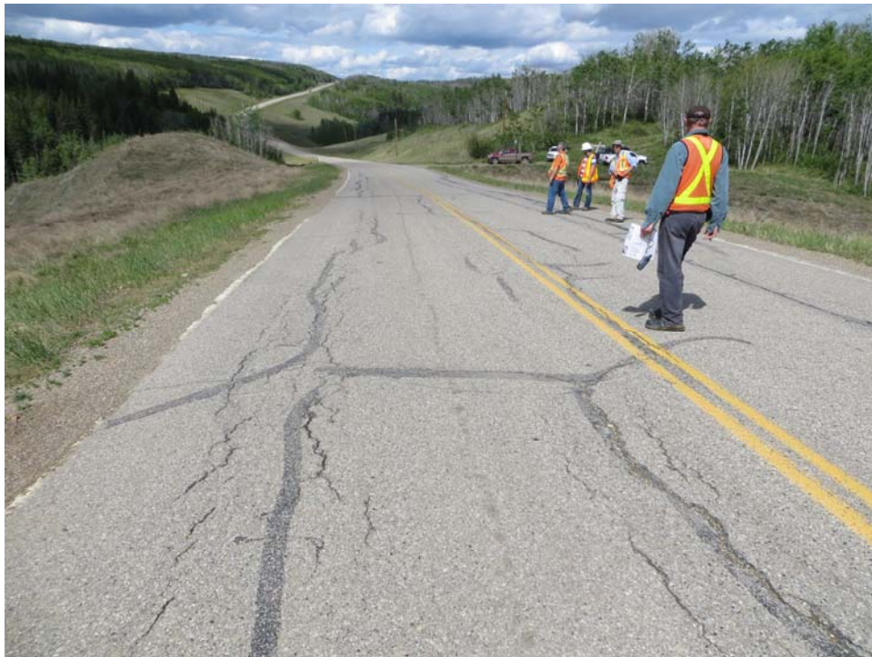
Photo 6 - Looking west along the highway and south embankment of Site 2. Note the settlement in both the highway and the embankment.
