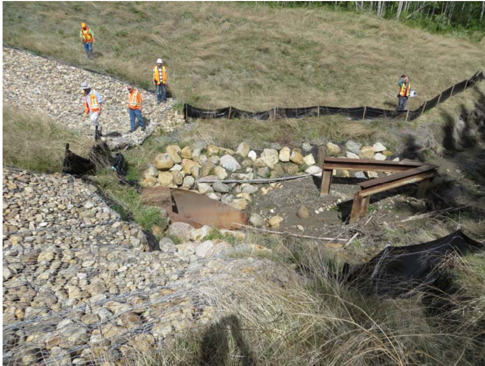
Photo 15 – Looking west across the culvert inlet area of the north embankment of Site 2. Note the undermining of the end of the gabions east of the culvert inlet.
