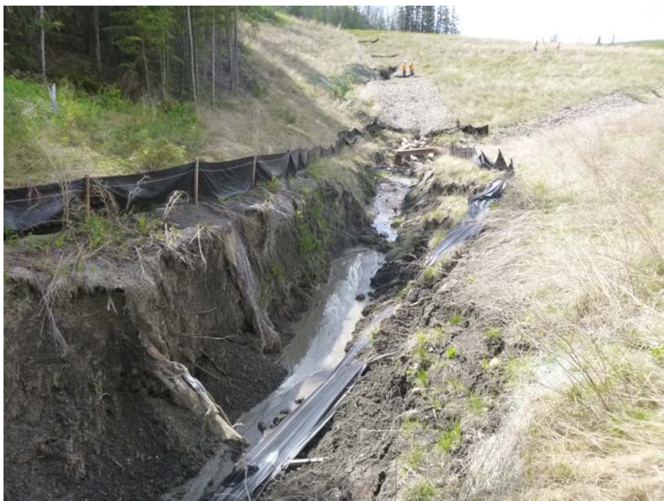
Photo 14 - Looking south from upstream of the culvert inlet area at the severe channel erosion north of the highway at Site 2.
