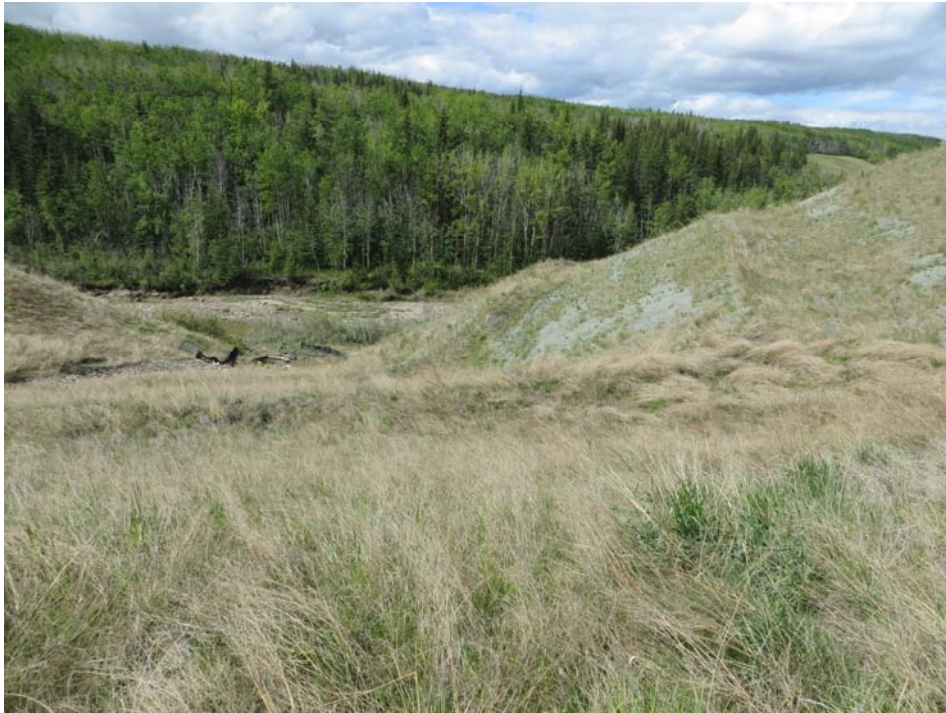
Photo 9 – Looking west along the south embankment of Site 2. Note the benched hillside and the subsidence near to the highway over the culvert.
