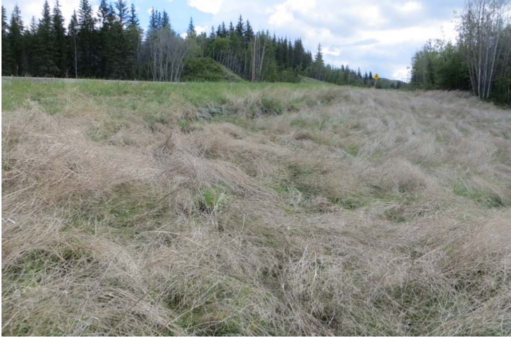
Photo 7 – Looking east at the slide scarp adjacent to the highway in the south embankment of Site 2.
