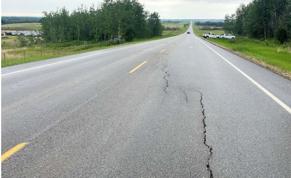
Photo 3: Looking west at cracks propagating west of the main scarp crack where previous hairline cracks were observed.
