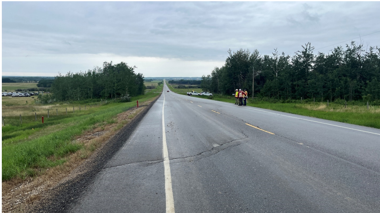
Photo 4: Looking west at the main scarp crack where it crosses the EBL.
