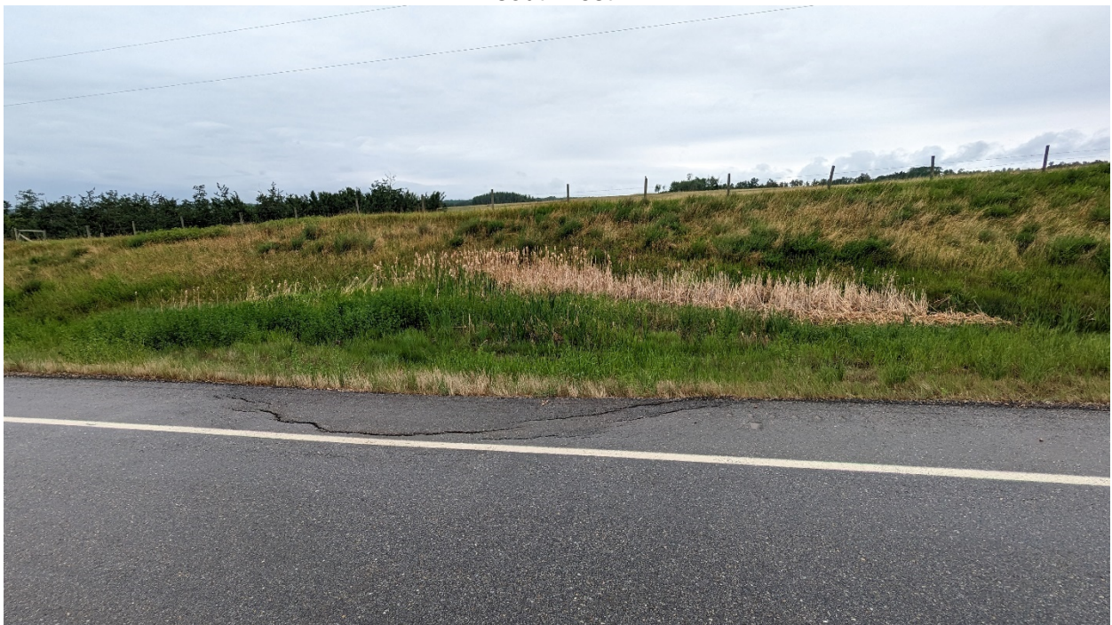
Photo 6: Looking northeast at a spring slumping observed in backslope to the east of the site. Cattails and ponded water are present in the ditch and cracking is developing on the shoulder.
