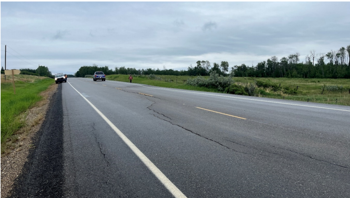
Photo 2 – Looking east at the west end of the arc-shaped crack. A crack is also forming on the shoulder of the WBL.
