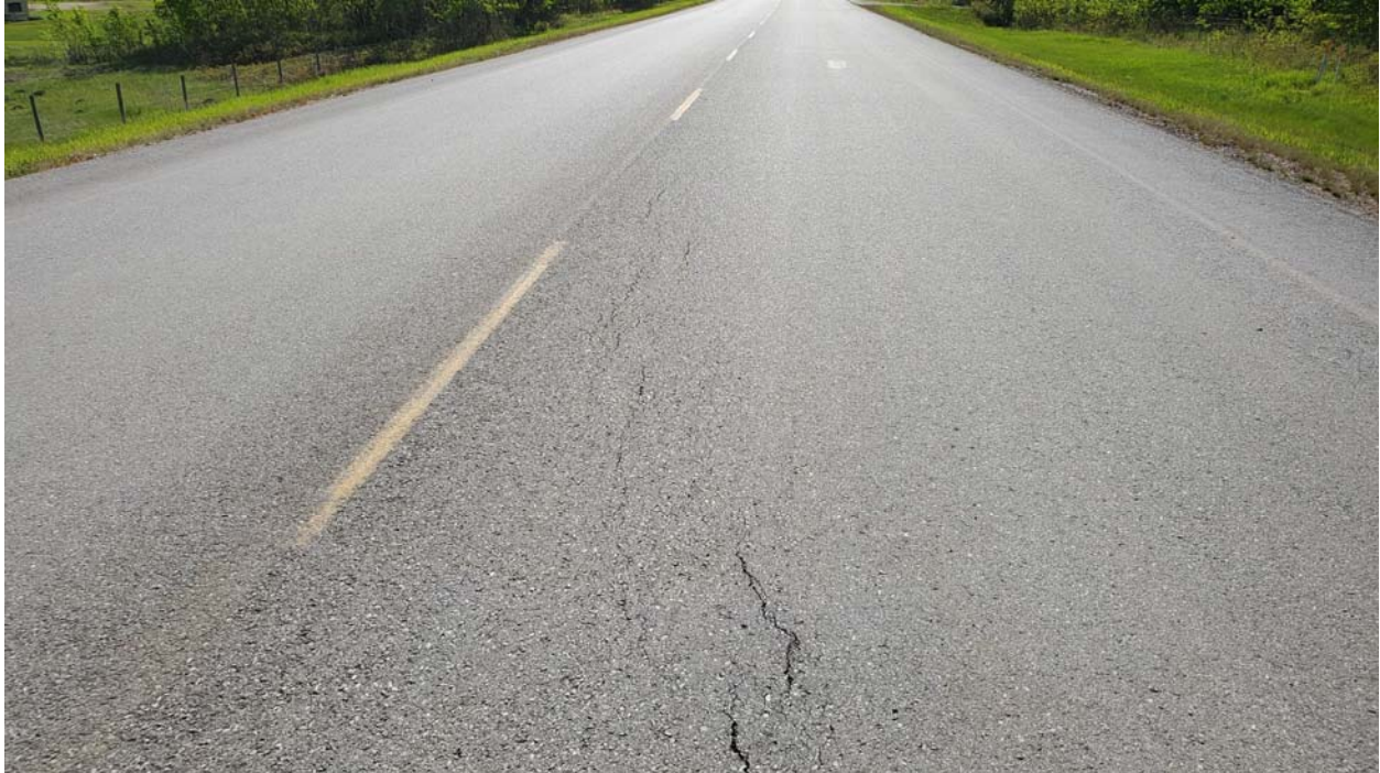
Photo 3 – Looking west at hairline cracks forming west of the main scarp crack.
