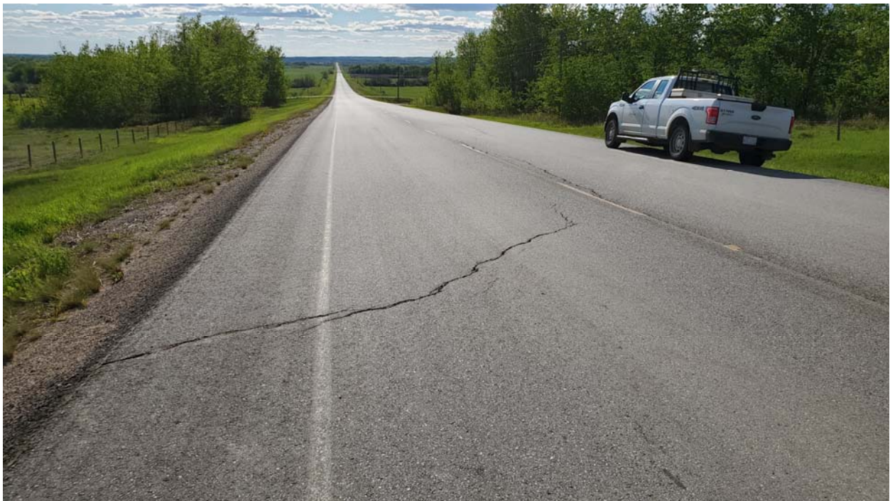
Photo 4 – Looking west at the main scarp crack where it crosses the EBL.
