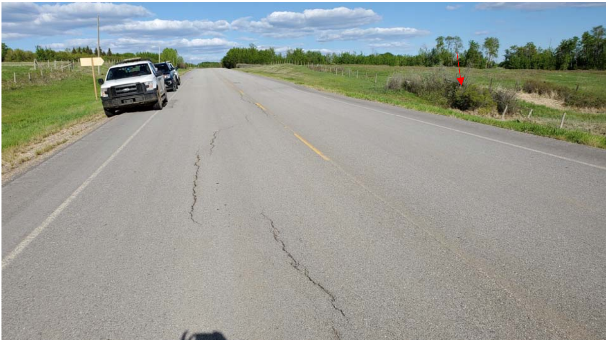
Photo 2 – Looking east at the west end of the arc-shaped crack. The second well is located in the bush on the south side of the highway (red arrow).
