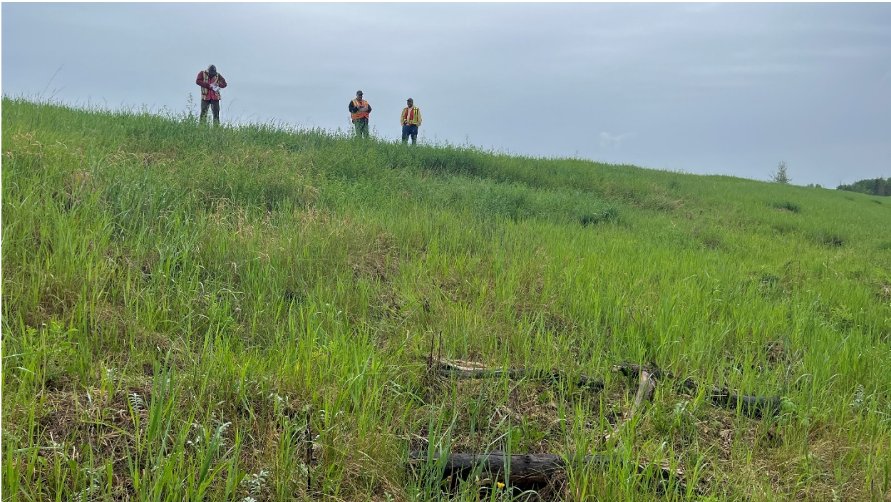
Photo 8 – Looking north up at the slide from the toe of the highway embankment.
