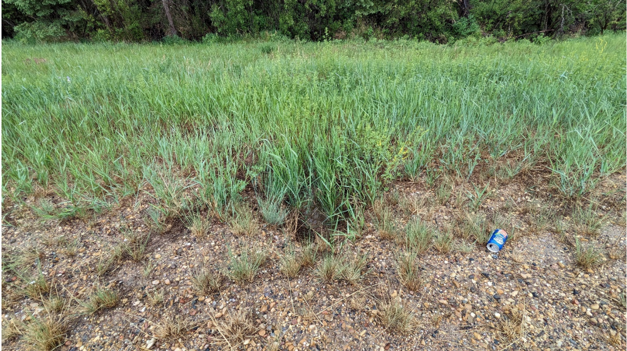
Photo 3 – Looking south at small sinkhole that has started to form on the embankment side slope.
