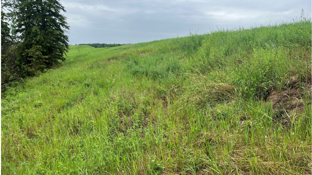
Photo 5 – Looking west at the slide scarp in the highway south embankment.
