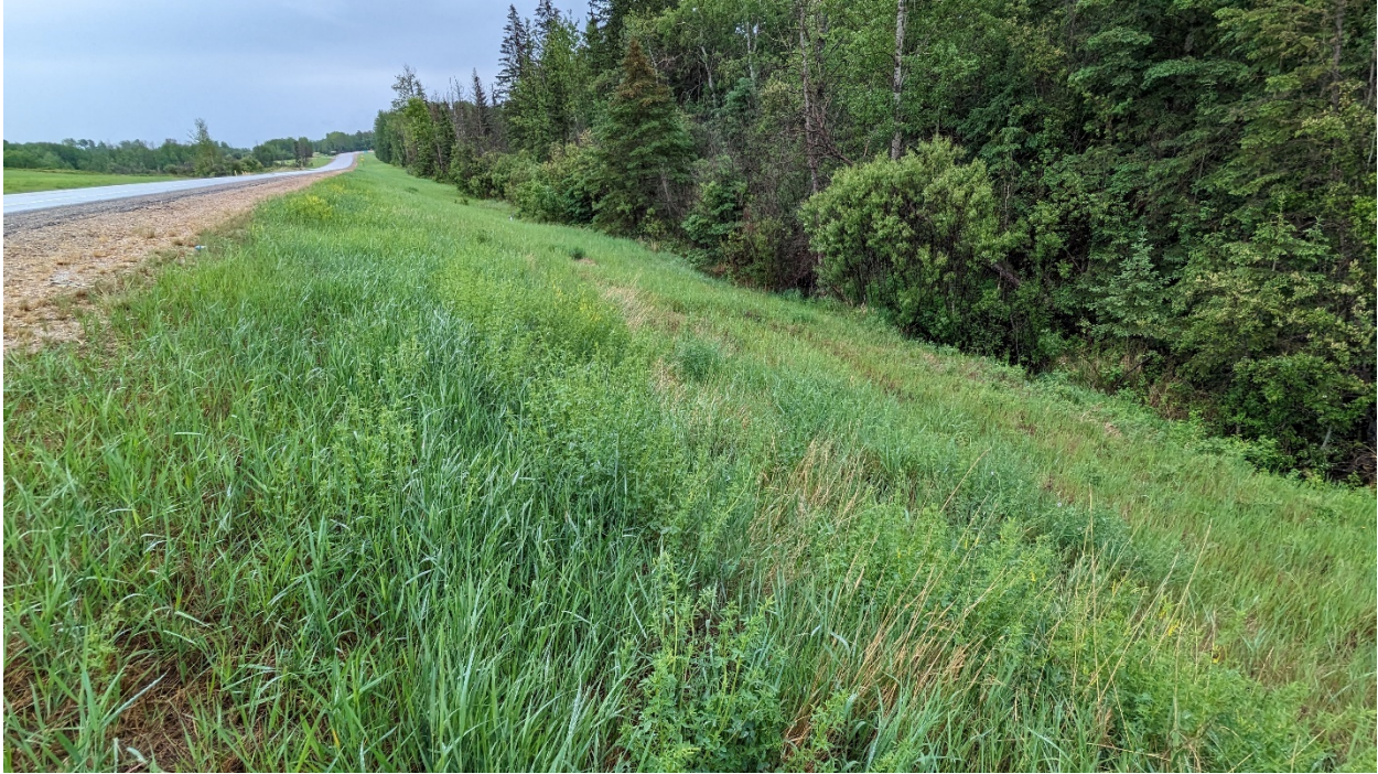
Photo 7 – Looking southeast across the slide. The dense forest extends over the stream and right up to the toe of the south highway embankment.
