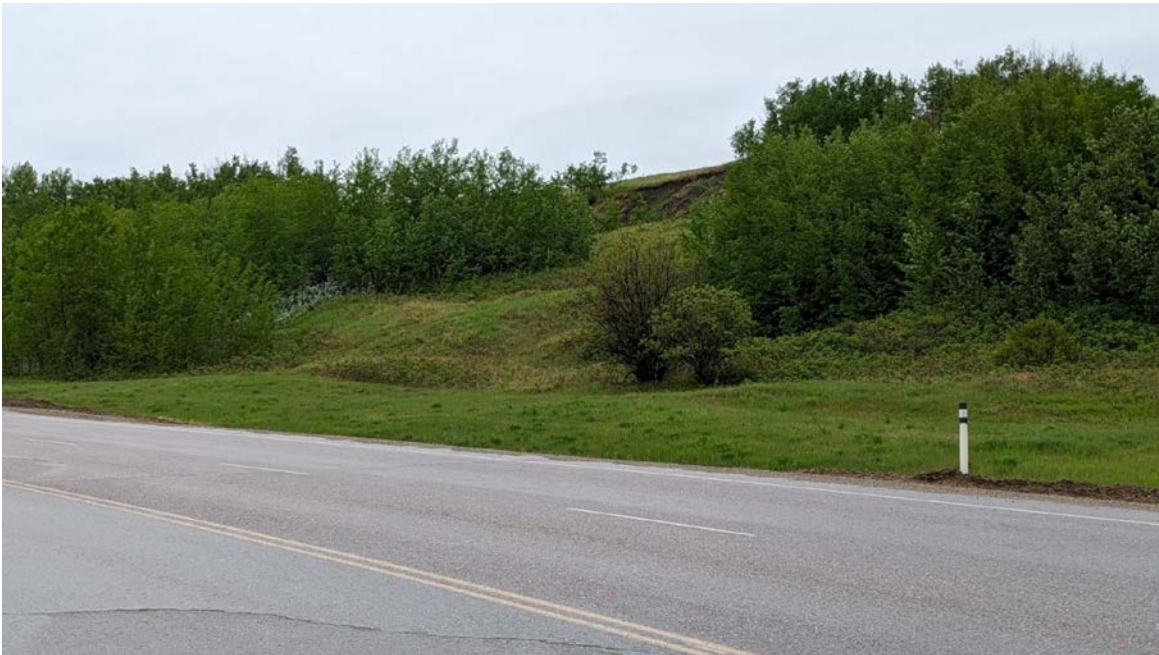
Photo 2 – Looking at the southwest slide movement in the backslope above the highway.
