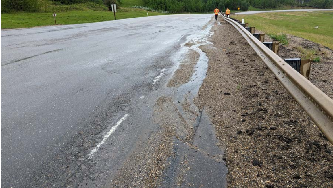
Photo 5 – Looking north at the first set of scarp cracks at south end of the site.
