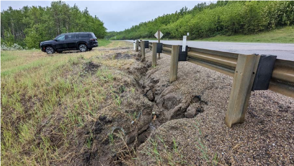
Photo 3 – Looking south at an erosion gully that has formed at the south end of the guardrail.
