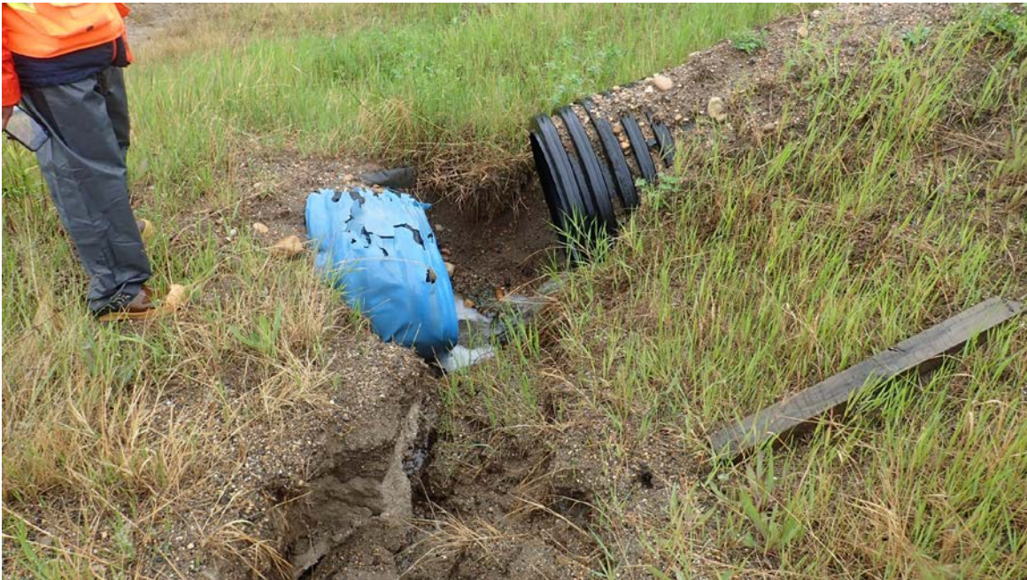
Photo 4 – Looking at 760 mm culvert joint separation. The gully in the foreground is the one shown in Photo 3.
