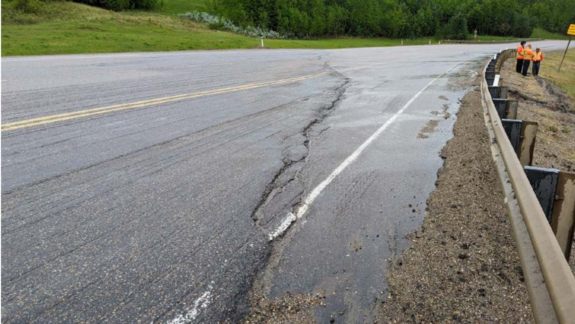
Photo 7 – The third set of scarp cracks further north of the second set and near the north end of the east guardrail.
