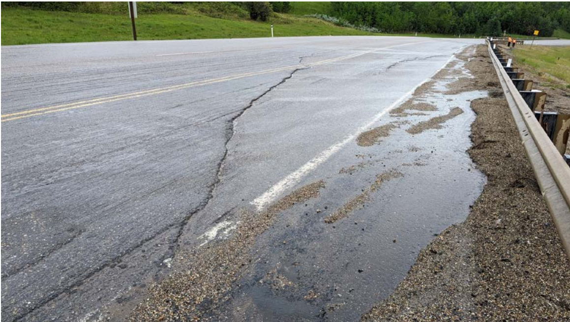
Photo 6 – The second set of scarp cracks just north of Photo 5.
