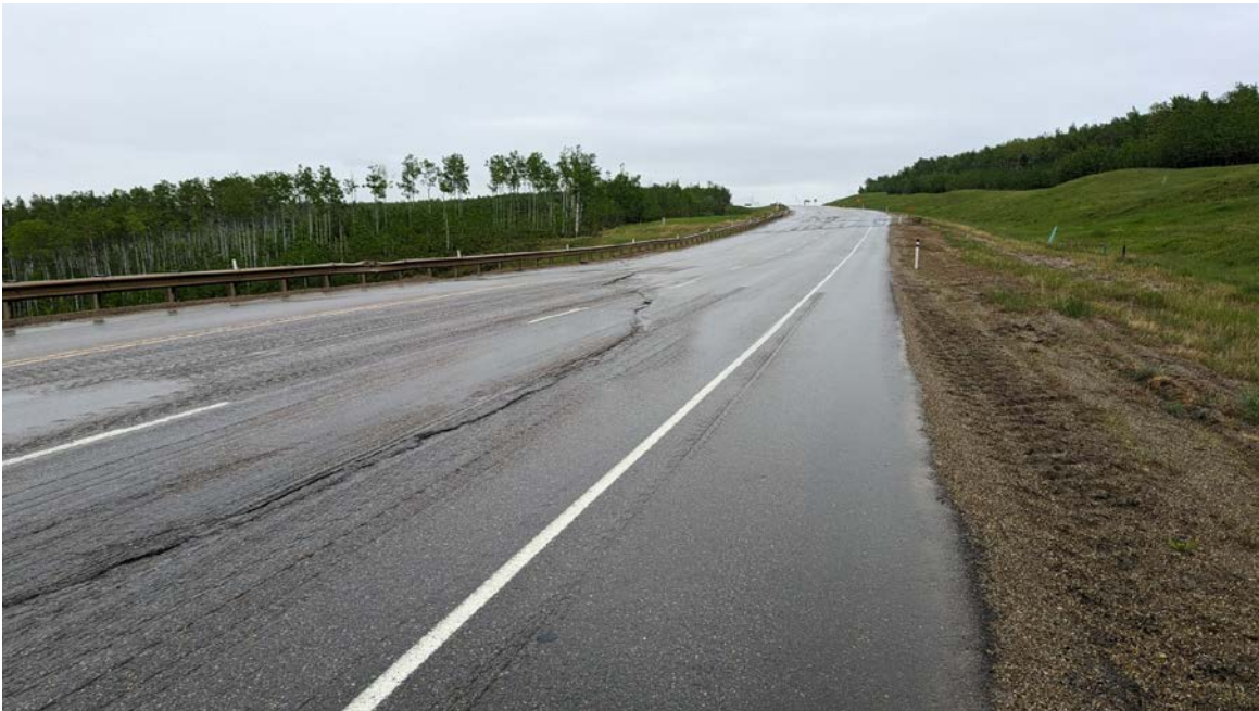
Photo 8 – Looking northeast at the cracks of the east side of main scarp block at Sta. 0+770.
