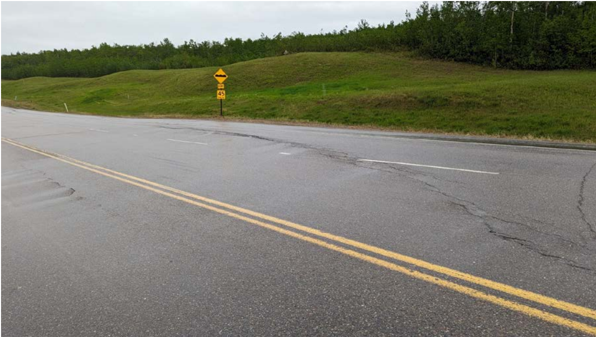
Photo 7 – Looking southeast at the cracks on the west side of main scarp block at Sta. 0+770.
