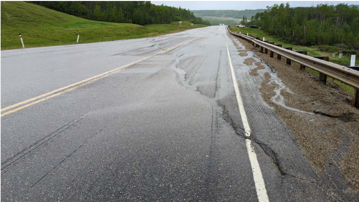
Photo 6 – Looking west at main scarp cracks at Sta. 0+680.
