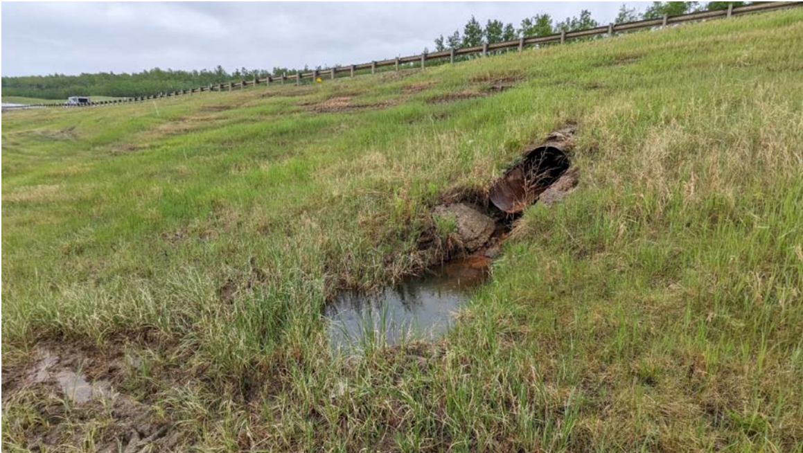
Photo 9 – Developing erosion bowl at outlet of the 750 mm-dia. culvert at about Sta. 0+810.
