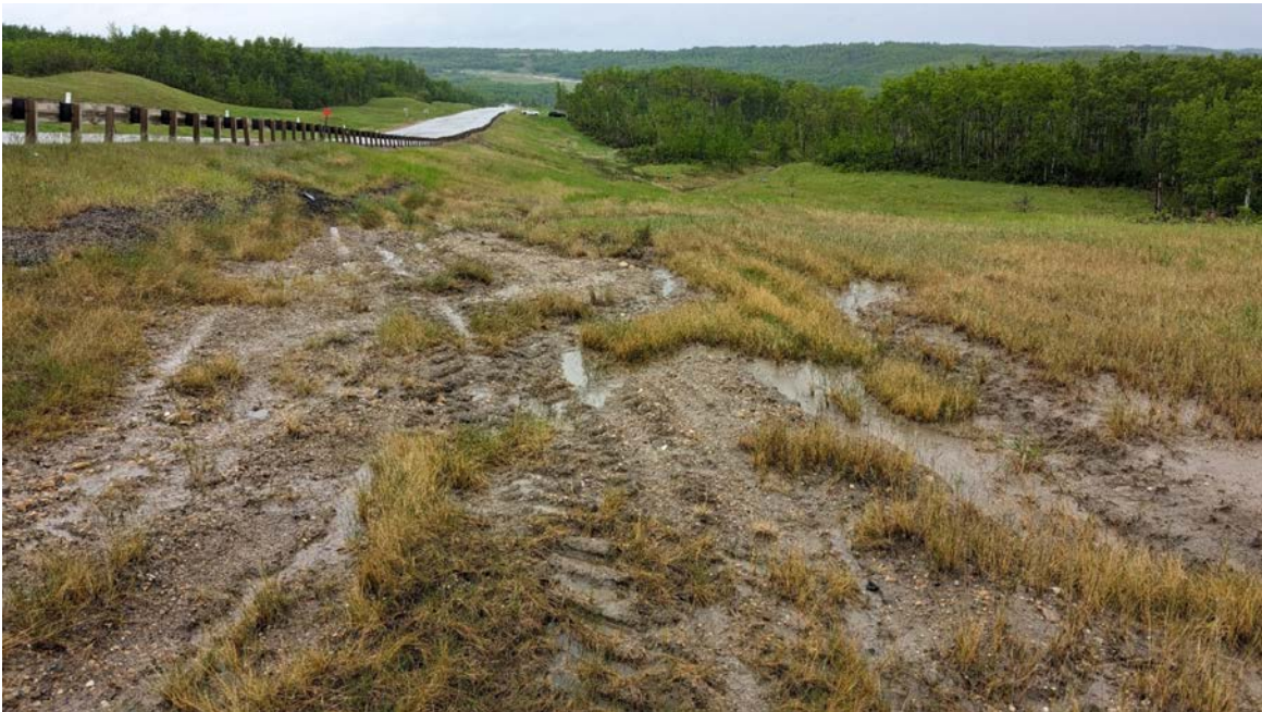
Photo 2 – Looking southwest along erosion gully near Sta. 0+550.
