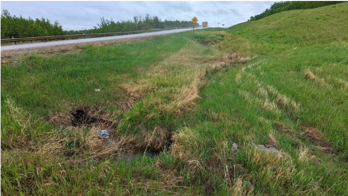
Photo 10 – Erosion at the culvert inlet (left side) and scour bowl (right side) at Sta. 0+430 is starting to encroach towards the highway.
