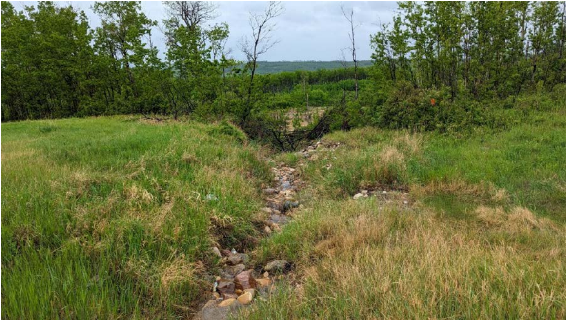
Photo 1 – Erosion gully at outlet of culvert at about Sta. 0+450.
