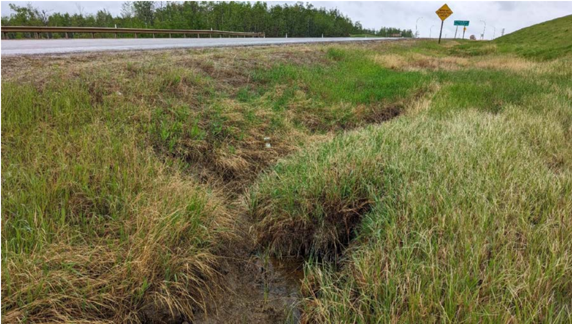
Photo 11 – Scour bowl forming close to the edge of the highway at Sta 0+430.
