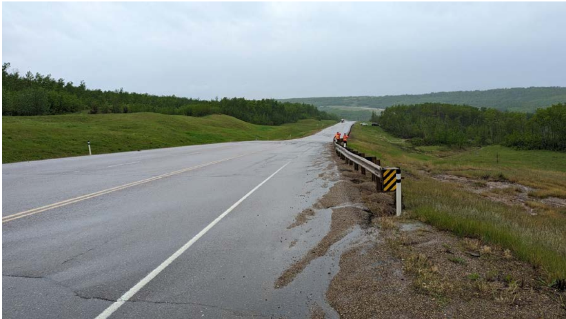
Photo 4 – Looking southwest over the main sag (graben) area extending from Sta. 0+600 to Sta. 0+800.
