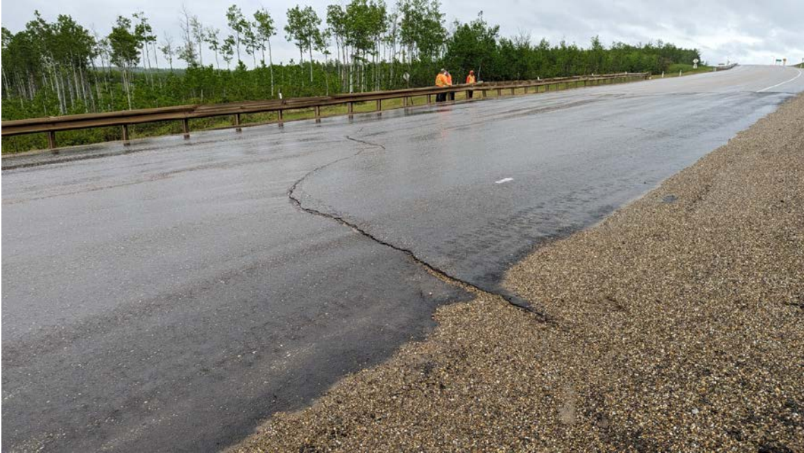
Photo 5 – Looking north at area of frequent patching in the main graben block movement at Sta. 0+600.
