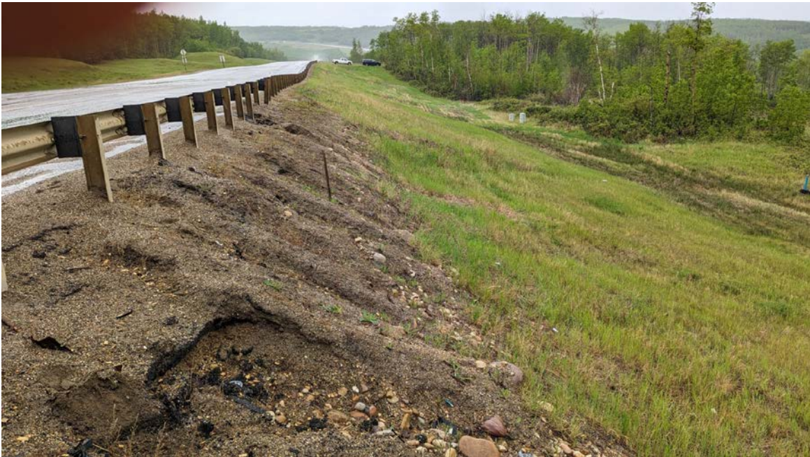
Photo 12 – Erosion rills by the guardrail and ravelling of the north side slope backscarp between Sta. 0+650 and 0+700.
