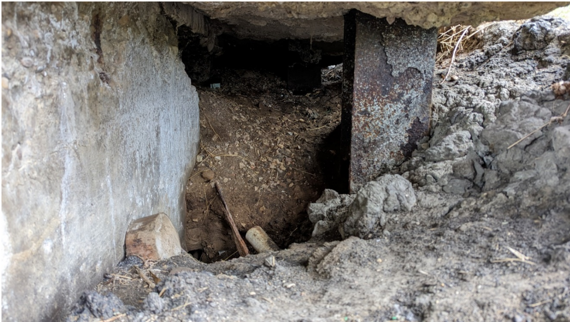
Photo 4: Void forming underneath the northeast corner of the old Abutment 1.
