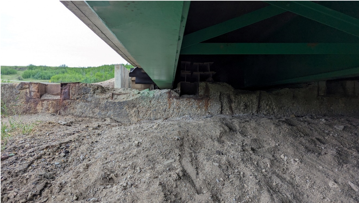
Photo 3 – Looking towards the West Abutment where portions of the old foundation concrete was removed to allow movement of the girders between the West Abutment and Abutment 1.
