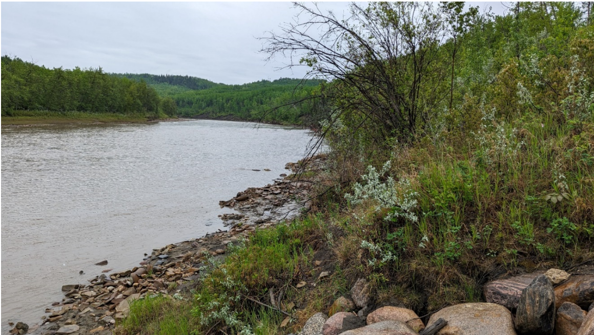
Photo 12 – Looking south at erosion along toe of riprap and riverbank.
