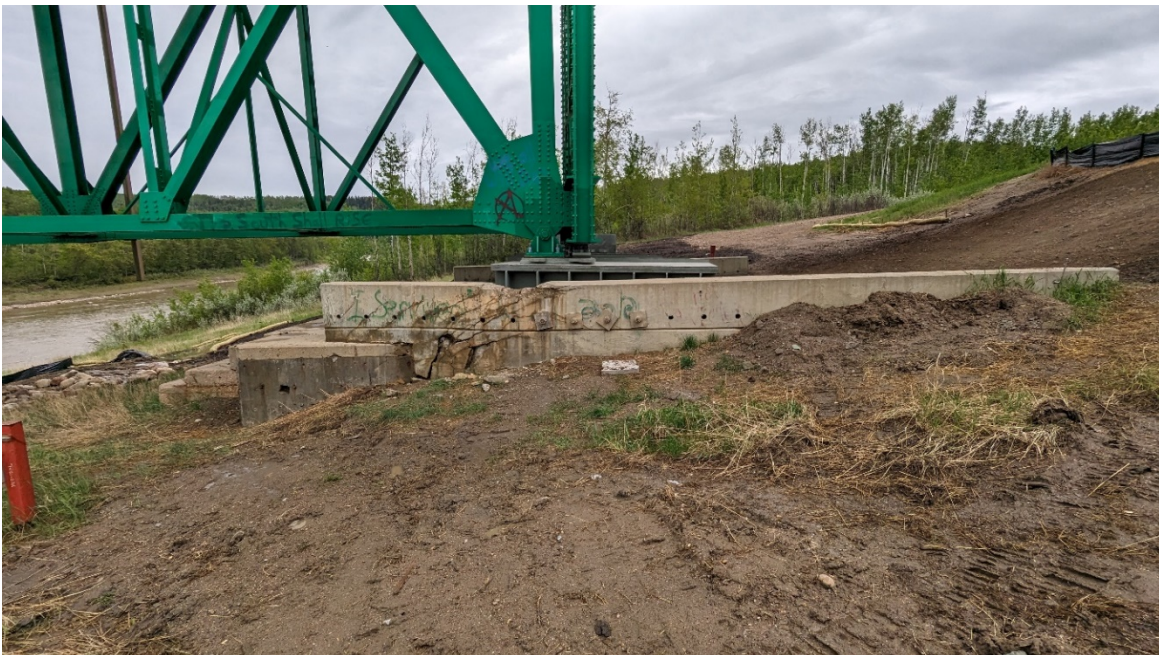
Photo 8 – Looking south at Pier 1 wingwall at arc-shaped compression crack pattern in foundation. Left-hand portion of foundation is pile supported; right-hand is on-grade.
