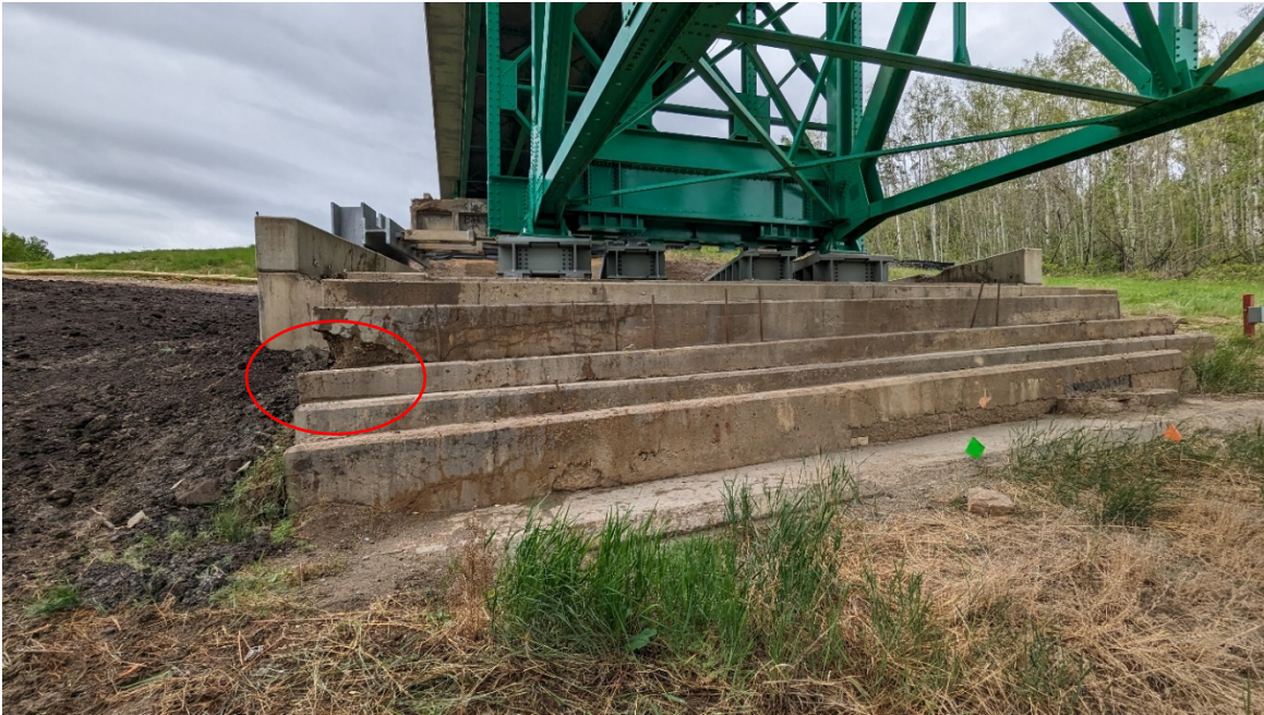
Photo 9 – Looking west at Pier 1 foundation which is tilted downward to the south. The angle from horizontal was 4° at the top and 7° at the bottom stage. Concrete is starting to crack and spall in circled area.
