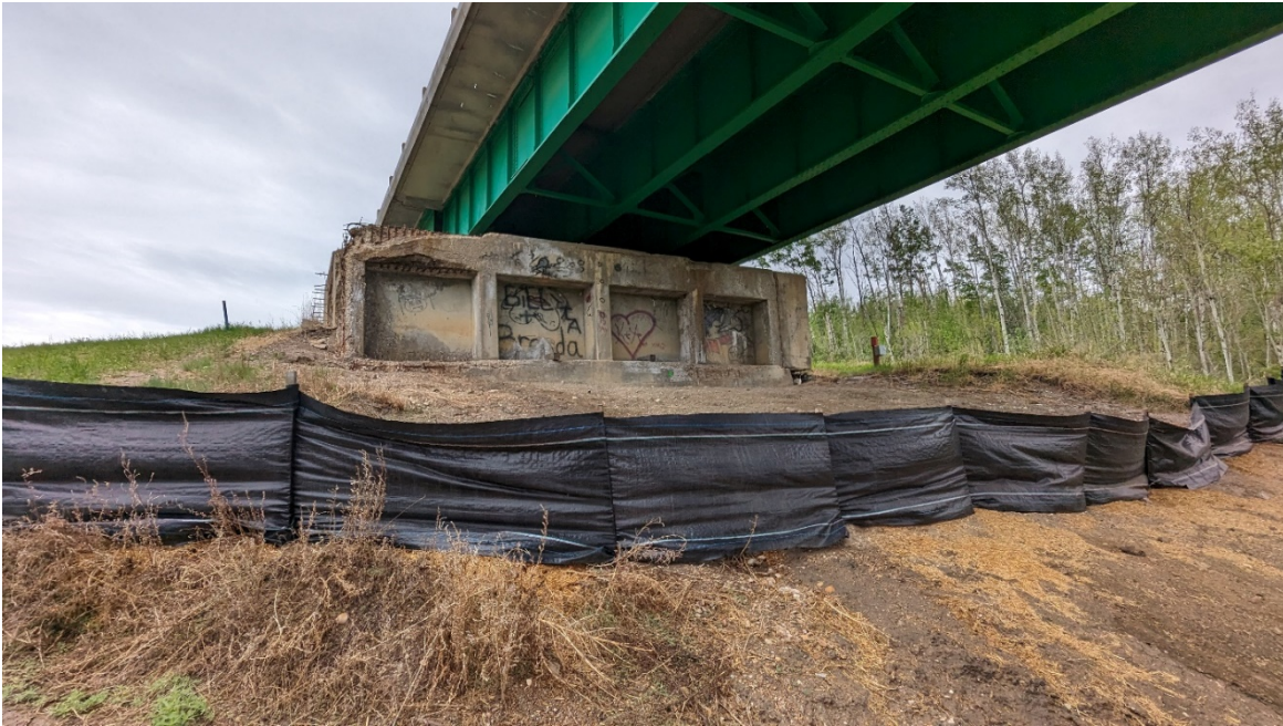
Photo 5: Looking west at headslope below Abutment 1. New erosion control measures installed since 2023.
