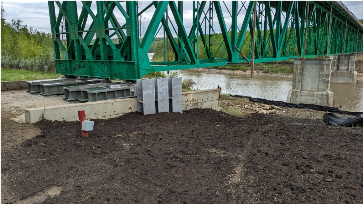
Photo 7 – Looking north at Pier 1 where new sliding plates and lateral restraints were installed since 2023 as well as regrading and topsoil around the pier.
