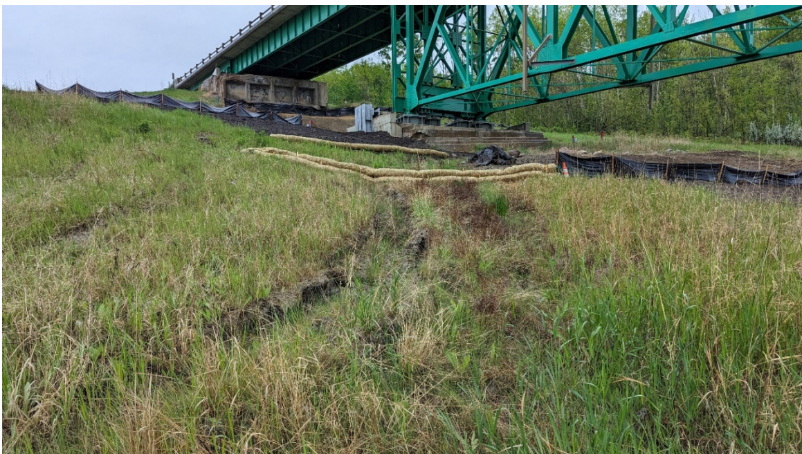
Photo 10 – Looking west toward Pier 1 at rutting and recently-installed erosion control measures.
