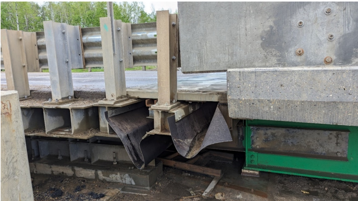
Photo 2 – Looking north at west bridge abutment. New I-beams added in 2023 (5 total) plus one below the finger joints. The tarps were added in 2024. Distance between angle iron and concrete of bridge deck was reset to 3.61 m prior to 2023 inspection and was 3.57 m in 2024 (previous gap shrunk to 2.42 m in 2022 from 2.82 m in 2017).
