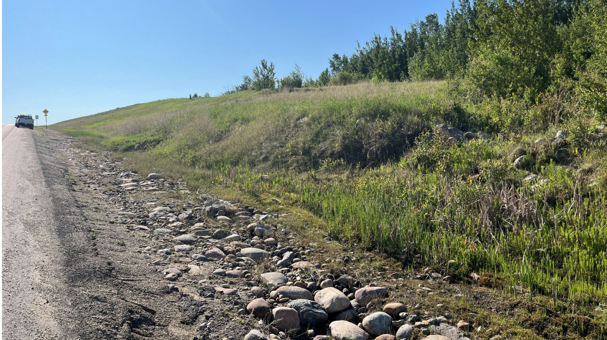
Photo 1 – Looking east at toes of Slumps B and A which were excavated in 2019 to improve ditch flow with the material placed back on top of the slumps.
