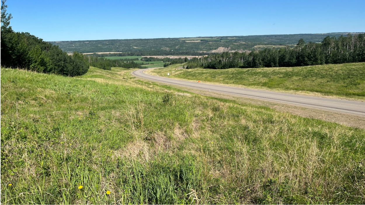
Photo 3 – Looking northwest at the crest of Slump D
