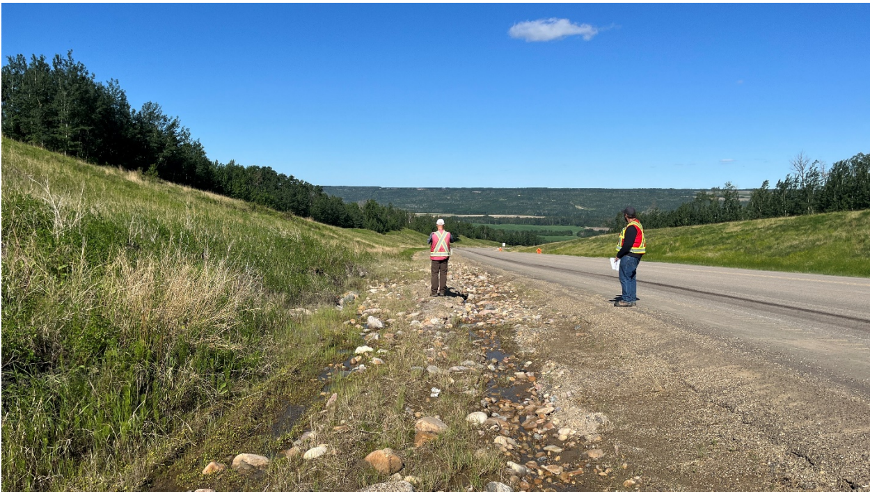
Photo 4 – Looking west at the toe of Slump B.
