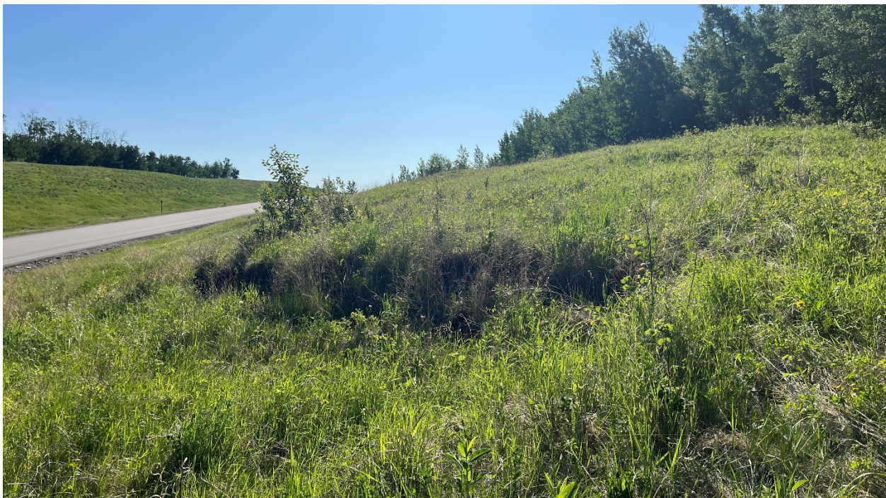
Photo 2 – Looking east at the top of Slump B. Vegetation has grown within the regraded area in 2019.
