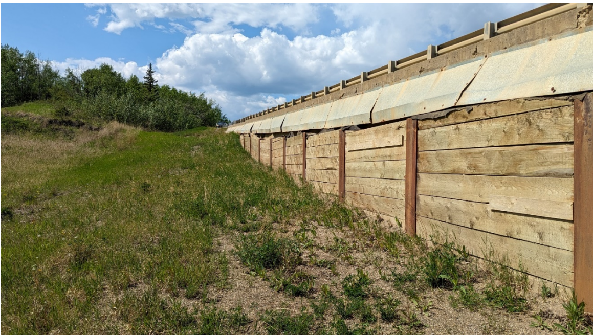
Photo 4 – Looking north at the displaced H-pile and timber lagging wall near the scarp at the north end of the wall.
