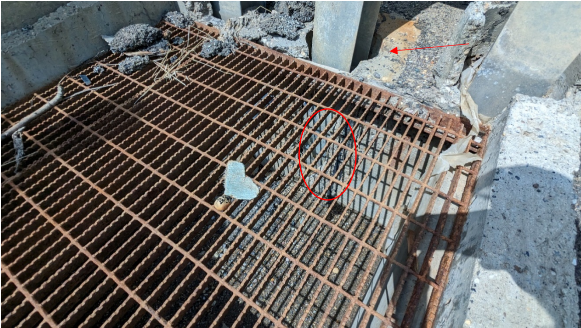
Photo 3 – The thin concrete on the side of the catchbasin (red circle) has crack and water from the surface (red arrow) is ponding in the void left during pouring of the basin.
