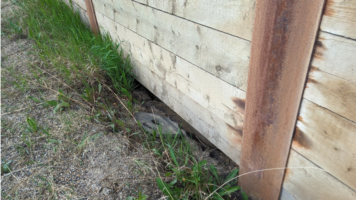
Photo 5 – Crack and void opening up below the timber lagging.
