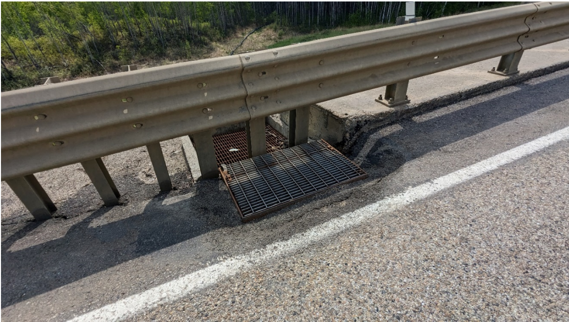
Photo 2 – Catch basin inlet at the south end of the wall leading to the elephant trunk downpipe.
