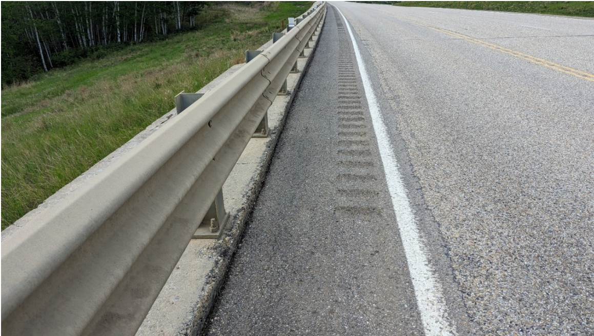
Photo 7 – Looking at the crack that is opening up again between the cap beam and asphalt.
