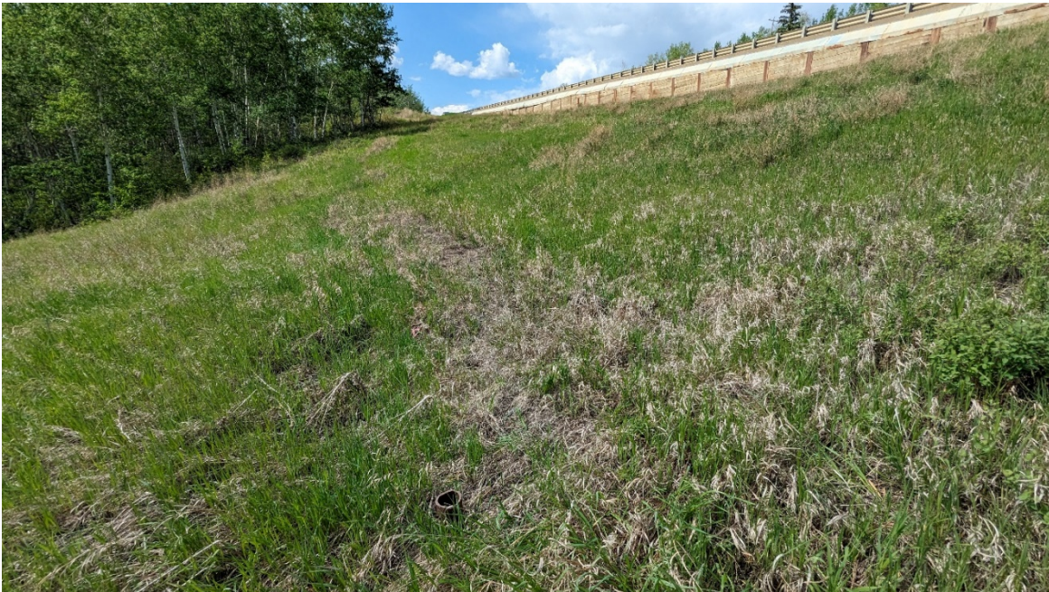
Photo 6 – Looking northwest at the gabion basket wall a newly-protruding screw pile.
