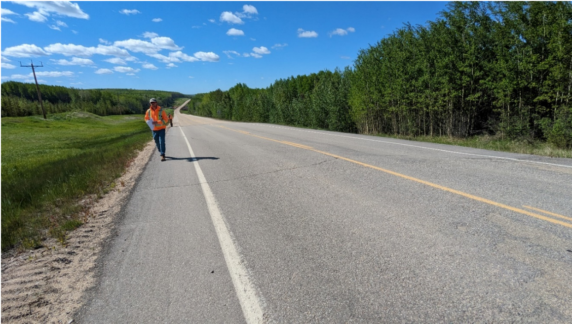
Photo 1 – Looking south from east shoulder at main scarp crack and patch at north end of site.
