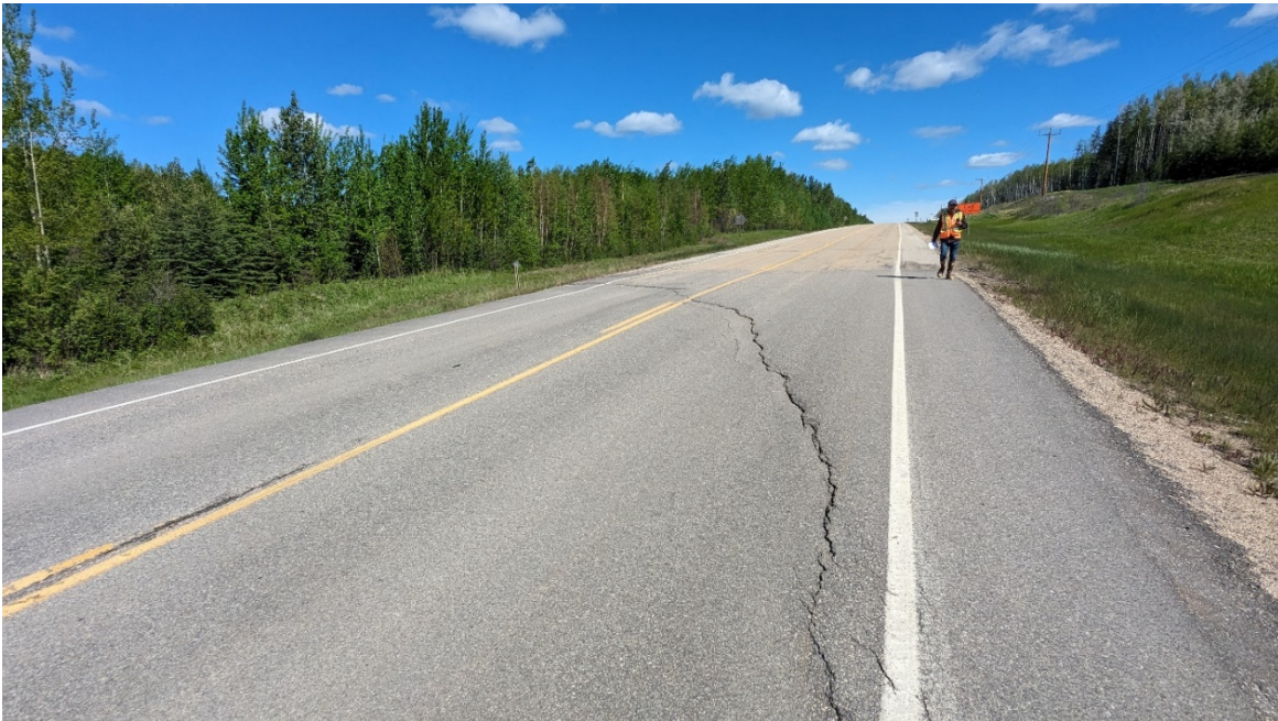
Photo 4: Looking south at crack at south end of patch at north end of the site.
