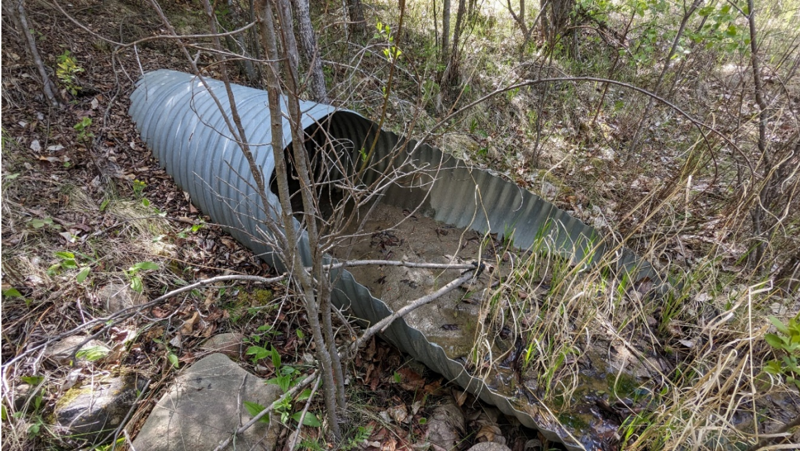
Photo 5: Looking at south culvert which had build up of sediment at outlet.
