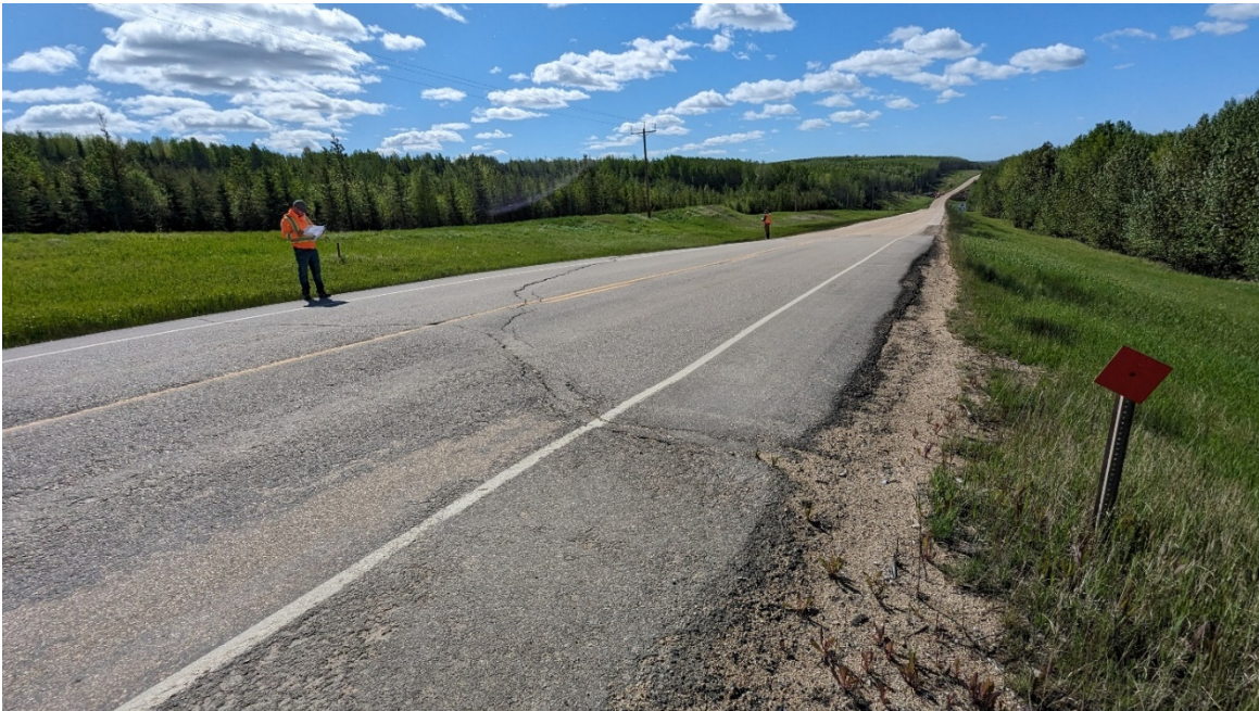
Photo 2 – Looking south from west shoulder at main scarp crack and patch at north end of site. Note powerline installed on east side of highway since 2017 visit.
