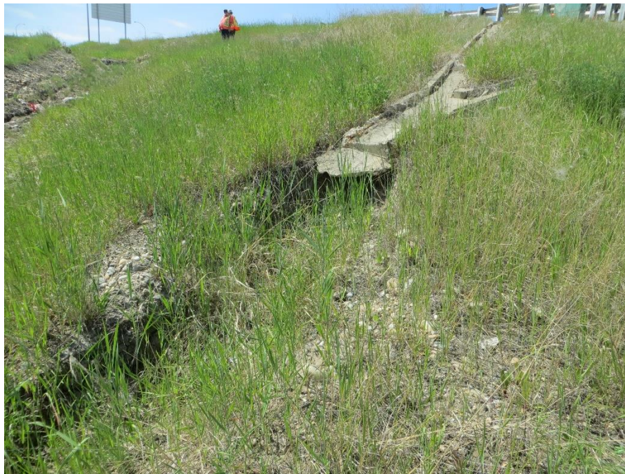
Photo 13. Looking northwest at the erosion occurring below the west abutment south sideslope concrete drainage swale.
