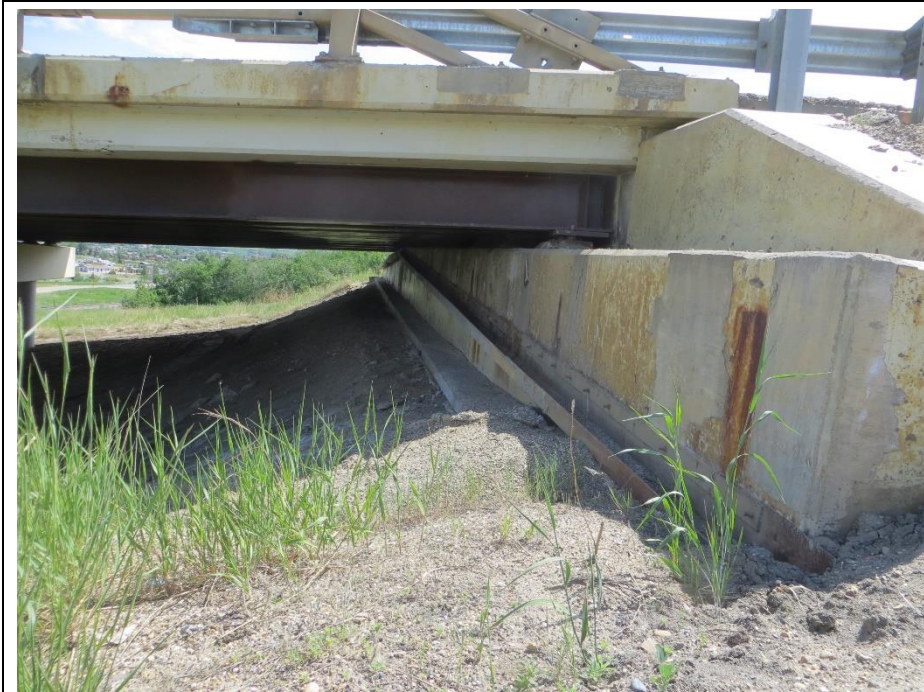
Photo 11. Looking southeast from the north side of the west bridge abutment seat.
