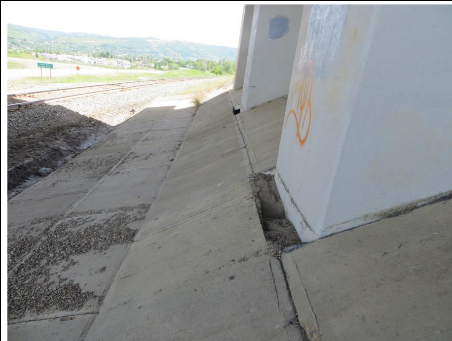
Photo 3. Looking southeast at the sliding of the concrete slope protection at the base of the west side headslope pier.
