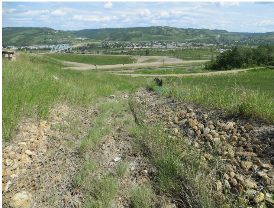
Photo 15. Looking northeast along the gabion mattresses at the interface of the west abutment sideslope and the slope (No significant change since 2016).
