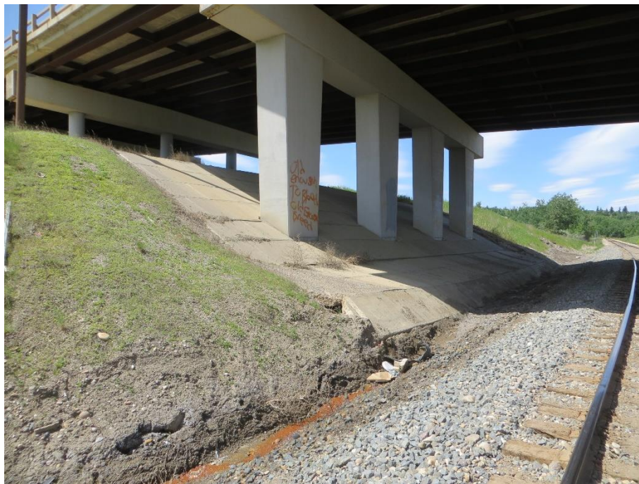
Photo 2. Looking northwest at the buckling of the concrete slope protection at the base of the west side headslope pier.
