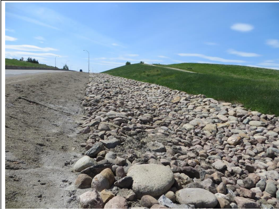
Photo 12. Looking southwest along the Hwy 2 WBL sideslope at the new rip rap placed in the ditch bottom in 2016.
