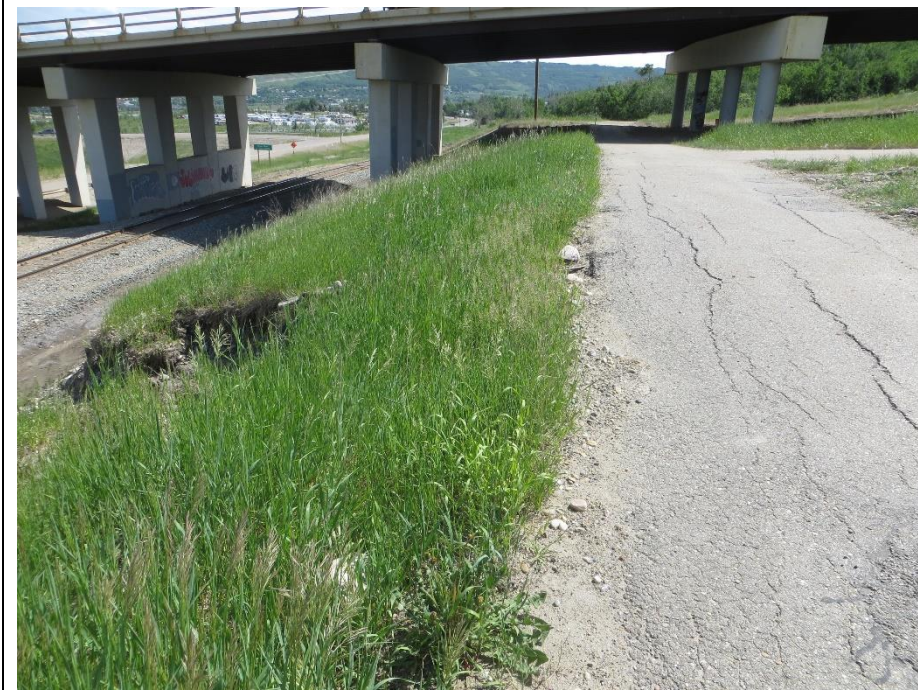
Photo 9. Looking southeast at the cracks forming in the ACP trail above the small backlope failure above the CNR railway line.
