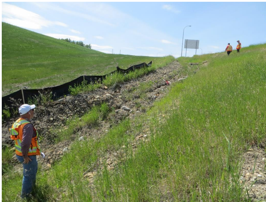
Photo 14. Looking southwest at the gabion mattresses along the interface of the west abutment sideslope and the slope (No significant change since 2016).
