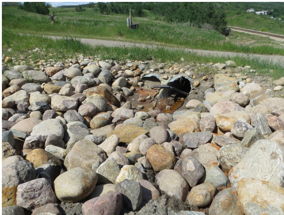
Photo 6. Looking northeast at the inlet to the double barrel culverts that run beneath the ACP pedestrian trail on the north side of the west abutment. Note the presence of oxides in the water at the culvert inlets.
