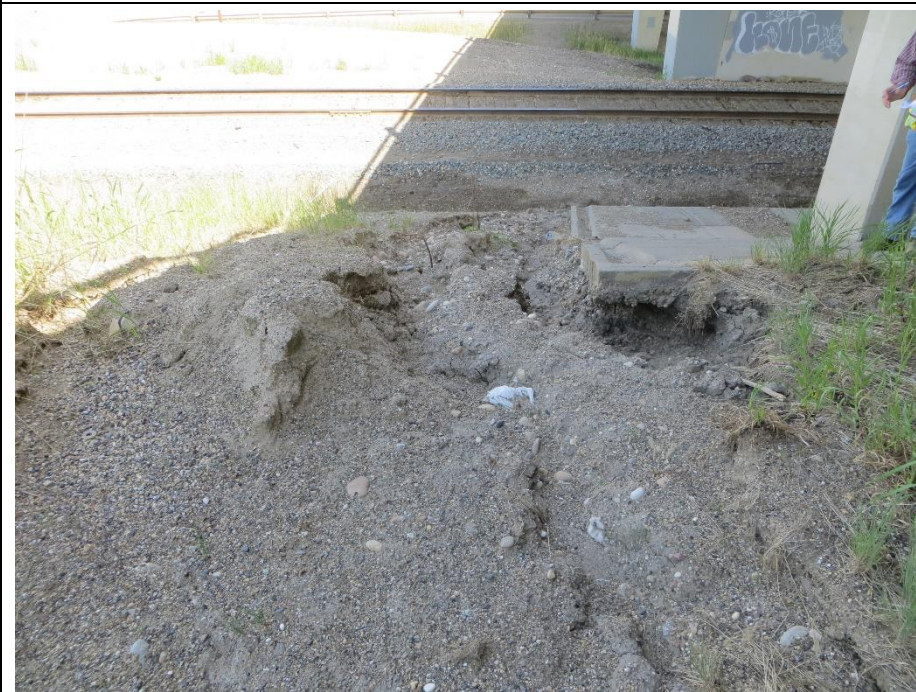
Photo 4. Looking northeast at the concrete headslope protection on the north side of the west abutment headslope that has been undermined by 270 mm.
