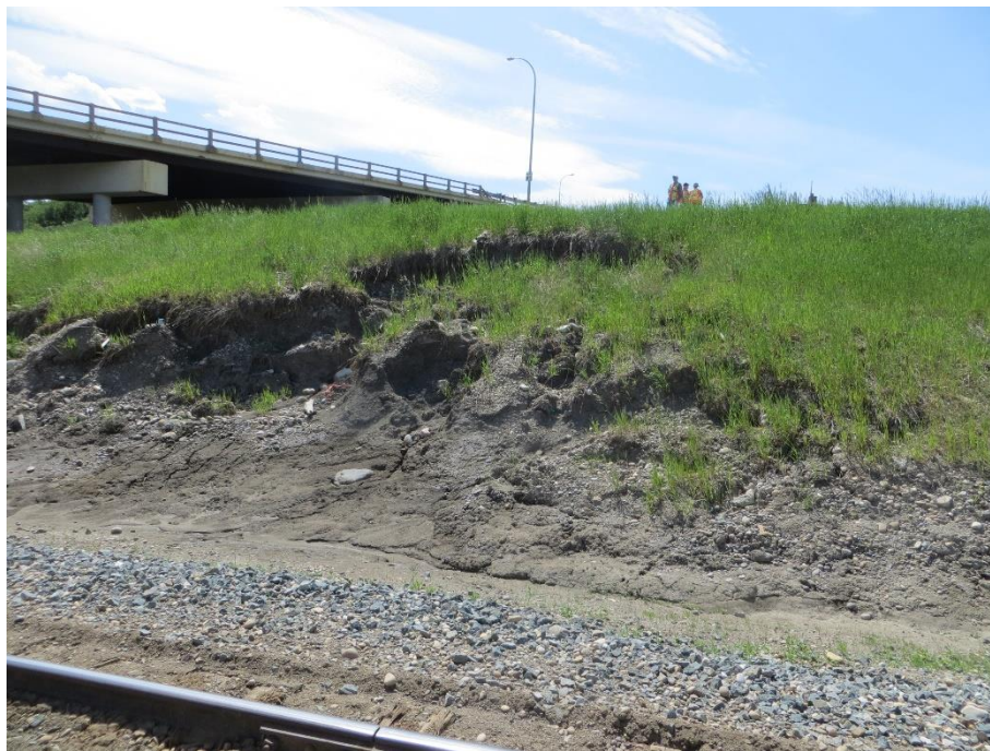
Photo 8. Looking southwest at the small backslope failure above the CNR railway line and ACP trail the runs beneath the west abutment.
