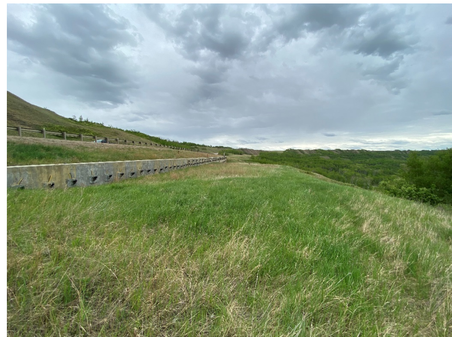
Photo 70-04. View east from the west end of the 2017 pile wall (34+000) on the downslope side. Similar appearance to the 2023 conditions.
