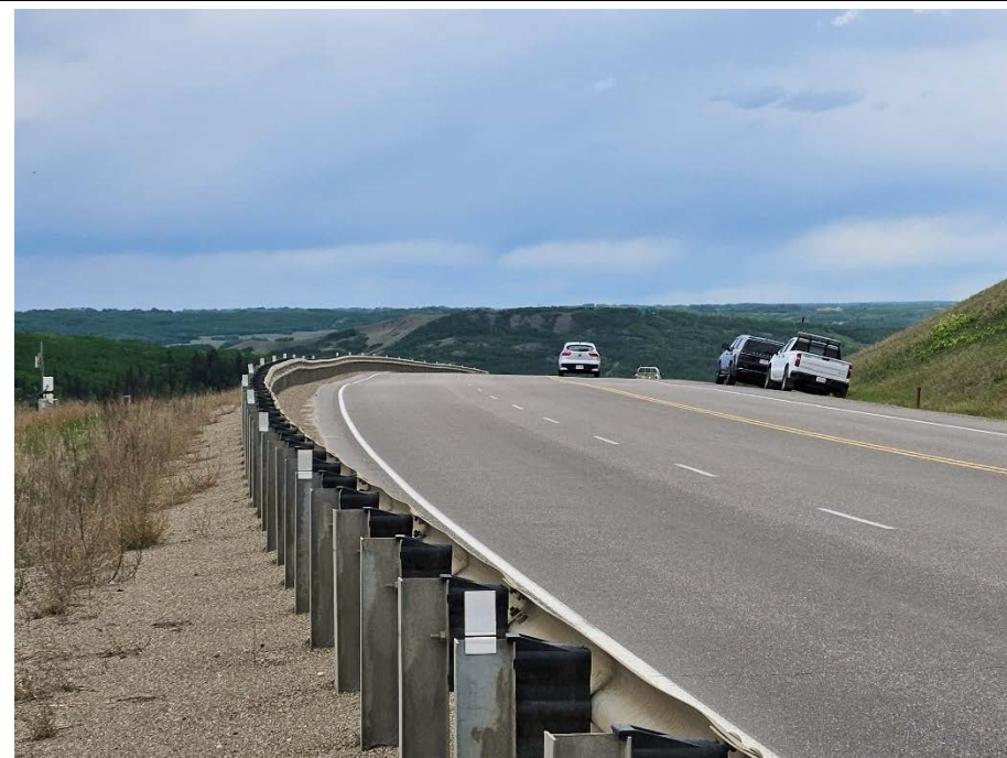
Photo 70-08. Looking west along highway above pile wall. Visible dip in guardrail (near 33+900) suspected from install and likely not related to slide related settlement that occurred prior to the pile wall. No cracking or other slide related distress was visible in pavement along previous damage extents since the highway was repaved in 2022.
