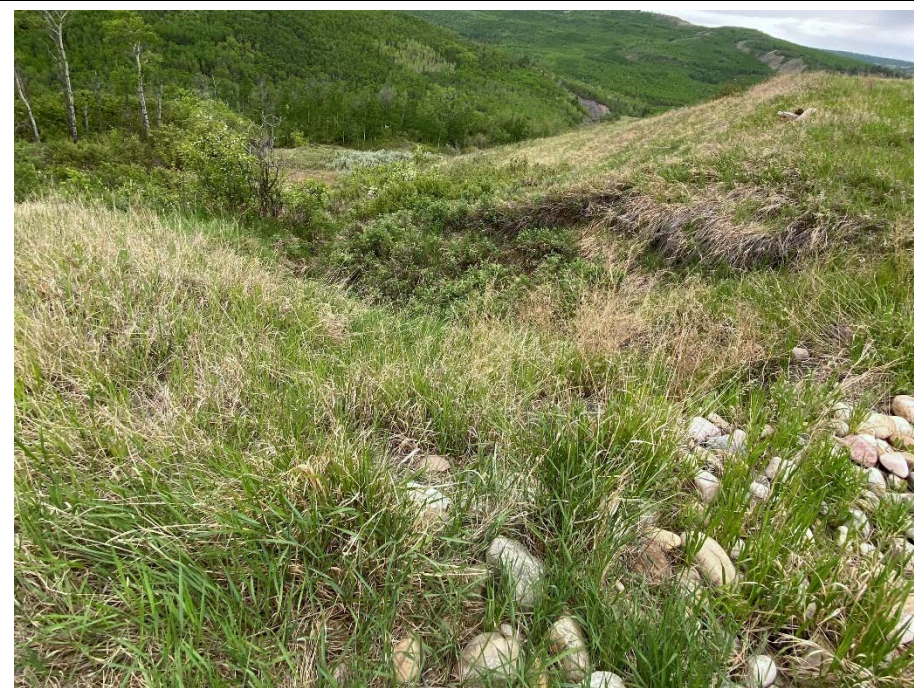
Photo 70-06. Looking south at the top of the erosion gully at the downstream end of the armoured drainage outlet (34+015). Slightly worse but gully sidewalls have grass growth.
