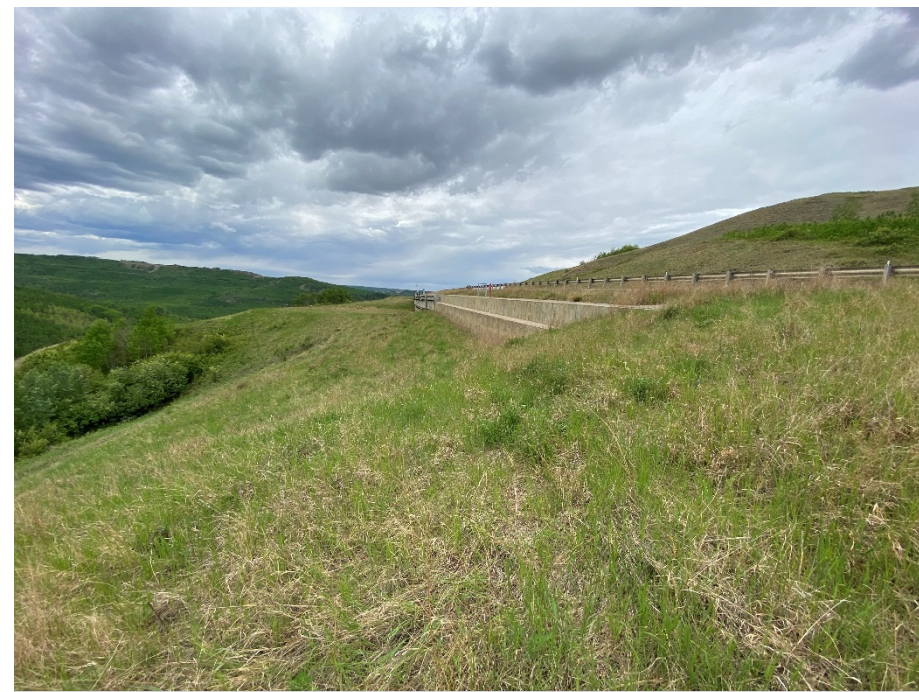
Photo 70-01. Looking west at concrete pile retaining wall at 33+850. No major visible changes downslope from the wall since 2023.
