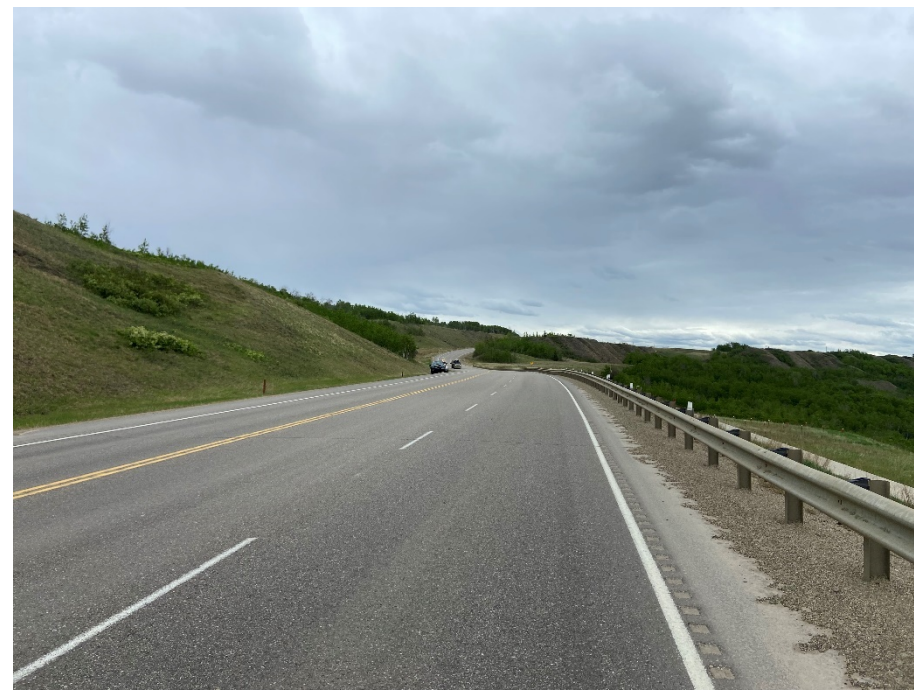
Photo 70-07. View along highway looking east above pile wall. No pavement disturbance was visible since the Fall 2022 repaving.
