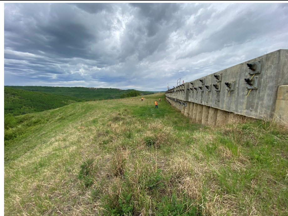
Photo 70-02. Looking west from the east end of the 2017 concrete pile retaining wall near 33+875.
