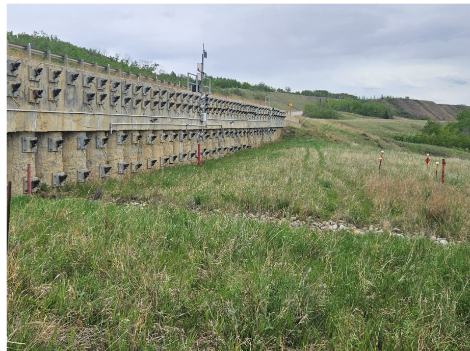
Photo 70-03. Looking east near the centre of the retaining wall with Class 1 riprap swale located near 33+950. East flank of the 2016 slide is visible in the background. SI13-3 is visible on the right side of the photo. No major changes were visible on the bench below the wall since 2023.
