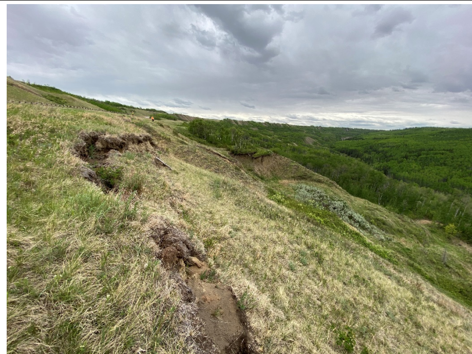
Photo 70-10. Looking east at main scarp expansion west of the pile wall near 34+100 with increased movement since 2023. Dropdown of the scarp in this area was up to 0.8 m in height. Increase dropdown and lateral expansion along previously observed tension cracks. No major retrogression towards the highway was observed. Lower slide terrain has ongoing movement but no major visible changes.
