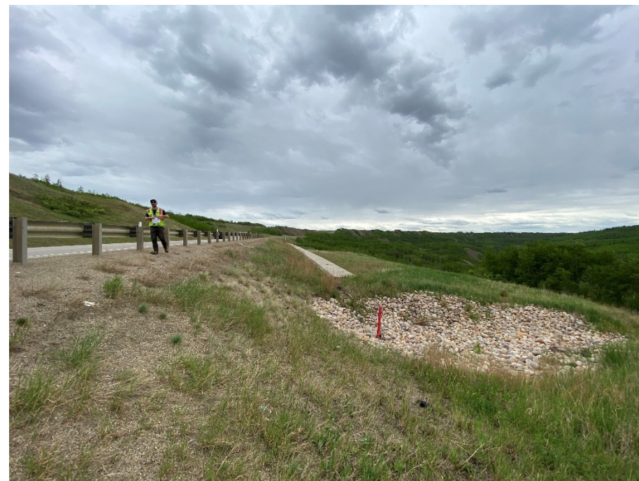
Photo 70-05. View east from west end of pile wall (km 34+015) at armoured drainage outlet for the drain trough along top of wall. Trough drain was open and working as intended with some minor debris and sediment buildup. Overall no major changes from the 2023 condition.
