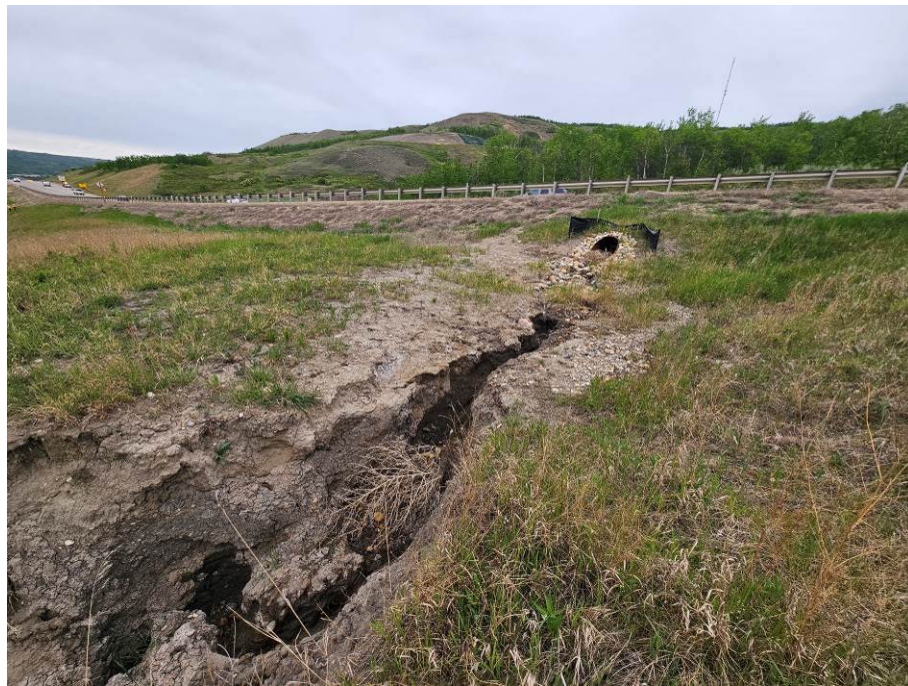
Photo 61-01. Looking north at culvert outlet with increased gully erosion depth near km 36+225.
