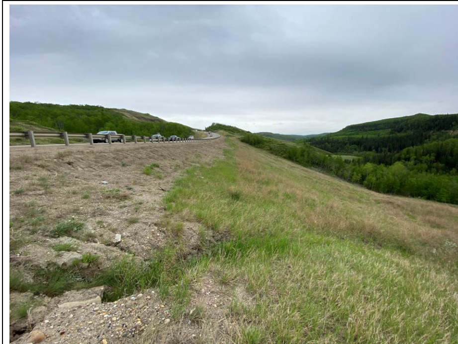
Photo 61-05. View towards the southeast from km 36+450 where three shallow slumps are located on the embankment downslope from the highway. Erosion rill is visible within the bottom of the photo which appeared similar to the 2022 condition.
