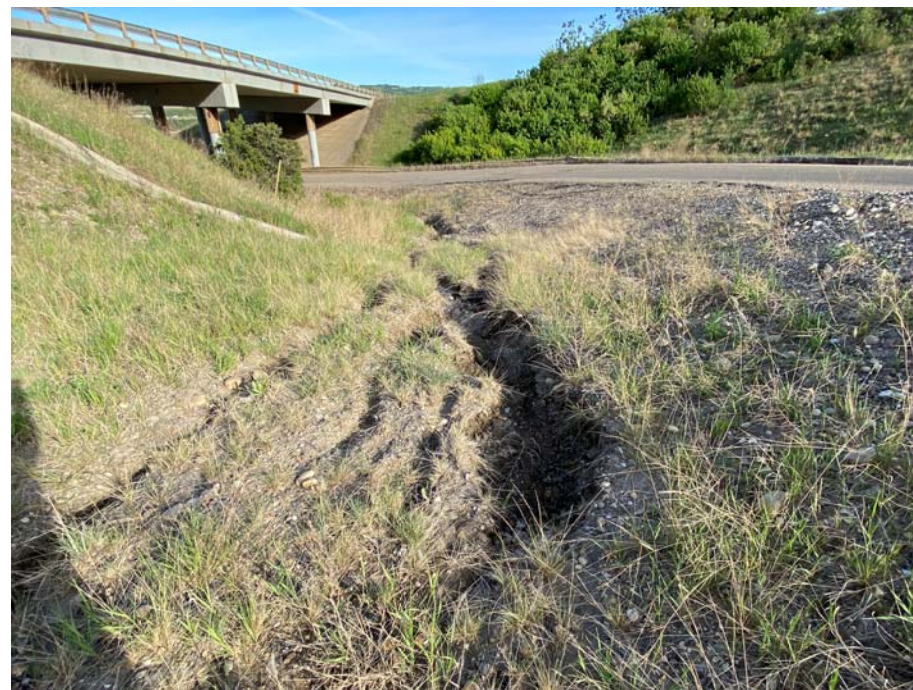
Photo 61-08. Looking northwest at increased ditch erosion at the base of the eastern Grouard bridge embankment (km 37+100). Erosion gully has formed up to 0.8 m wide and 0.6 m deep.
