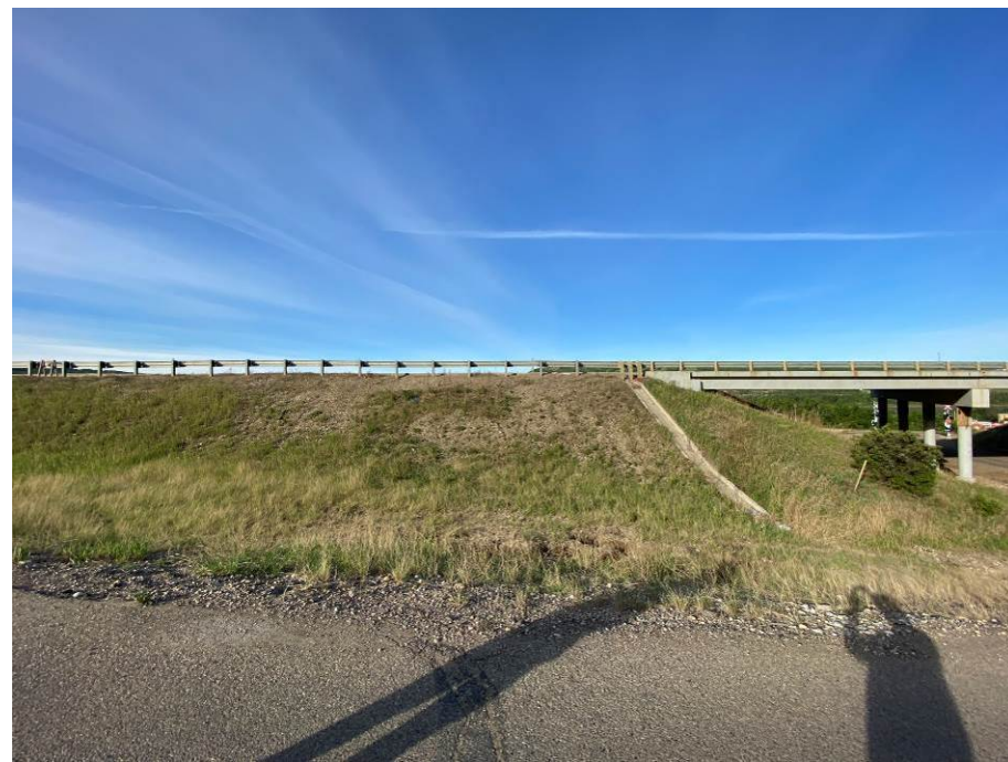
Photo 61-07. View southwest of the east Grouard bridge embankment (km 37+100) where there was previous gully erosion damage that was repaired in Fall 2022. There were minor rills and vegetation disturbance (likely from winter salt) but overall repairs were in good condition and the curb/swale drainage system was functioning as intended.
