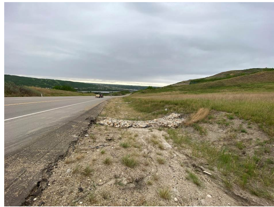
Photo 60-09. Looking west towards the north ditch where Fall 2022 erosion repairs were completed with gabion check dams installed between approximately km 36+050 and km 36+300.
