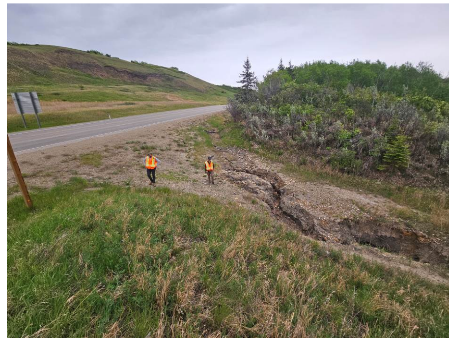
Photo 60-05. View south towards erosional gullying occurring below the roadway where ditch runoff enters near km 36+050. Top of the gullying was slightly deeper and closer to the highway relative to the 2022 condition.
