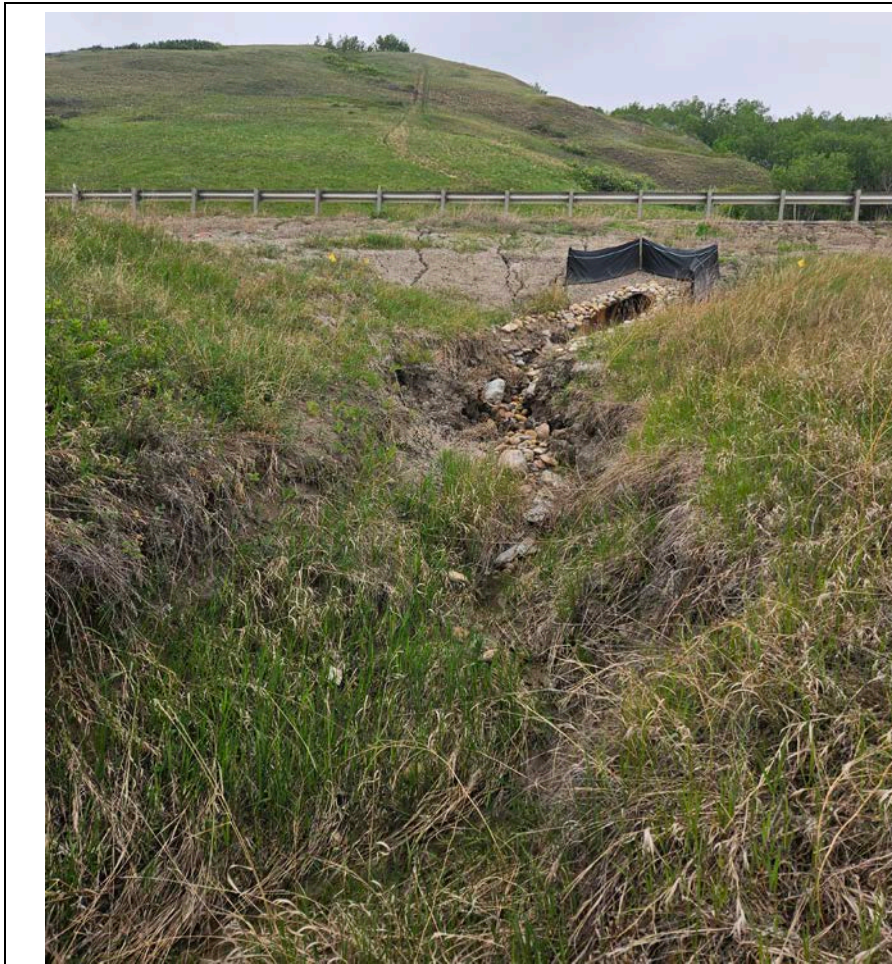
Photo 60-01. View north towards the culvert outlet near km 35+675. As part of Fall 2022 repair work, a 900 mm diameter SWSP liner was installed and rock armoring was added at the inlet and outlet. Ongoing erosion downstream of culvert and rilling above. Scour depth below culvert inlet was 0.3 m.
