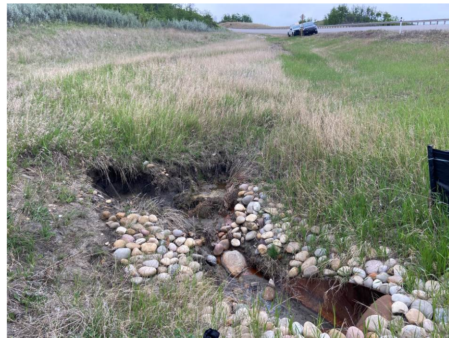
Photo 60-08. Minor erosion at the culvert inlet near km 35+675. Culvert was lined and had rock armoring added as part of the Fall 2022 repairs. Erosion damage was approximately 0.5 m wide and there was a 0.2 m drop.
