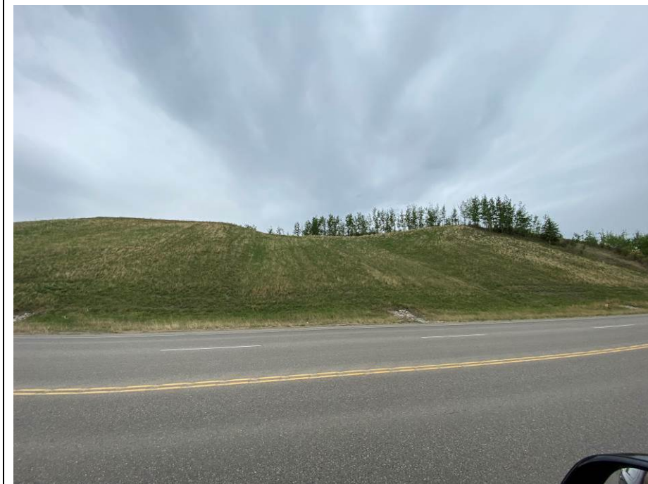
Photo 60-03. View south towards the backslope near km 35+830 where a landslide had previously developed. As part of the Fall 2022 repair work the backslope was cut back flatter and regraded. New slope configuration was well vegetated and in good condition.
