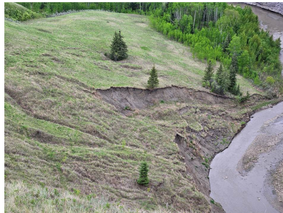
Photo 60-07. Looking southeast at active sliding at the bottom of the Heart River valley near KM 35+600 (downslope from PH059 site). Increased downdrop and expansion of the sliding area as the slide material and valley toe soils are eroded by the river.
