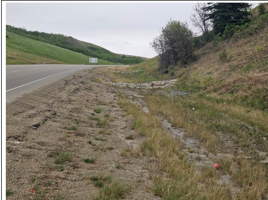
Photo 60-04. Looking east near km 35+950 at the regraded south ditch. ECM and gabion check dams installed as part of Fall 2022 repairs.
