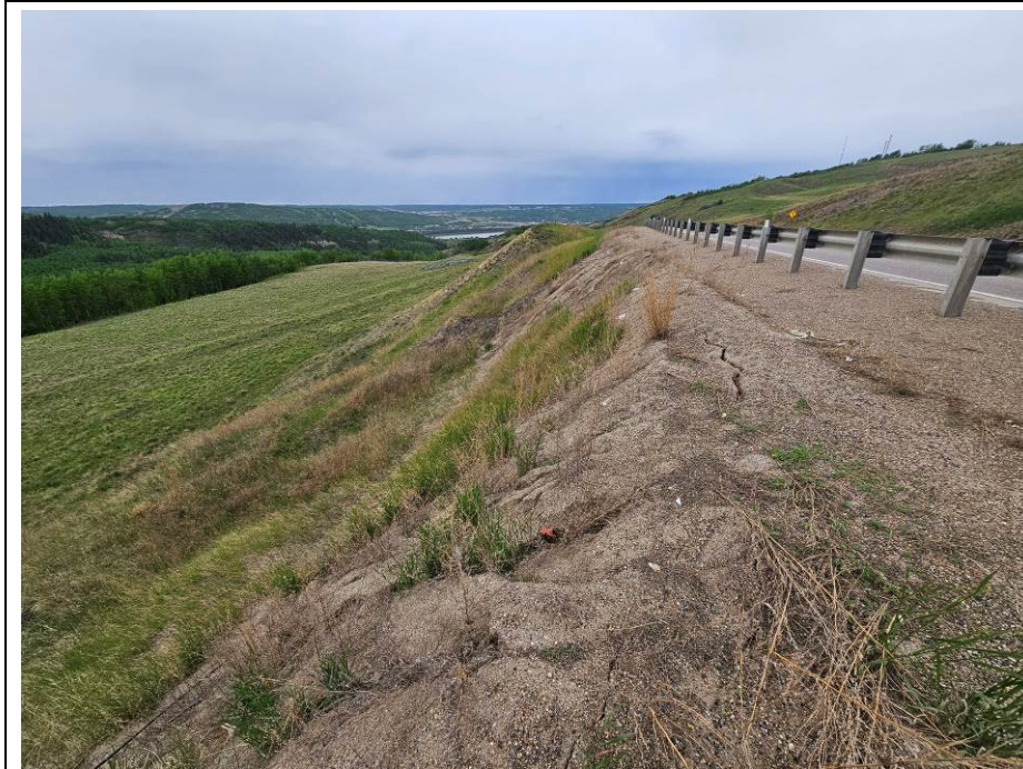
Photo 59-01. Looking northwest at headscarp area of shallow landslide on downslope side of roadway first observed in 2007 (34+850). There was additional downslope movement of the slide mass, a new tension crack was observed above the main scarp, there was some rill erosion in the upper scarp and reduced vegetation growth (likely a result of winter salt and sanding).
