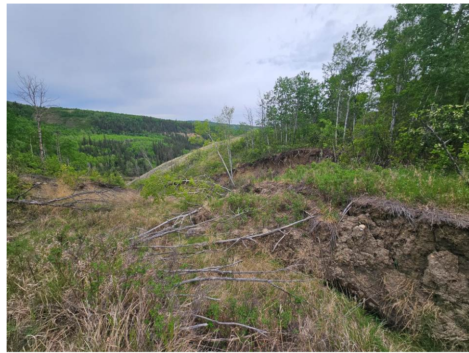
Photo 59-11. Looking southwest at the erosion gully / slide area downstream of the erosion gully near KM 35+500. Ongoing erosion and slide movement but no significant retrogression towards the highway (main headwall offset approximately 115 m from the highway). More trees have fallen into gully due to the collapse of the gully sidewalls.
