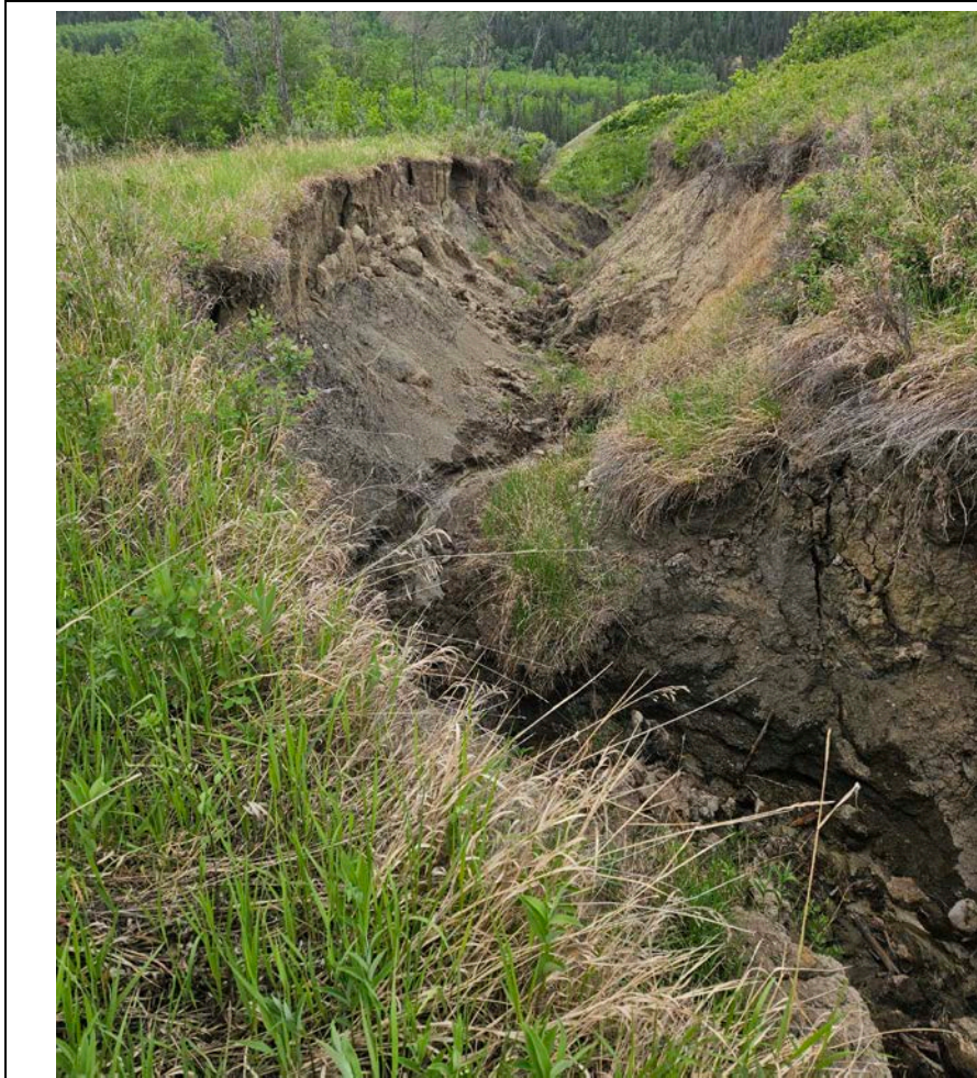
Photo 59-10. Looking southwest at the erosion gully downstream of the gabion culvert outlet (35+500). Ongoing erosion and flank expansion relative to the 2022 condition.
