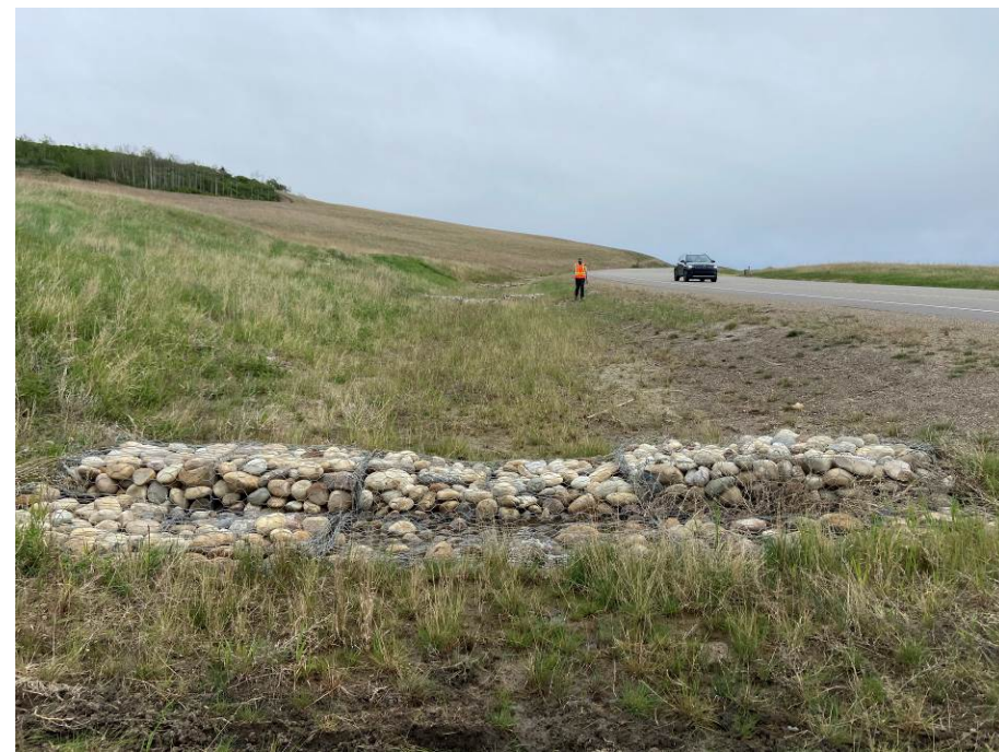
Photo 59-07. Looking east towards the Fall 2022 north ditch repair section (35+200 to 35+350) with gabion basket check dams. Similar repairs were also completed within this section in the south ditch.
