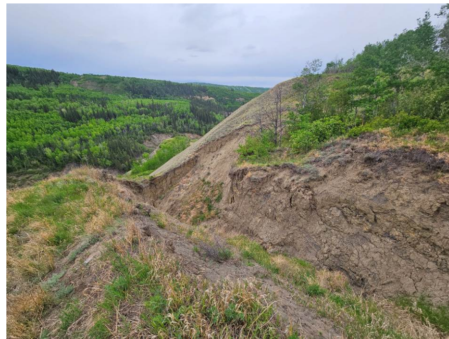
Photo 59-06. Looking west at headwall area of an erosion gully approximately 125 m downslope (south) from the highway (35+450). Ongoing erosion and sliding of the vertical sidewalls and some minor expansion relative to the 2022 condition but no major headwall retrogression.
