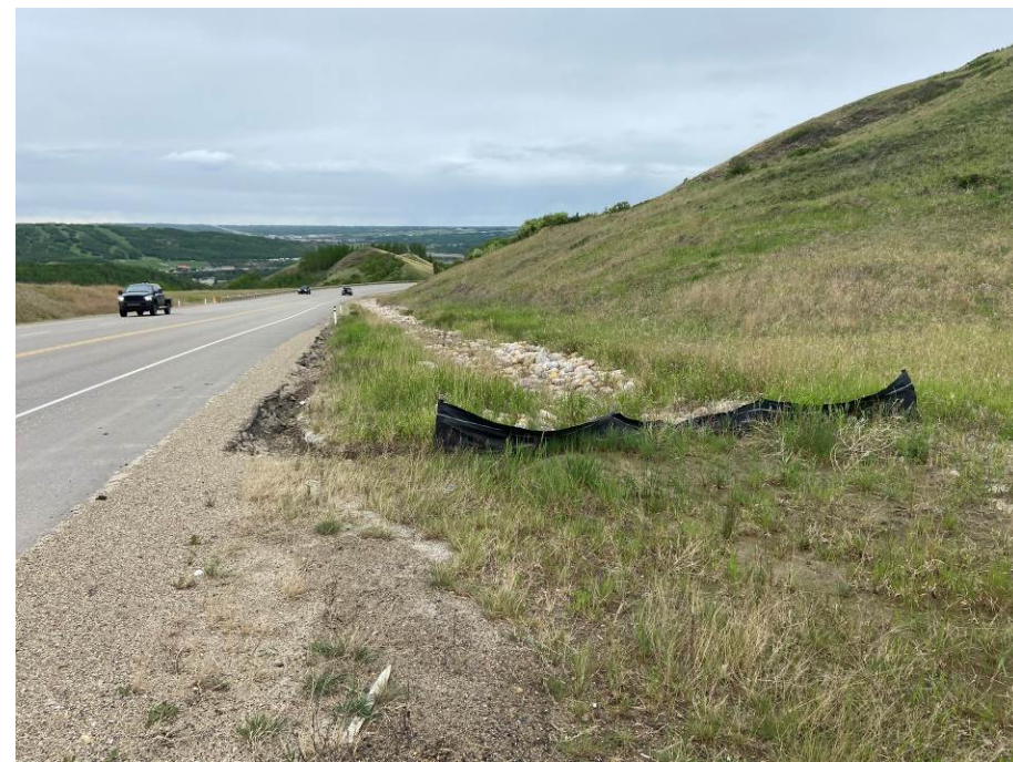
Photo 59-08. Looking west at north ditch erosion damage starting at the downstream end of the 2022 repair section near 35+350. Water flow has been directed outside the gabion ditch armouring and eroded along the edge of the pavement shoulder due to the silt fence. Erosion channel was up to 0.3 m wide and 0.2 m deep.
