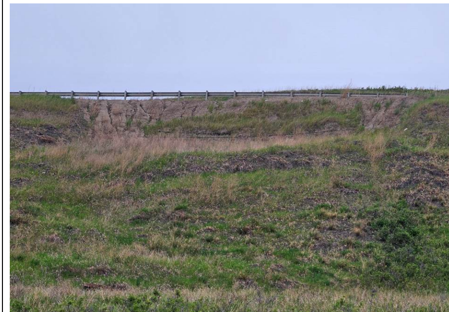
Photo 59-02. Looking north (upslope) from the base of the slide area near 34+850. Increased downslope movement of the slide mass relative to the 2022 condition. Rill erosion visible in the backscarp. Scarp is still offset 0.8 m from the guardrail (unchanged since 2022).
