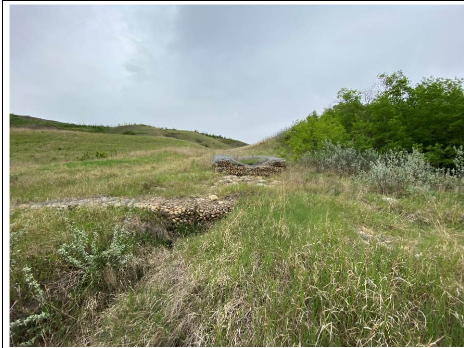
Photo 59-09. View northeast downslope from the gabion culvert outlet structure (35+500). There was a 0.5 m scour drop below the downslope row of gabion baskets that drains towards a much large erosion gully.
