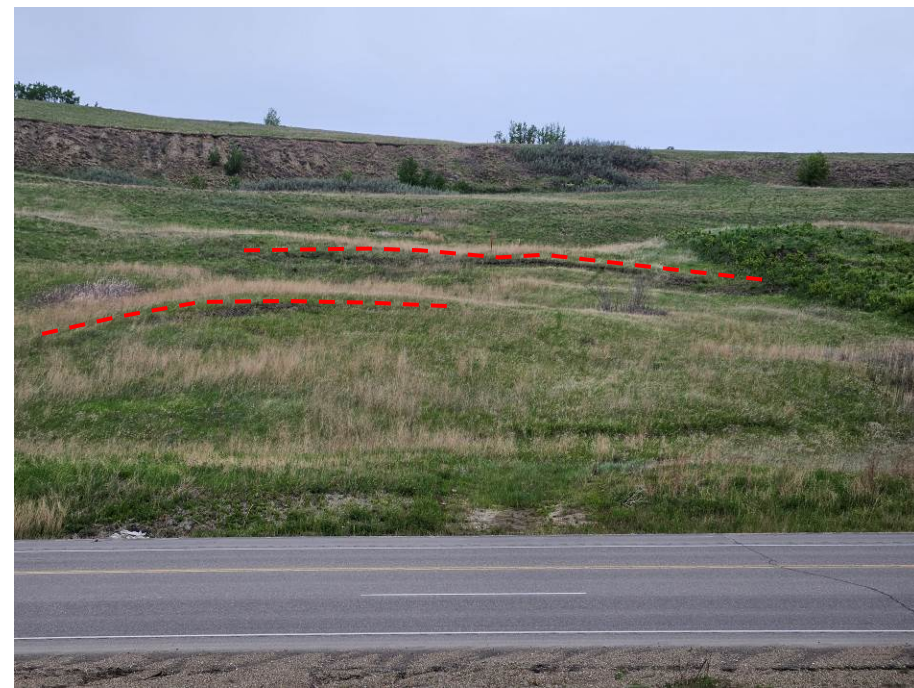
Photo 59-05. Looking at backslope north of the highway near KM 35+250 within historic slide terrain. Potential new slide scarps and tension cracks appeared to be forming within the disturbed slide toe deposits approximately 75 m to 100 m upslope from the highway ditch near 35+250.
