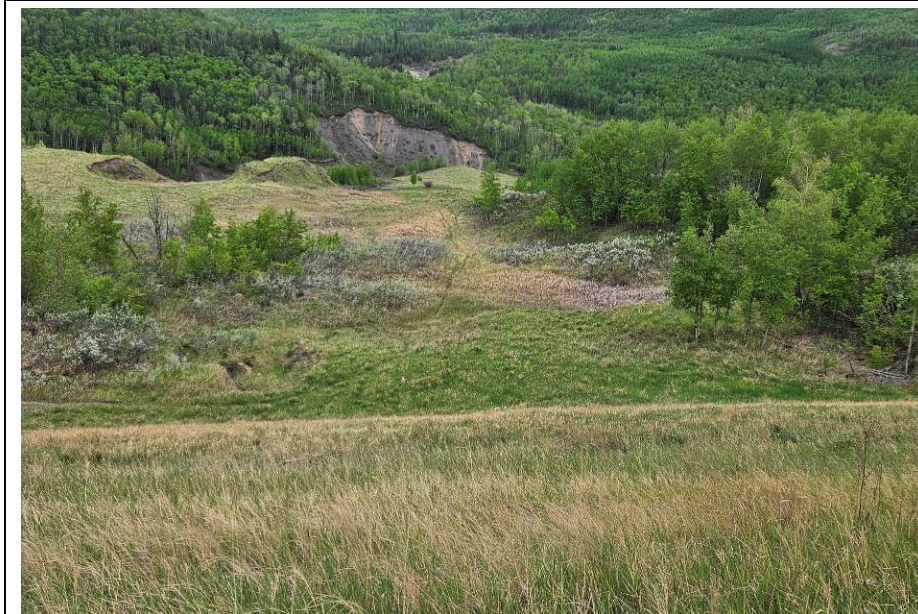
Photo 2-12. Downslope (south) view of the mid-slope below the road embankment near 34+550 (Old Site 1). No visible changes from the 2022 condition.
