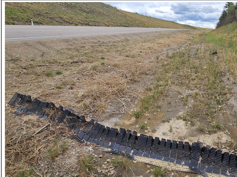
Photo 2-06. Looking east towards the south road ditch where there was previous erosion damage between 33+300 to 33+715 that was repaired in Fall 2022. Ditch was regraded and ECB and synthetic check dams were installed.
