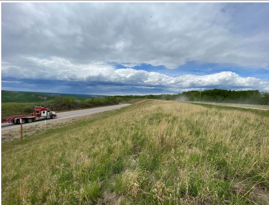
Photo 2-02. Looking northwest at cut slope area with previous shallow slumps on the northeast side of the road (33+100). Backslope regrading and granular replacement was completed as part of the Fall 2022 repair work. Repaired slopes were good condition, well vegetated and no new slide damage was observed.
