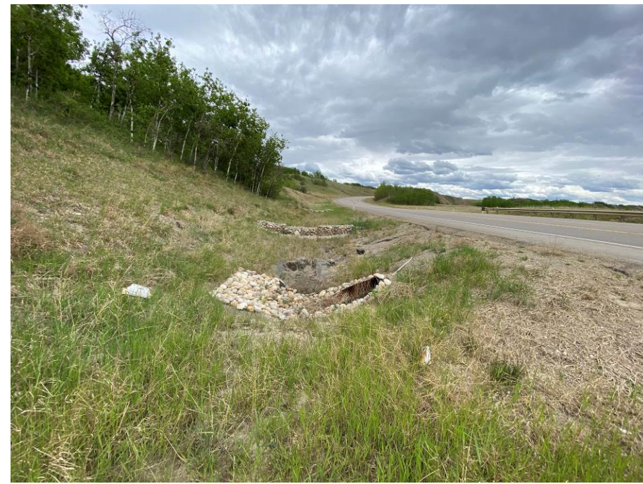
Photo 2-08. Looking east within the north ditch at the culvert inlet near 33+715 that was relined with SWSP and inlet/outlet rock armoured during the 2022 repairs. Minor erosion area (0.3 m x 0.2 m) was noted within the ditch bottom upstream of the inlet.
