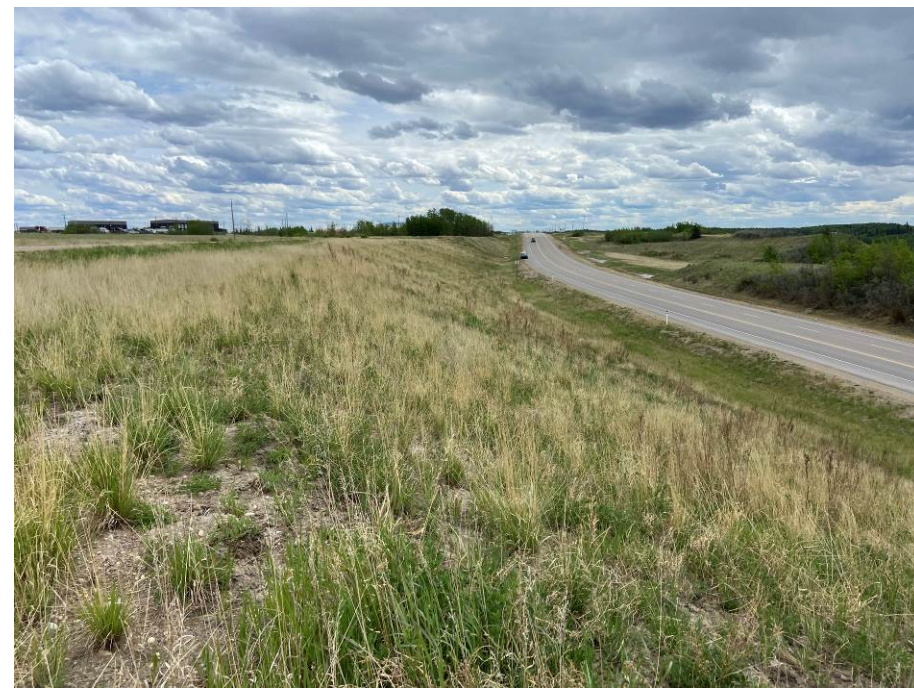
Photo 2-03. Looking southeast at the cut slope repair section (33+150). No new slide damage was noted.
