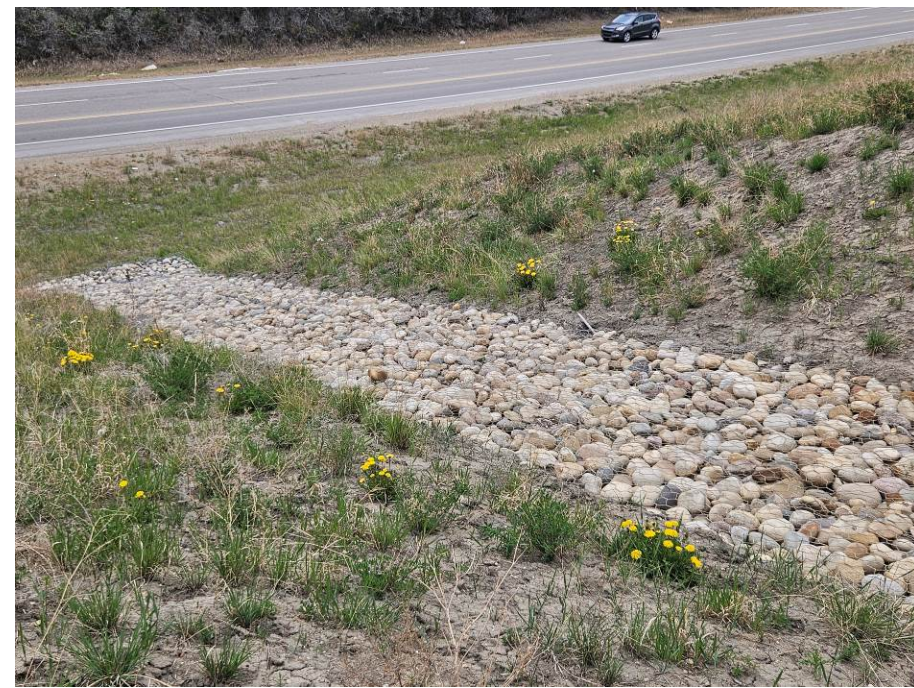
Photo 2-04. Looking south from the top of a gabion mattress armoured drainage swale installed near km 33+175 as part of the Fall 2022 repair work. The swale conveys ditch flow from the gravel road above the cut slope. Some minor erosion was noted at the edges of the mattress at the base to swale side slope transition.
