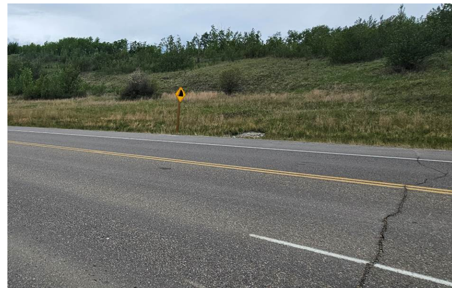
Photo 2-07. Looking northwest towards the shallow slump north of the highway near 33+550. Previous slide toe material that was encroaching into ditch cleaned out as part of the ditch regrading work in 2022.
