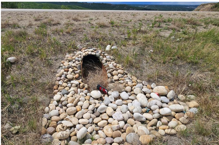
Photo 2-01. Previously damaged and partially buried culvert inlet was repaired and rock armoured at 33+000 as part of the Fall 2022 overlay and repair work.
