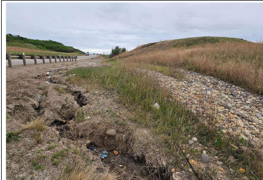
Photo 2-11. Looking east at slightly worse erosion gully from ditch flow outside the armored swale near 34+450.
