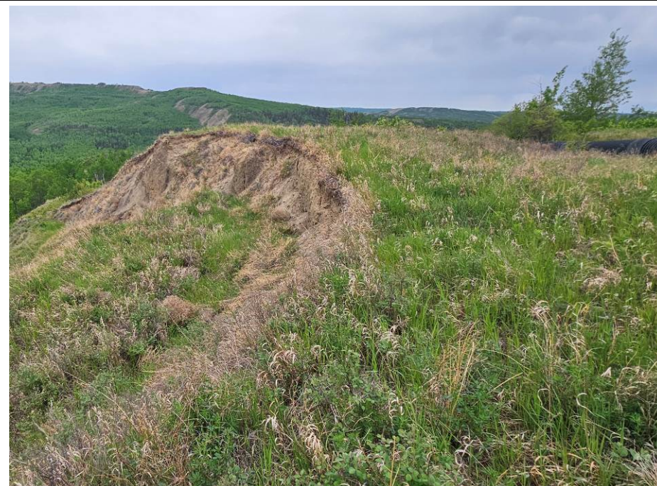
Photo 2-14. View southwest of the 6 m backscarp near the top of trunk drain, near 34+625. No major changes visible since 2022.
