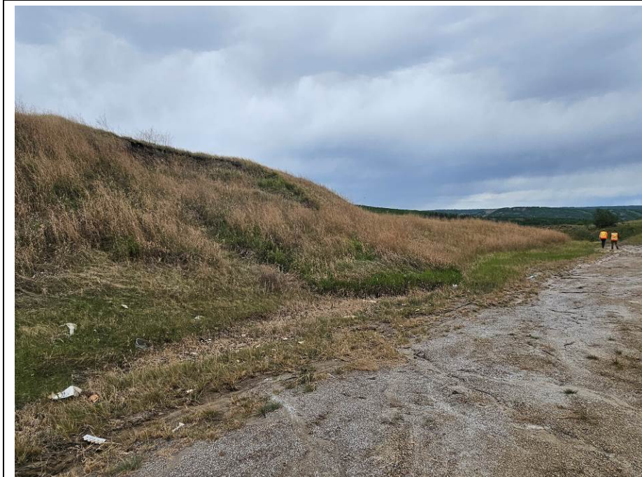
Photo 2-10. Backslope slump near 34+000 south of highway had no visible changes from the 2022 condition.
