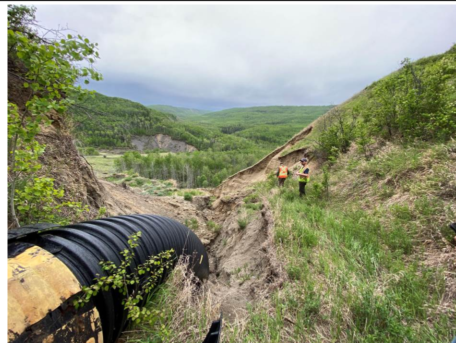
Photo 2-15. Looking east at the trunk drain breach (34+650). Significant gully erosion and landsliding has developed upslope from the initial breach. Terrain is actively eroding and sliding that is expected to continue to retrogress upslope. Diversion of the current trunk drain to a new alignment is required to slow the erosion.
