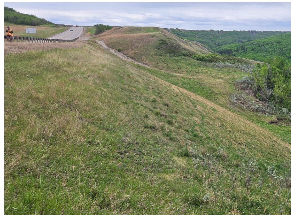
Photo 2-13. Looking east towards the road fill embankment between 34+450 to 34+600 (old Site 1). No visible changes from the 2022 condition.
