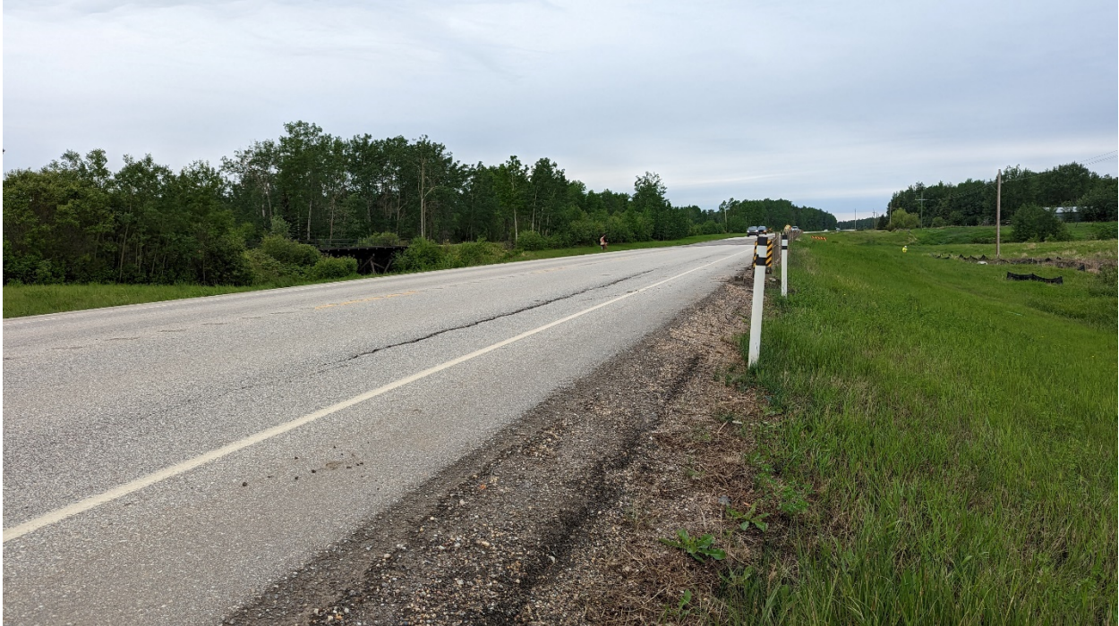
Photo 11 – Looking west at crack near east end of guardrail which is on the other side of the culvert from the main area of movement.
