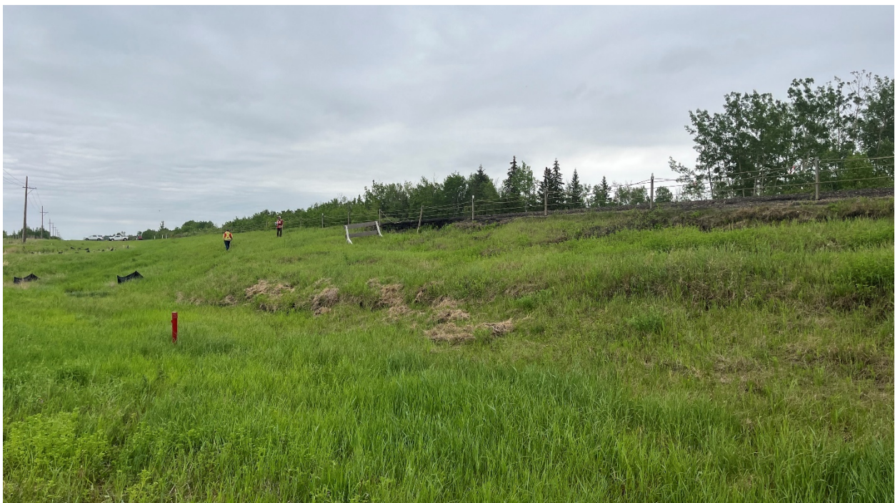
Photo 4: Looking southeast at the east end of the slump; note the presence of a well-defined toe roll.
