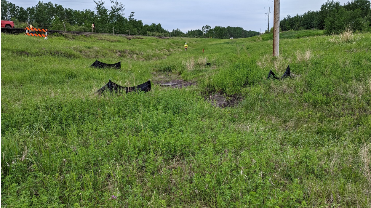
Photo 1 – Looking southwest at slump in north shoulder.
