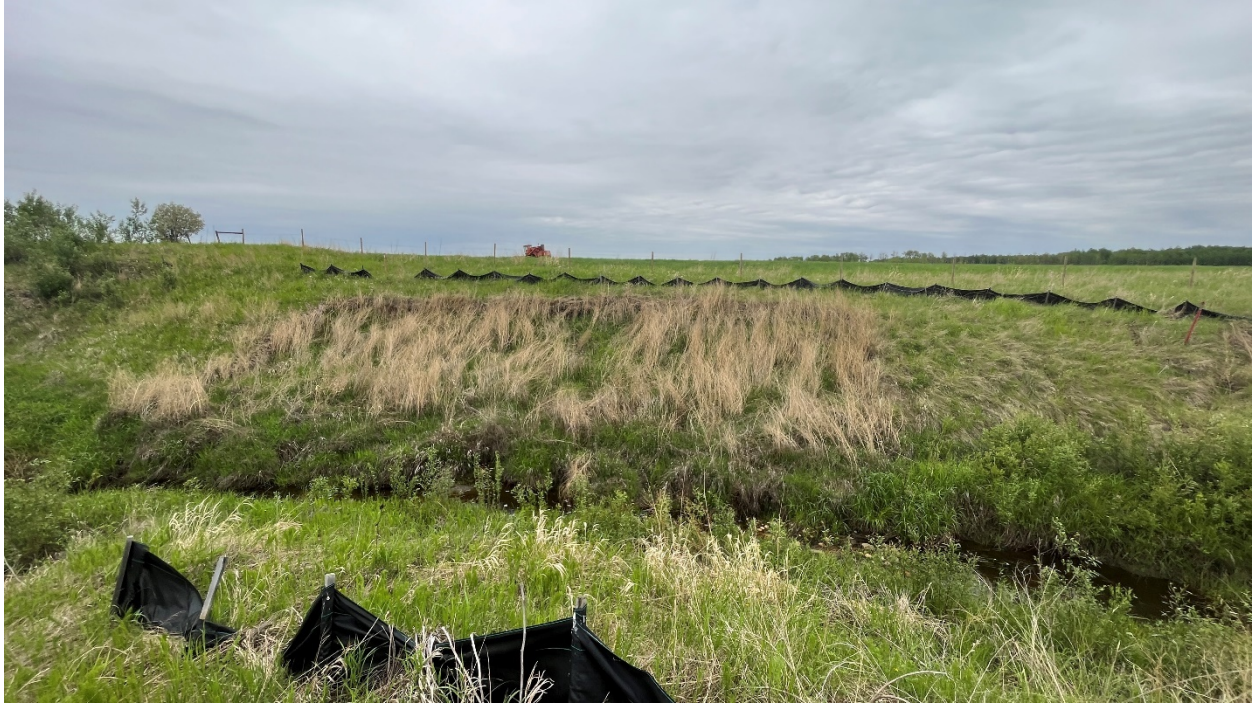
Photo 9 – Looking northeast at slump on east side of channel.
