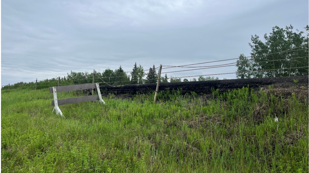
Photo 5 - Looking southeast at undermined guardrail and exposed pavement structure.
