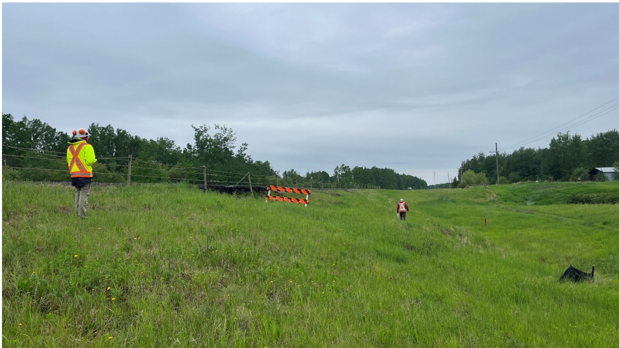
Photo 2 – Looking west from the east end of slump.
