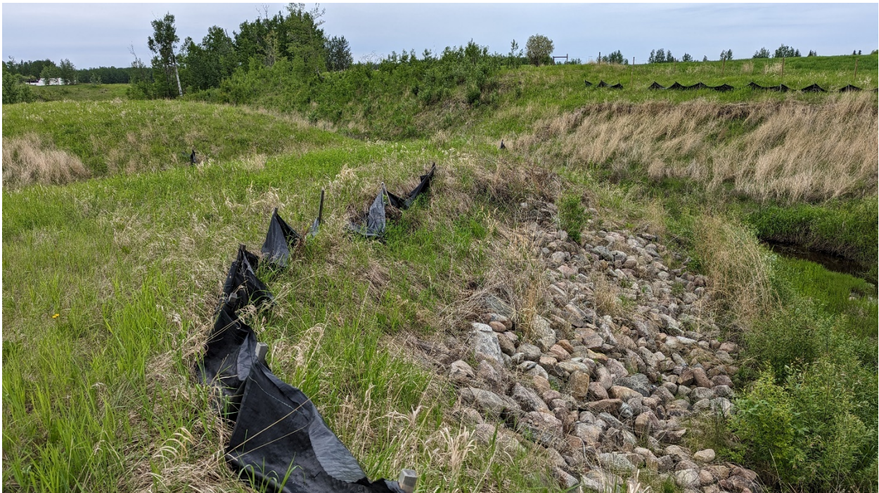
Photo 8 – Looking at slumping above west riprap (somewhat obscured by grass).
