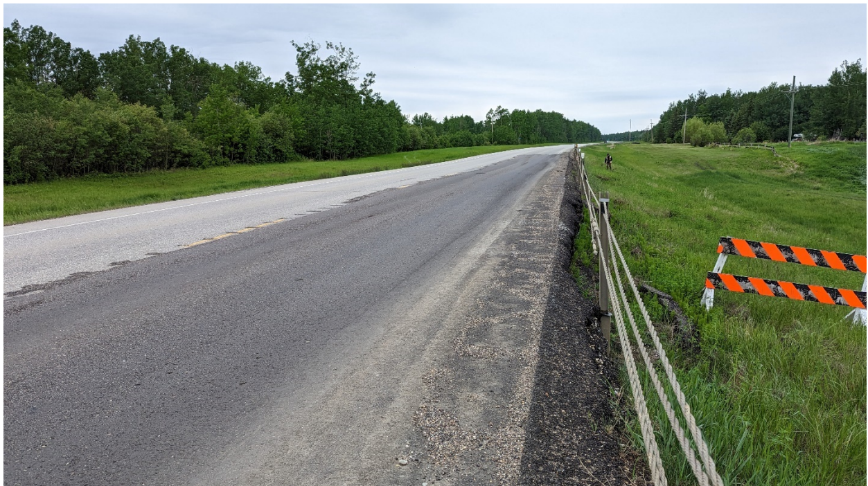
Photo 6 - Looking west at location of previous cracks and subsidence in highway above scarp shown in Photo 5.
