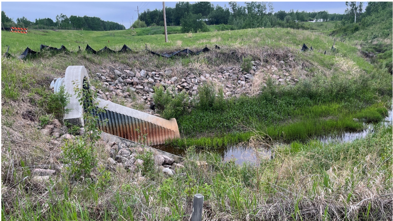
Photo 10 – Looking west at culvert outlet, with slump beyond, and riprap with minor movement.
