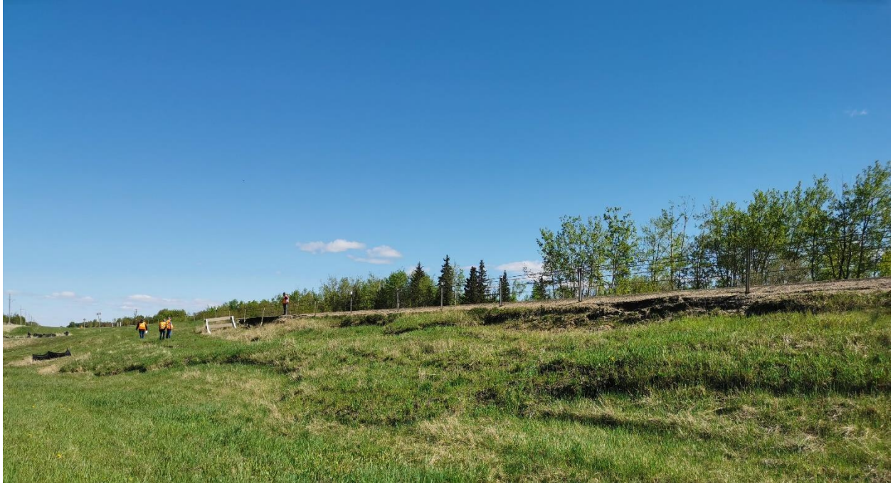
Photo 3 – Looking southeast at east end of slump.
