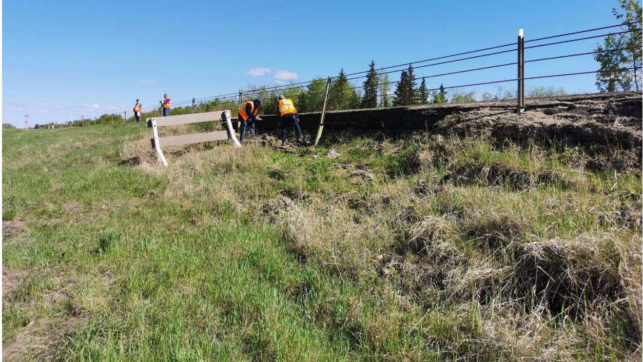
Photo 5 – Looking southeast at undermined guardrail and exposed pavement structure.
