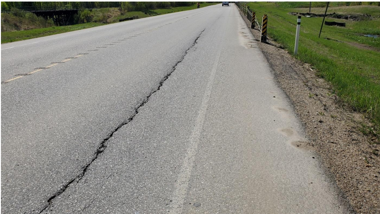
Photo 12 – Looking west at the same crack shown in Photo 11 which may be related to separate movement zone.
