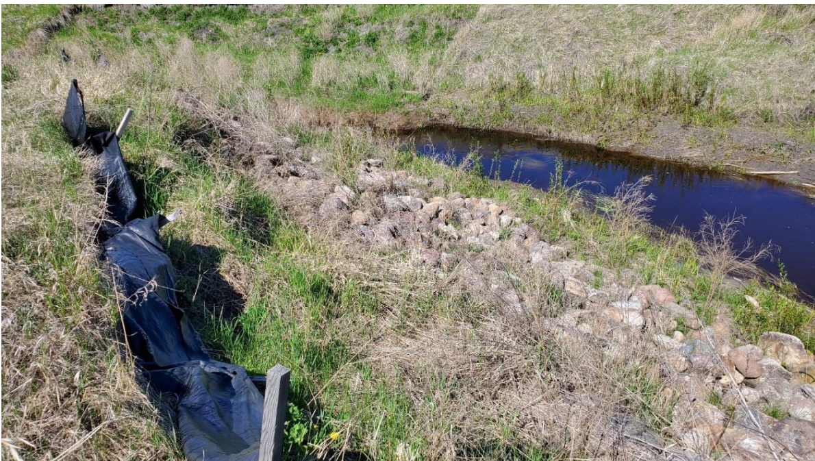
Photo 8 – Looking at slumping above west riprap (somewhat obscured by grass).
