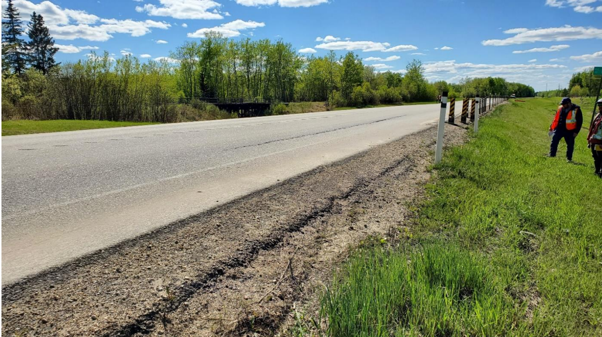
Photo 11 – Looking southwest at crack near east end of guardrail which is on the other side of the culvert from the main area of movement.
