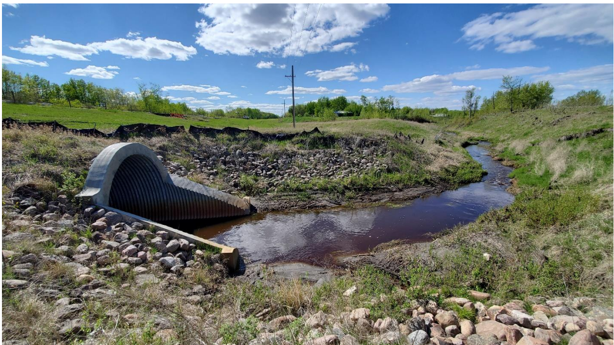
Photo 10 – Looking west at culvert outlet, with slump beyond, and riprap with minor movement.
