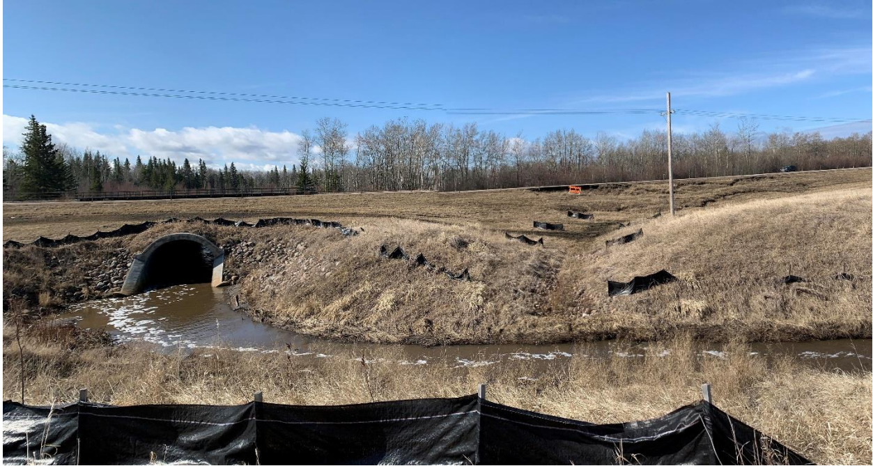
Photo 1 (AT, May 3, 2022) - Looking south across creek at slump in north shoulder.
