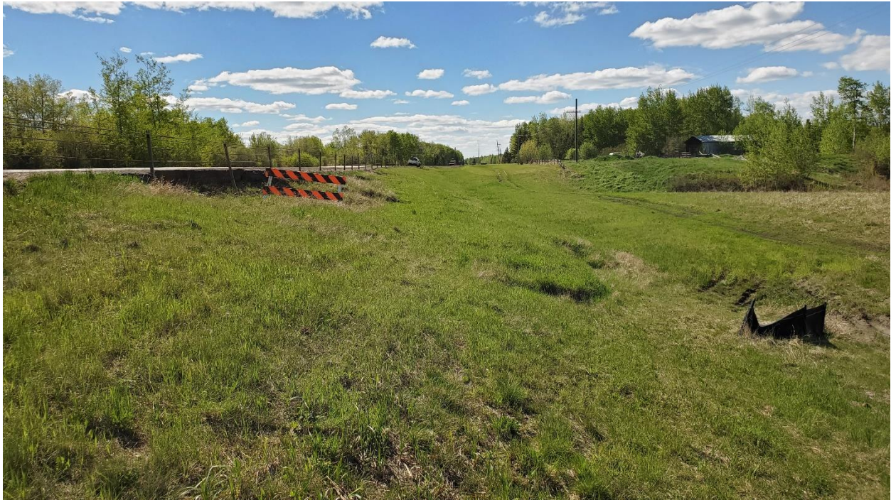
Photo 2 – Looking west from east end of slump.
