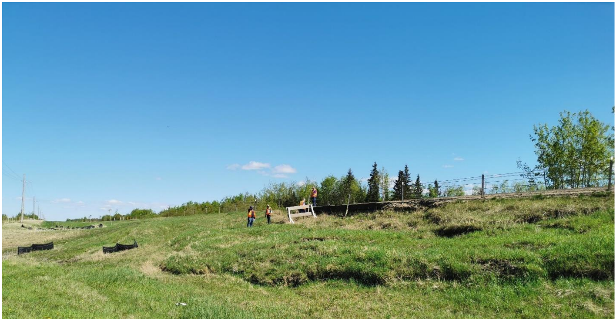
Photo 4 – Looking southeast at east end of slump.
