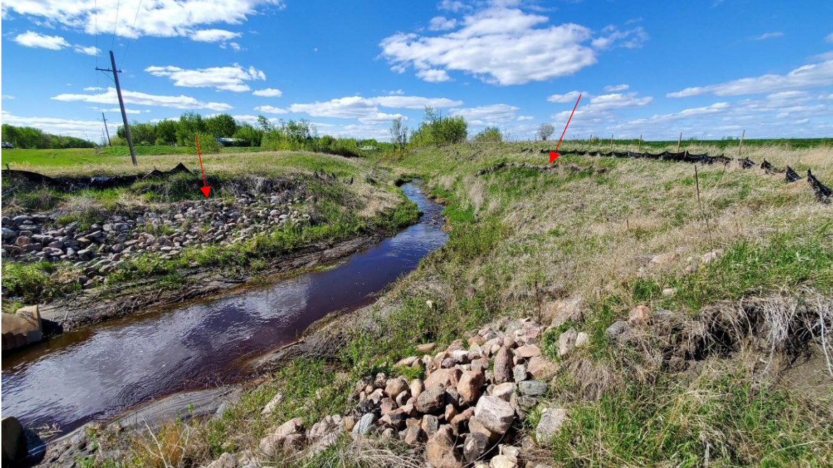
Photo 7 – Looking north (downstream) along the creek. There is minor slumping at the top of the riprap on the west (left) side and a larger slump further downstream on the right (east) side.
