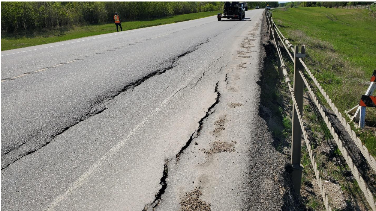
Photo 6 – Looking west at cracks and subsidence in highway above scarp shown in Photo 5.
