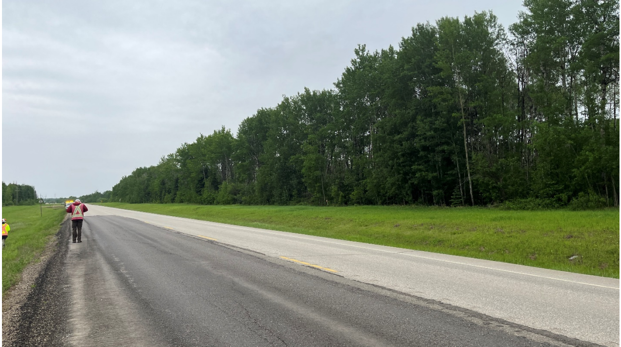
Photo 1 – Looking east along the WBL at the main landslide’s head scarp crack and highway dip.
