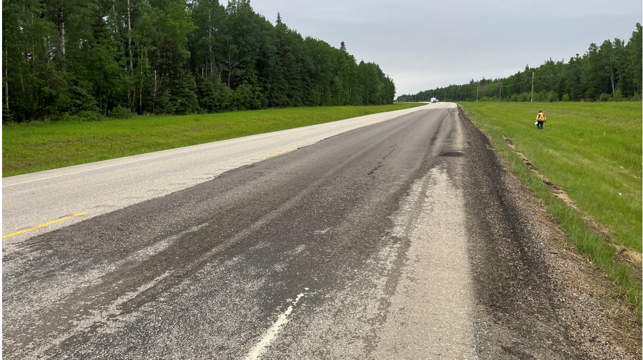
Photo 3 – Looking west at the main area of distress.
