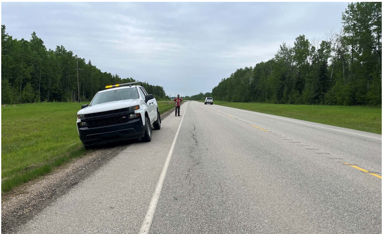
Photo 4 – Looking east along the WBL where cracks are starting to form east of the patched area.
