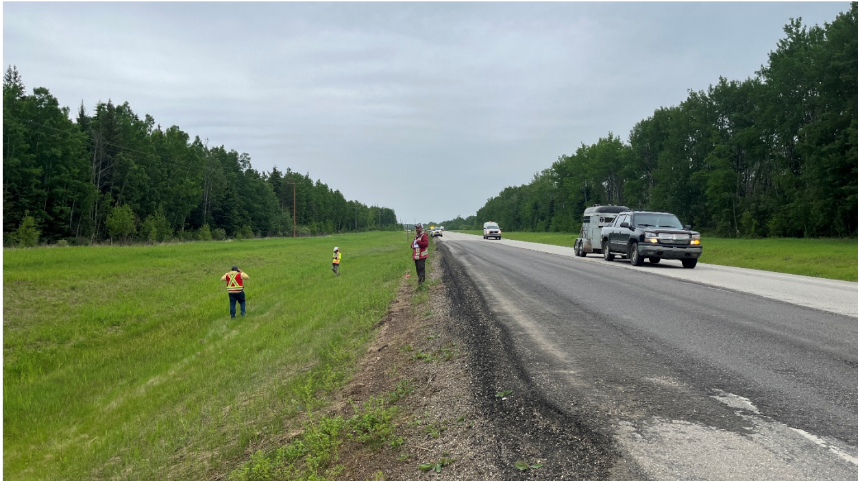
Photo 2 – Looking east at the sideslope below the main crack where a toe roll is present in the ditch.
