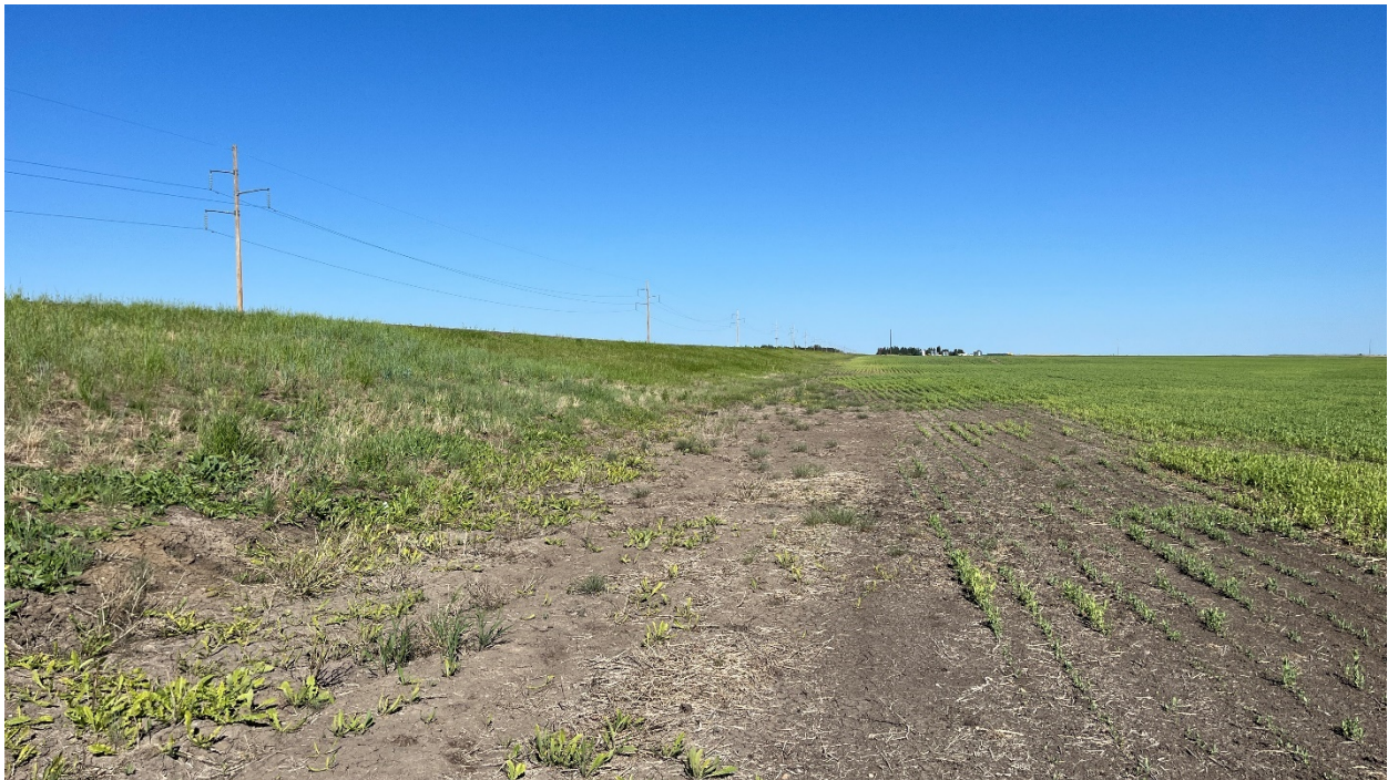
Photo 2 – Looking northeast at south slope of highway embankment from the south ditch.
