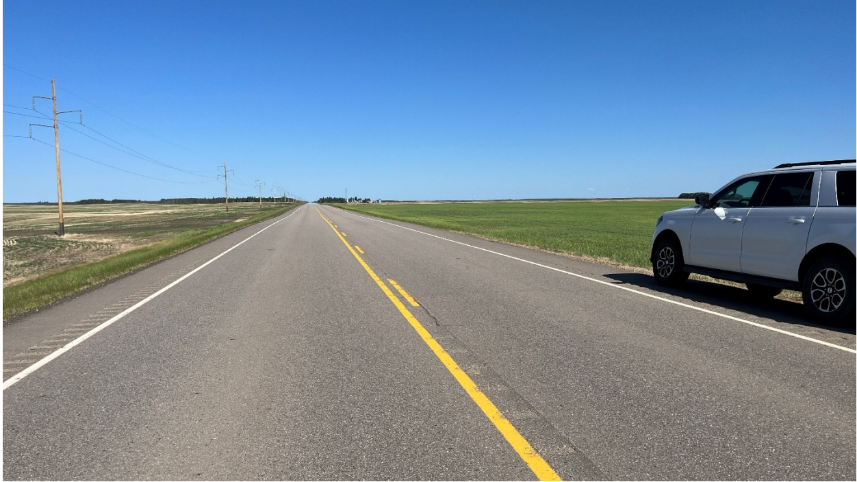
Photo 1 – Looking east from WBL at middle of the reconstructed portion of EBL.
