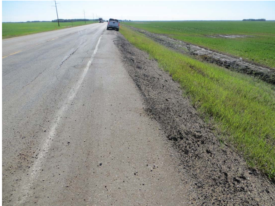
Photo 3: Looking east at east slide. Note cracks in the asphalt of the eastbound lane.
