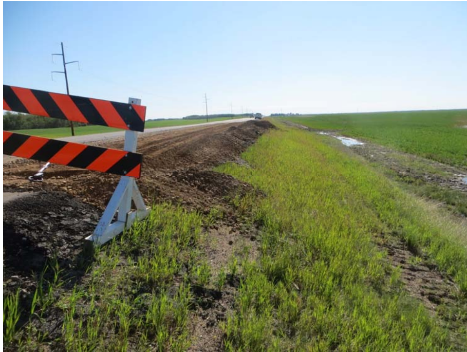
Photo 5: Looking east from west side of west slide. Note ponded water adjacent to embankment and lack of drainage.
