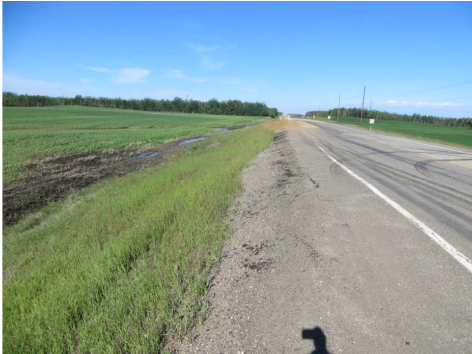
Photo 1: Looking west along south shoulder of Hwy 2A:54. Note crack of east slide at edge of asphalt and gravel placed over west side.
