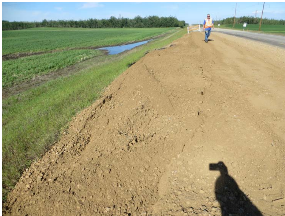
Photo 4: Looking south at west slide. Note crack through temporary gravel in line with the buried edge of asphalt.
