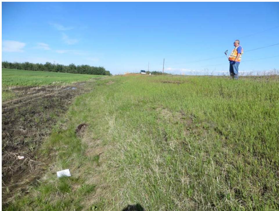
Photo 2: Looking west at east slide. Note scarp near top of embankment and toe roll at the bottom.
