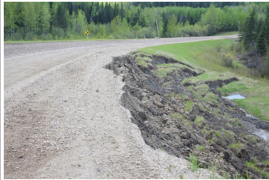
Photo 2. Looking southwest at the back scarp which has retrogressed into the highway.
