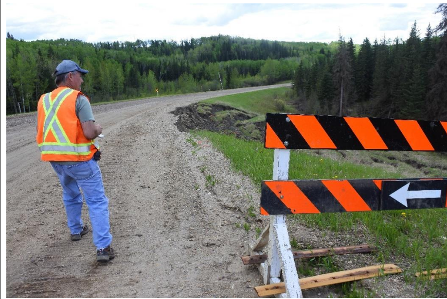
Photo 1. Looking southwest at main scarp from the road.
