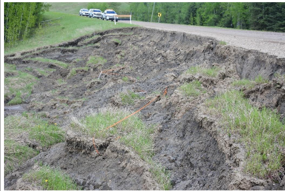
Photo 5. Looking east at back scarp and destroyed Telus line.
