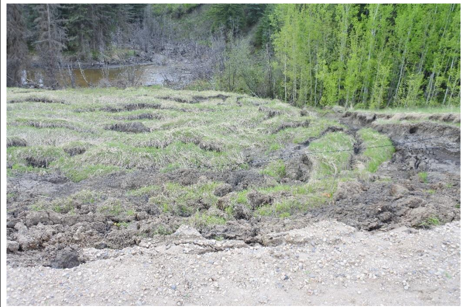
Photo 3. Looking west down at failed slide mass.
