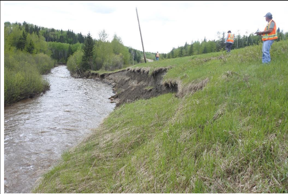
Photo 9. Looking southwest at the riverbank erosion.
