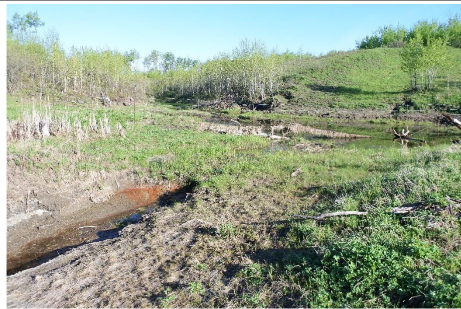
Photo 2. Looking northwest at upstream end of eroded channel.
