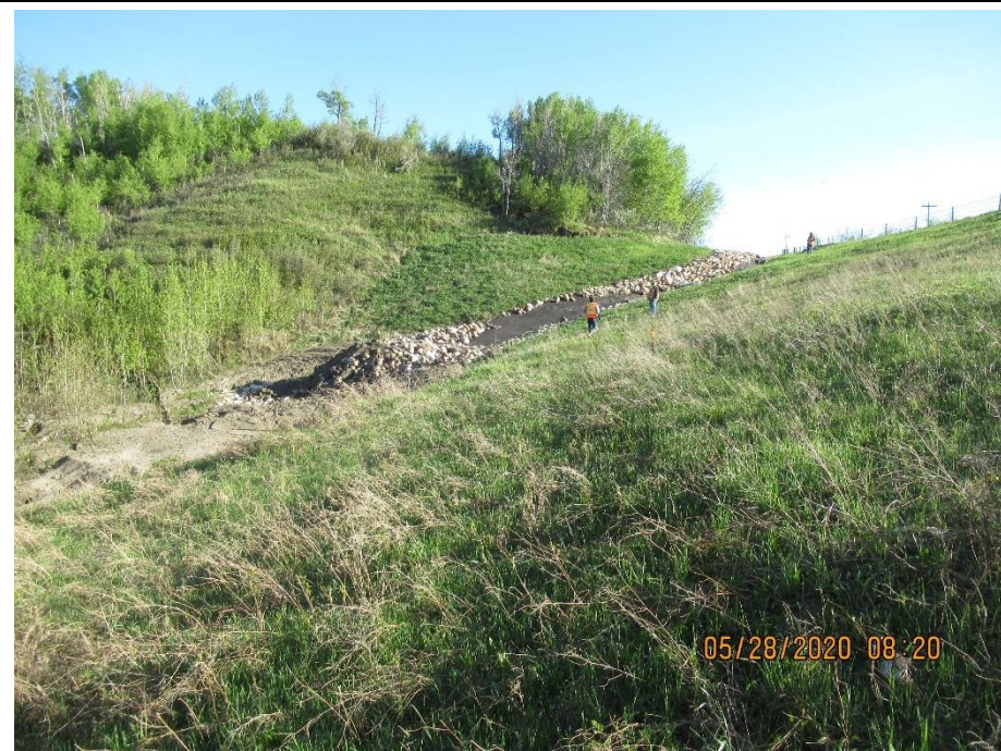
Photo 9. Looking north at the swale and debris accumulation pile below the area that had the previous erosion gully filled in.
