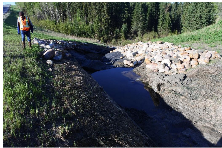
Photo 5. Looking southwest at point where flatter ditch lined with ECB meets the steeper ditch lined with rip rap. Not the extensive erosion at the curve transition.
