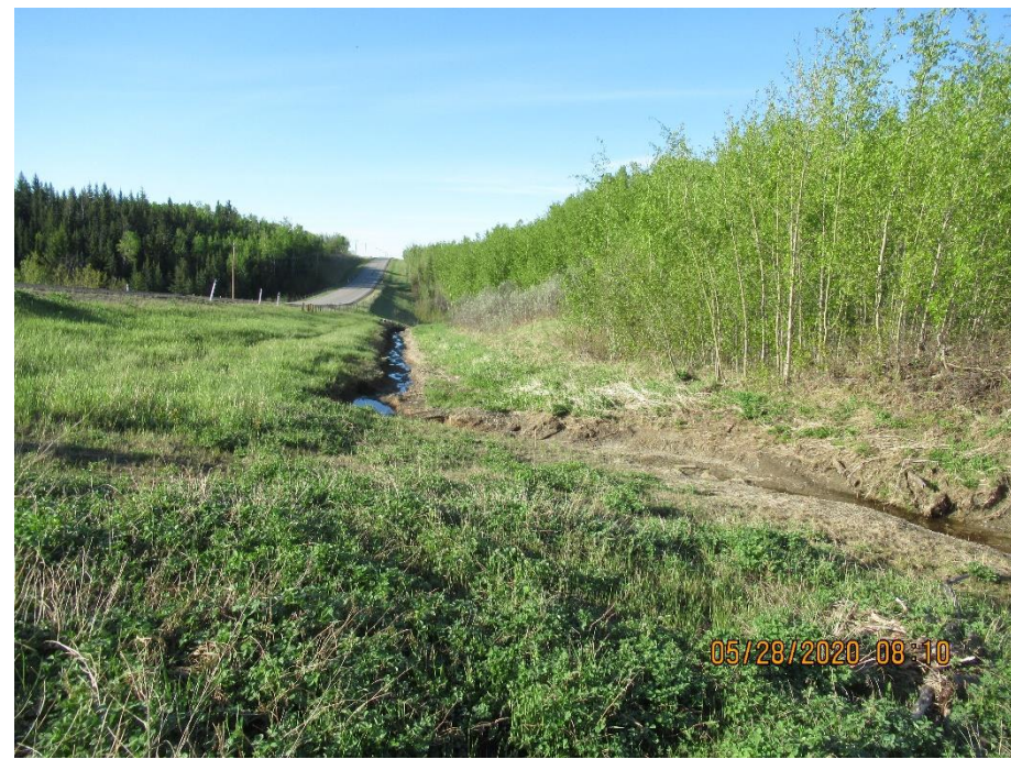
Photo 3. Looking south at eroded ditch along straw and coconut matting in west ditch.
