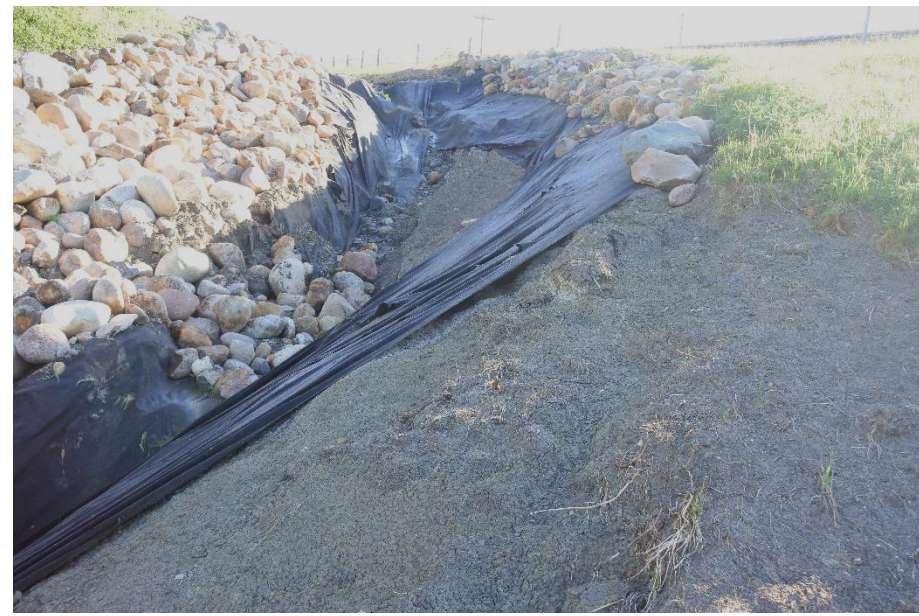
Photo 6. Looking north at reinforced swale that was constructed during the 2018 repair which has been eroded and the non-woven geotextile has been exposed.
