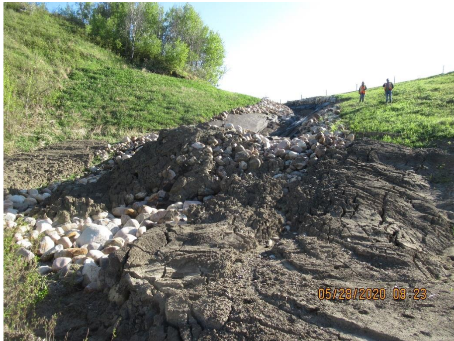
Photo 8. Looking northeast at the swale and debris accumulation near the toe of the embankment slope. The grassed area to the left was where the previous erosion gully had been filled in.
