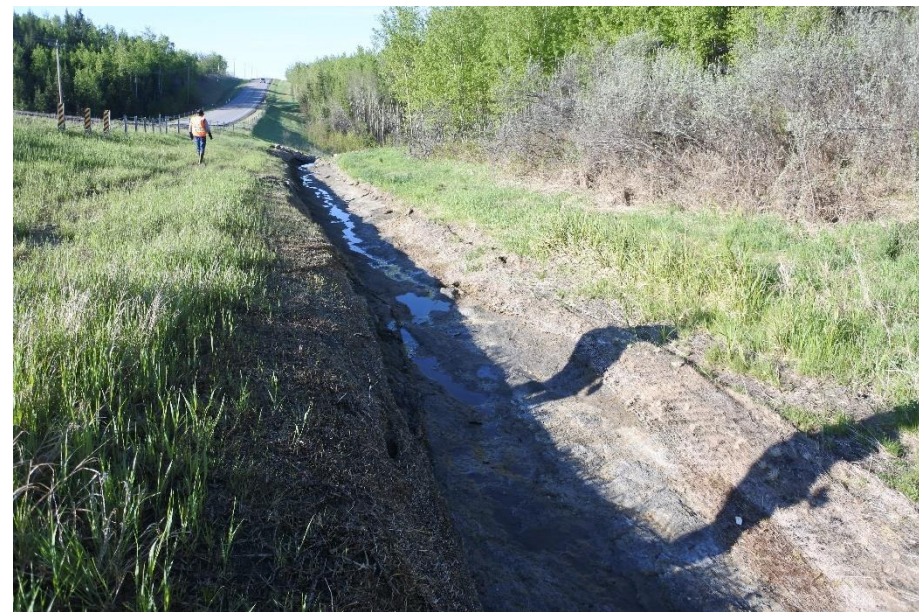
Photo 4. Looking south at erosion gully has undermined the straw and coconut matting in west ditch.
