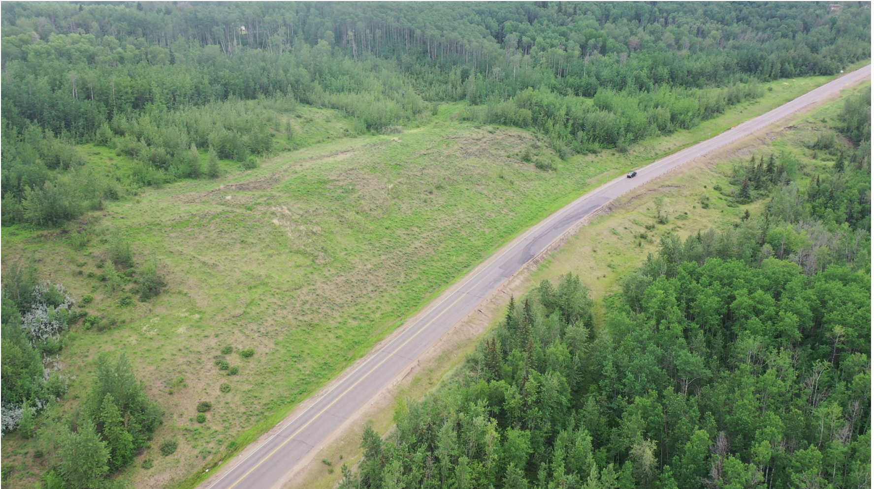
Photo 3 Overview of GP016-1 (upper) site. Note pavement patches, and cracking and settlement in westbound (north) lane of Hwy 666:02. As well as sliding along backslope and highway embankment (see next photo). Photo taken June 13, 2023, facing southwest.
