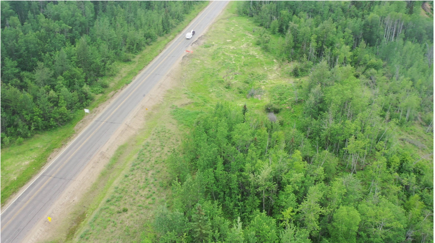
Photo 5 Overview of GP016-3 (upper) site. Note slide along shoulder of westbound (north) lane of Hwy 666:02. Photo taken June 13, 2023, facing southwest.
