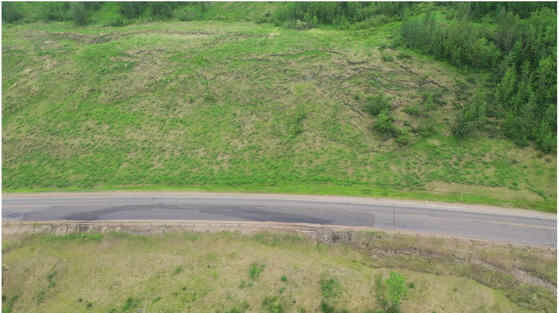
Photo 4 Cracking and settlement westbound (north) lane of Hwy 666:02 at GP016-1 (middle) site. Note cracking and toe rolls along backslope and highway embankment. Photo taken June 13, 2023, facing southeast.
