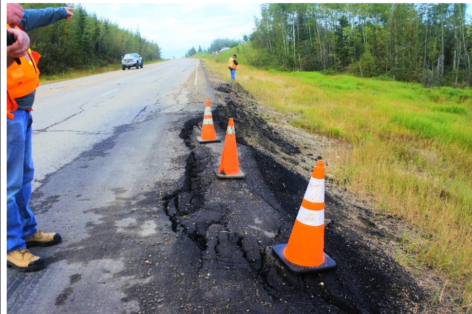
Photo 16. Looking southwest along backscarp in the west section of the Valley Top Landslide (Site 3). Site was patched in June 2019. Cracks extend 200 mm past the white line into the WBL, are open 220 mm and are 1 m deep.
