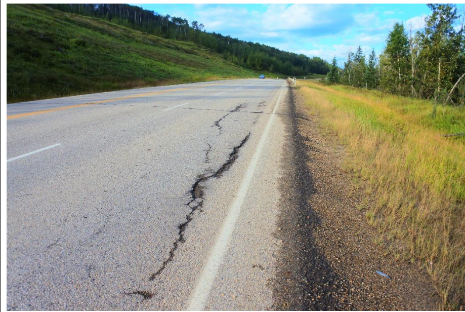
Photo 11. Looking southwest from the WBL shoulder at the slide in the backslope in the eastern portion of the Mid-Valley/"Old Major" Landslide (Site 1).
