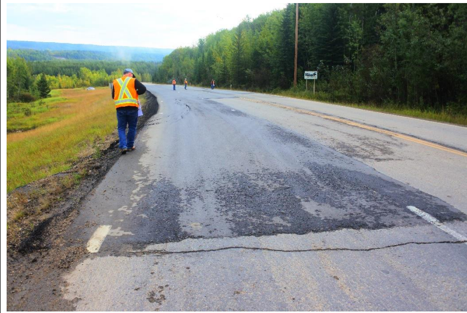
Photo 8. Looking northeast along cracks in pavement Lower Valley Landslide (Site 2).
