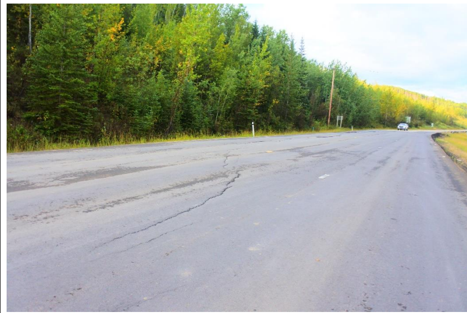
Photo 3. Looking southwest along Hwy 666 at west portion Lower Valley Landslide (Site 2). The drops along the scarp in the ACP in this section in the roadway surface were about 15 mm to 30 mm.
