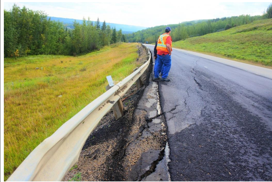
Photo 13. Looking northeast at graben below the highway at the Mid-Valley Landslide / “Old Major”(Site 1) and the cracking in the ACP in the WBL. The drop in the ACP along the backscarp near the guardrail at the west end is now at about 80 mm and the cracks are open to 80 mm.
