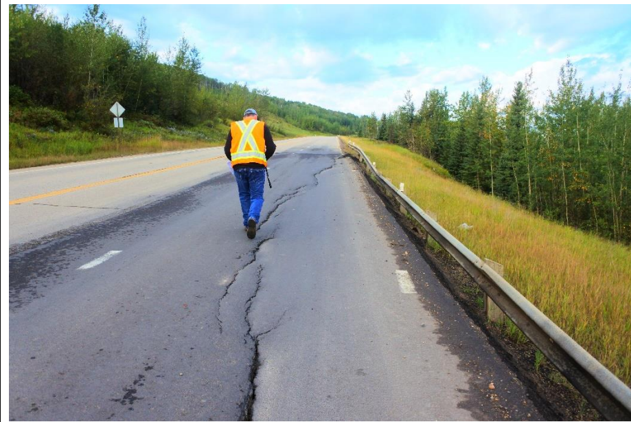
Photo 10. Looking southwest along WBL between the Lower Valley Landslide (Site 2) and the Mid-Valley/"Old Major" Landslide (Site1). Cracks drop from 50 mm to 120 mm along the scarp at the west end.
