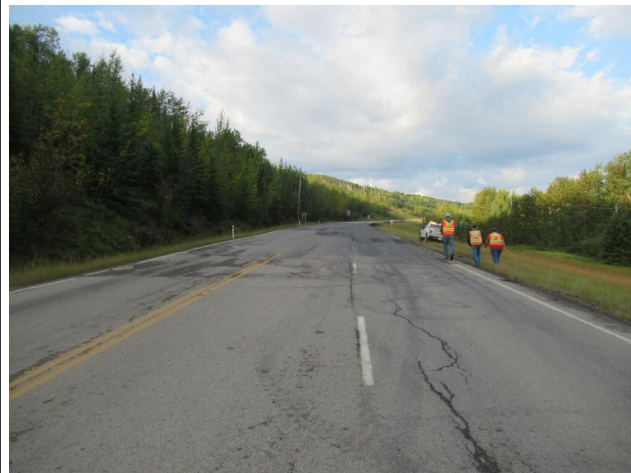
Photo 1. Looking southwest towards the Lower Valley Landslide (Site 2).
