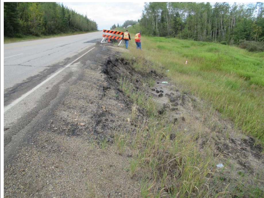
Photo 15. Looking southwest along backscarp of Valley Top Landslide (Site 3). Backscarp drop in embankment side slope now about 1.5 m
