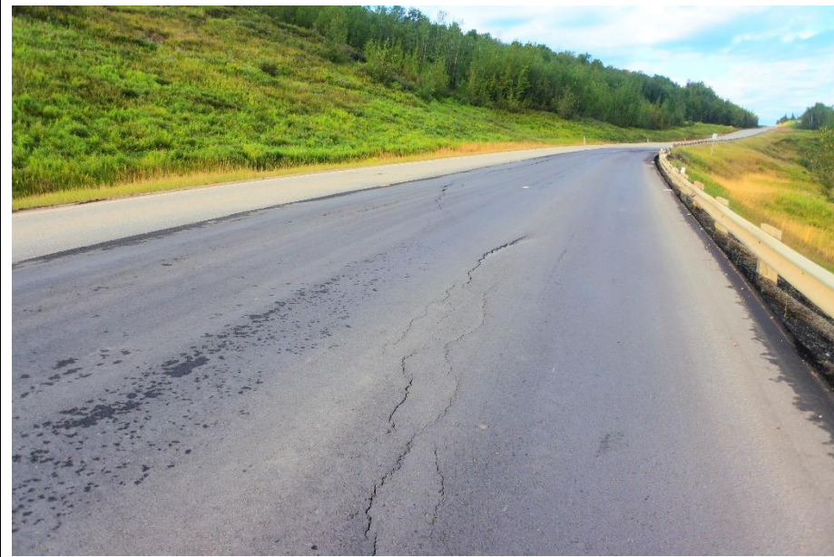
Photo 12. Looking west at the ACP patch in outer WBL at Mid-Valley/"Old Major" Landslide (Site 1). There is a 40 mm drop along the scarp in the ACP.
