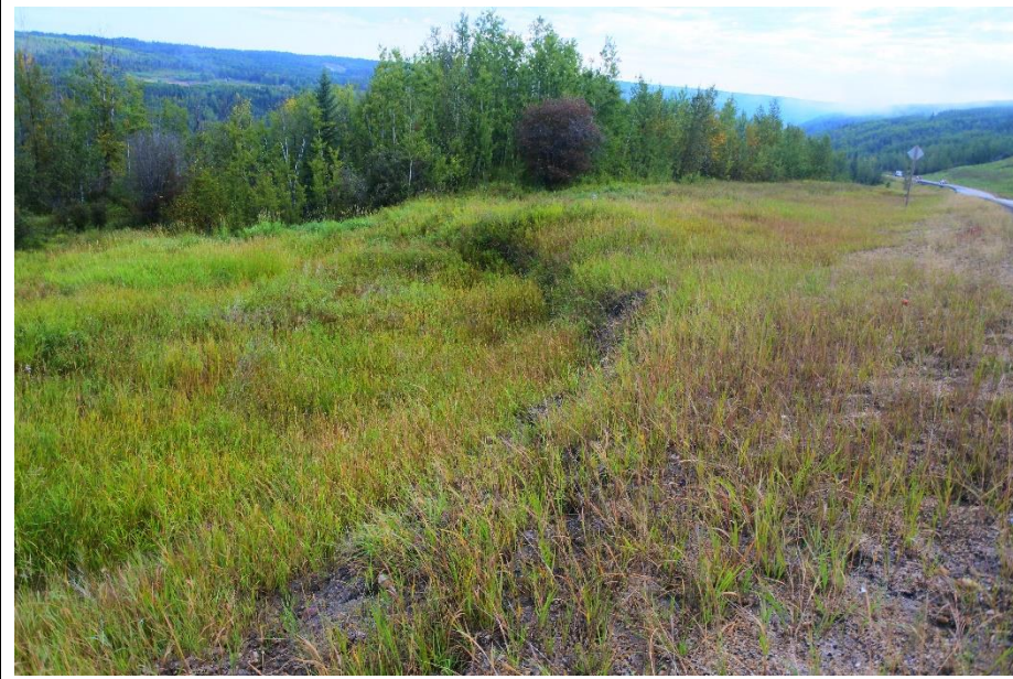
Photo 14. Looking northeast from the shoulder of the WBL at the scarp extending into the brush at the Valley Top Landslide (Site 3).
