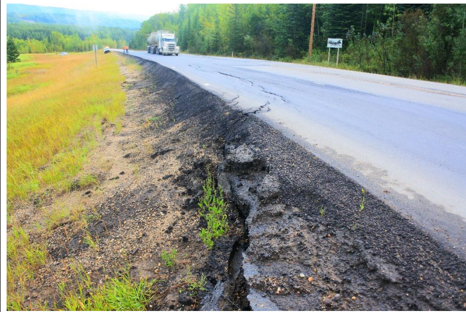
Photo 7. Looking northeast along cracks in pavement at Lower Valley Landslide (Site 2) that extend off the roadway.
