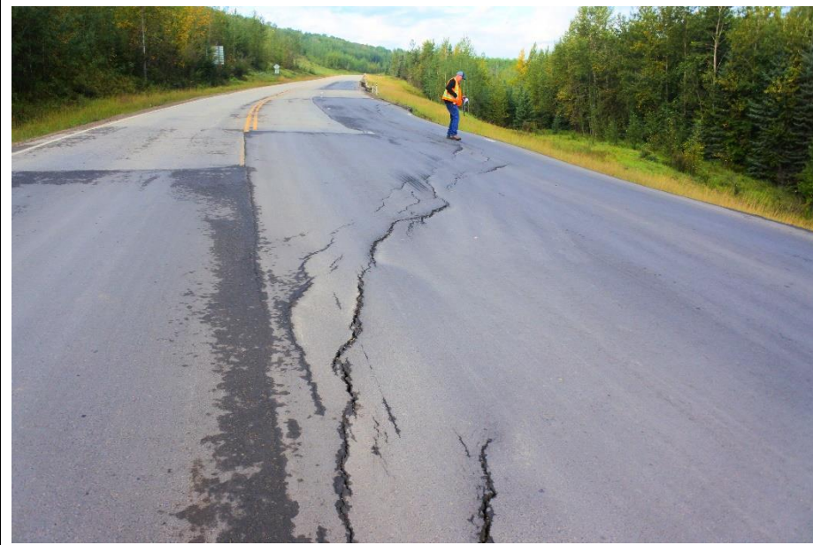
Photo 5. Looking southwest along Hwy 666 at west portion Lower Valley Landslide (Site 2). The scarp has a 0.3 m drop in the WBL shoulder.
