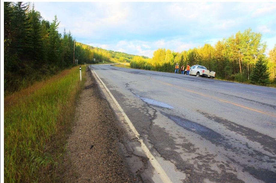
Photo 2. Looking southwest towards the Lower Valley Landslide (Site 2).
