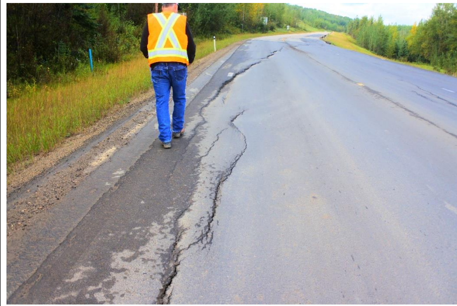
Photo 4. Looking southwest along Hwy 666 at middle portion Lower Valley Landslide (Site 2). The drop along the scarp in the ACP in this section in the roadway surface was up to about 70 mm
