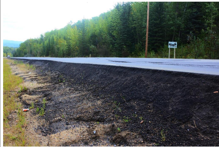
Photo 9. Looking east at overly steep drop off from several layers of ACP patching at Lower Valley Landslide (Site 2).
