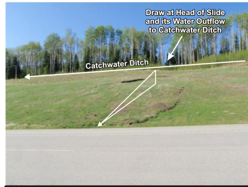
Photo 1 Looking east downgrade at backslope along eastbound lane • Slide located at below a catchwater ditch • Headscarp just below catchwater ditch • Toe bulge not affecting ditch yet
