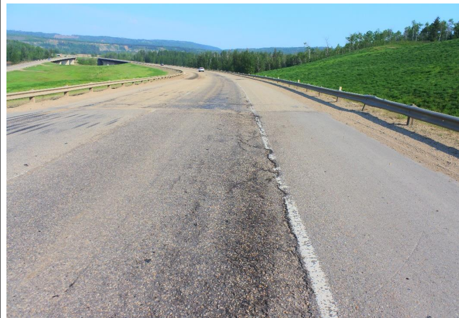
Photo 2. Looking northwest standing in right NBL looking at cracks and the dip.
