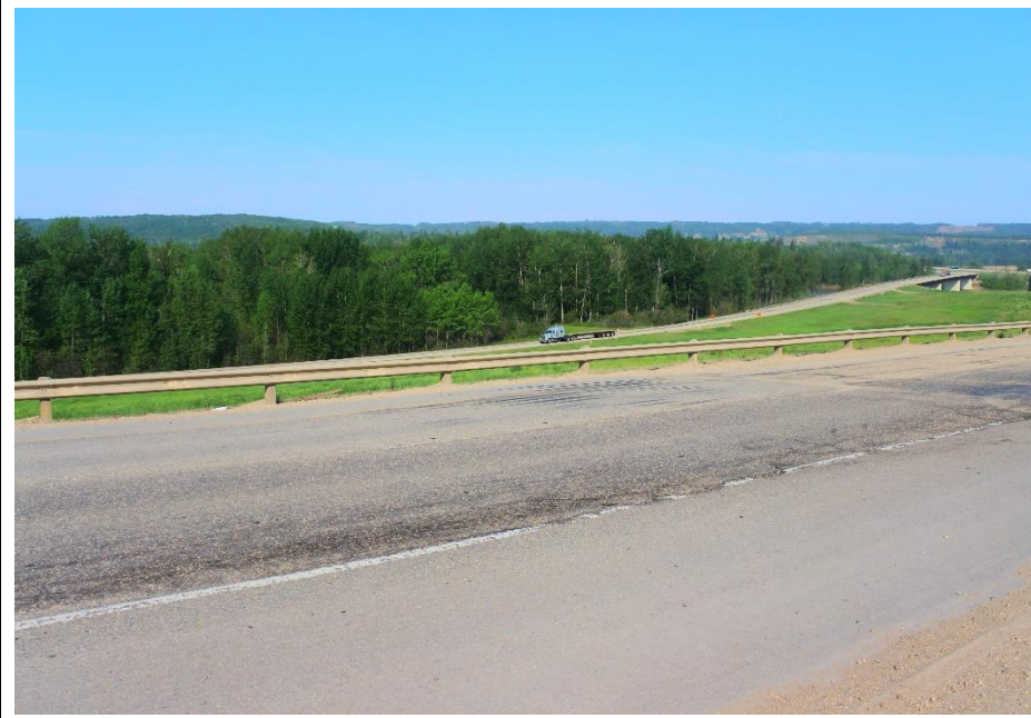
Photo 1. Looking northwest at dip in the pavement.
