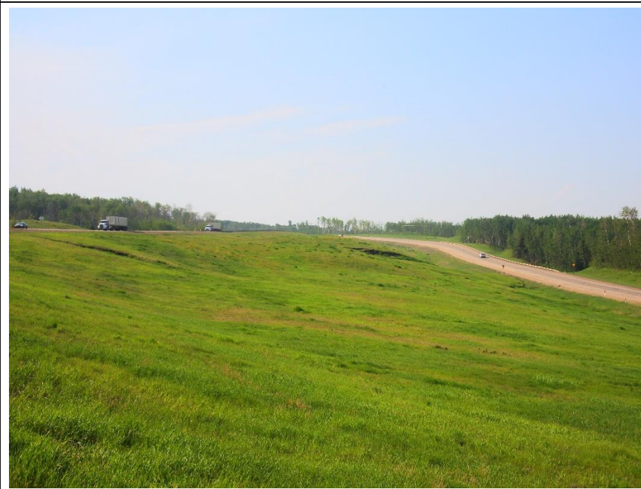
Photo 6. Looking southeast at GP 45 and eroded area 140 m east.
