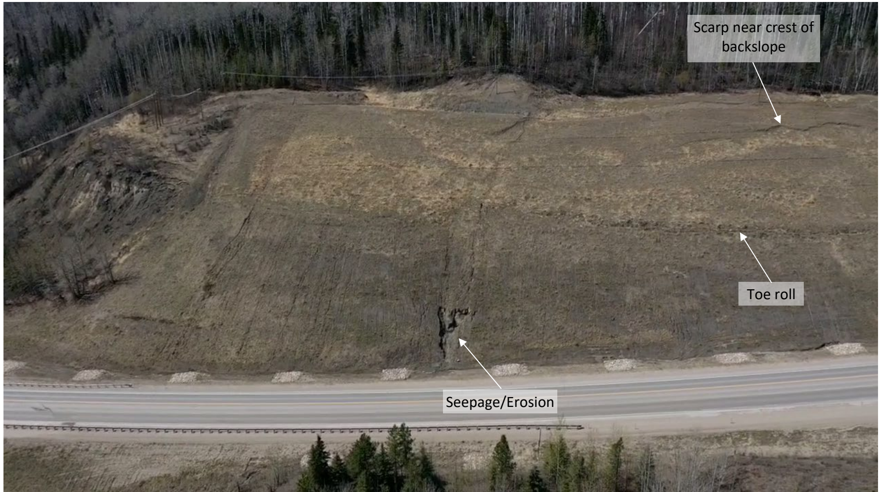
Photo 2 South end of GP044 site along backslope on west side of Hwy 40:40. Note rill and small gully erosion on backslope. Photo taken with UAV on May 9, 2024, facing west.
