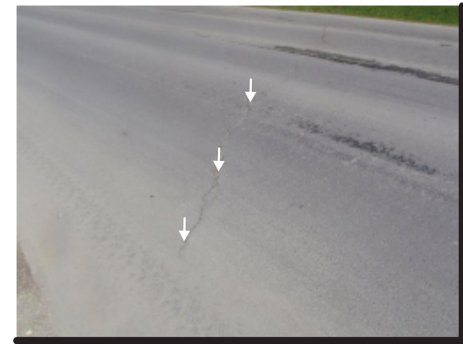
Photo 1a Cracks – Closeup
