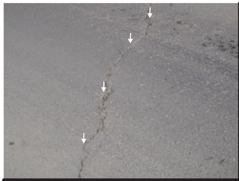
Photo 1b Cracks – Closeup
