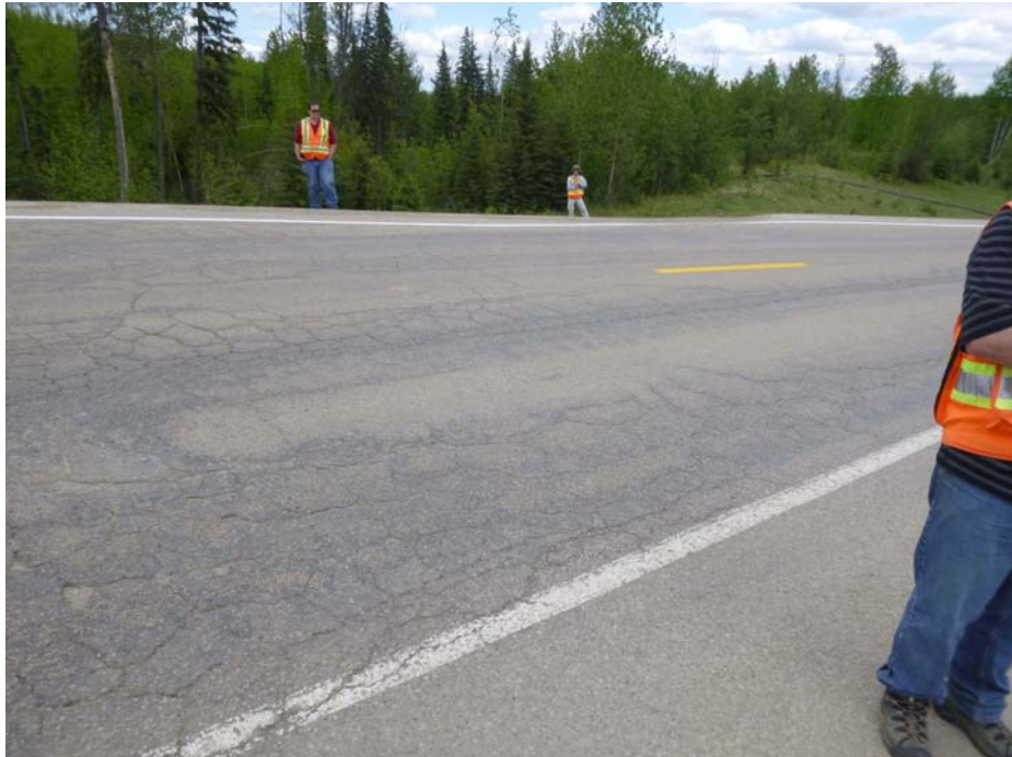
Photo 7 – Looking southeast at the alligator cracked pavement, and the dip in the east highway shoulder.
