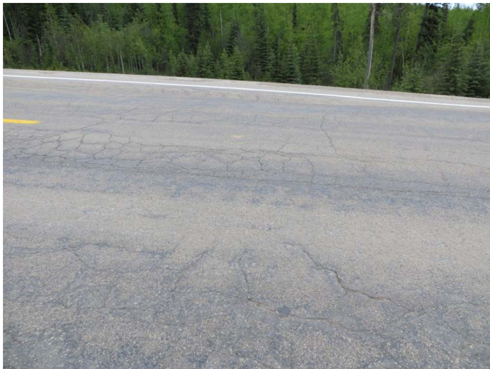
Photo 6 – Looking west across the alligator cracked pavement.
