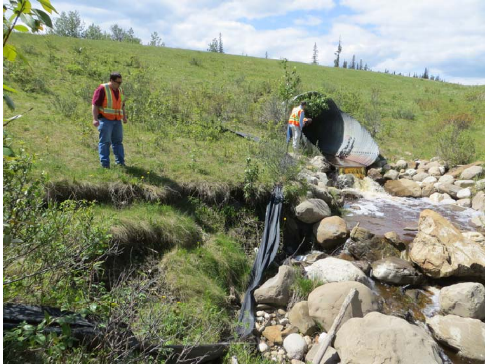
Photo 3 – Looking west at the 3 m diameter SPCSP outlet, plunge pool, and east highway embankment. Note the exposed woven geotextile adjacent to the slumped channel.
