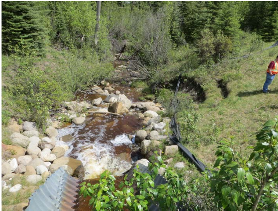
Photo 4 – Looking east at the culvert outlet and the riprap plunge pool. Note the slump scarp alongside the south channel edge.
