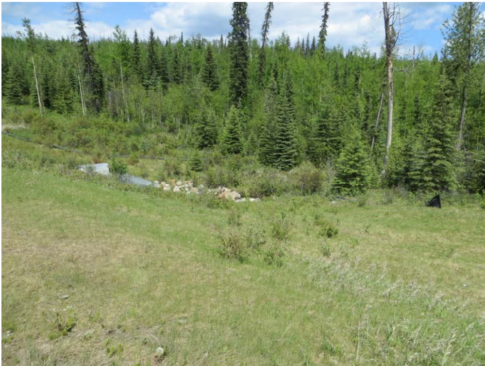
Photo 2 – Looking northeast across the east highway embankment, with the culvert outlet in the background.
