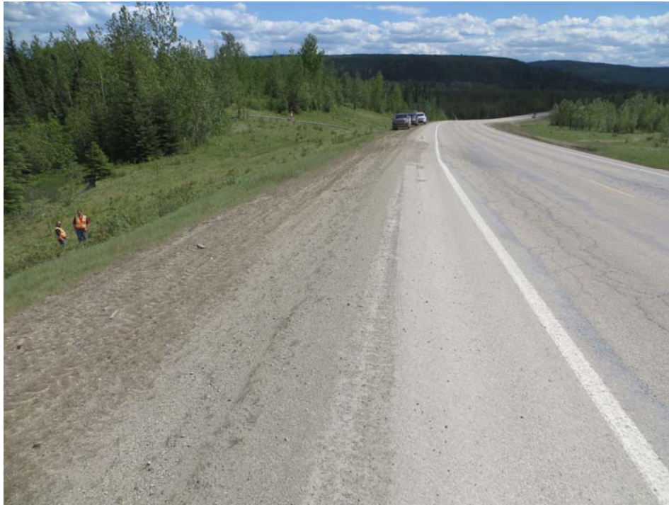
Photo 5 – Looking south along the east highway shoulder at the dip and scarp crack.
