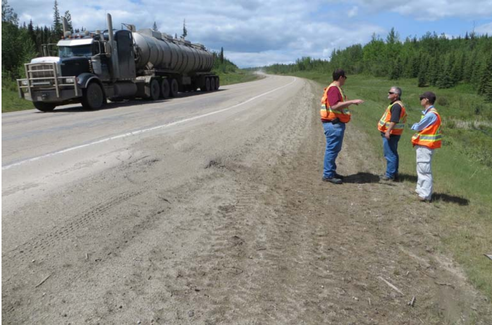
Photo 1 – Looking north along the east edge of the highway, at the dipped area. A slide scarp appears to be developing at this location.
