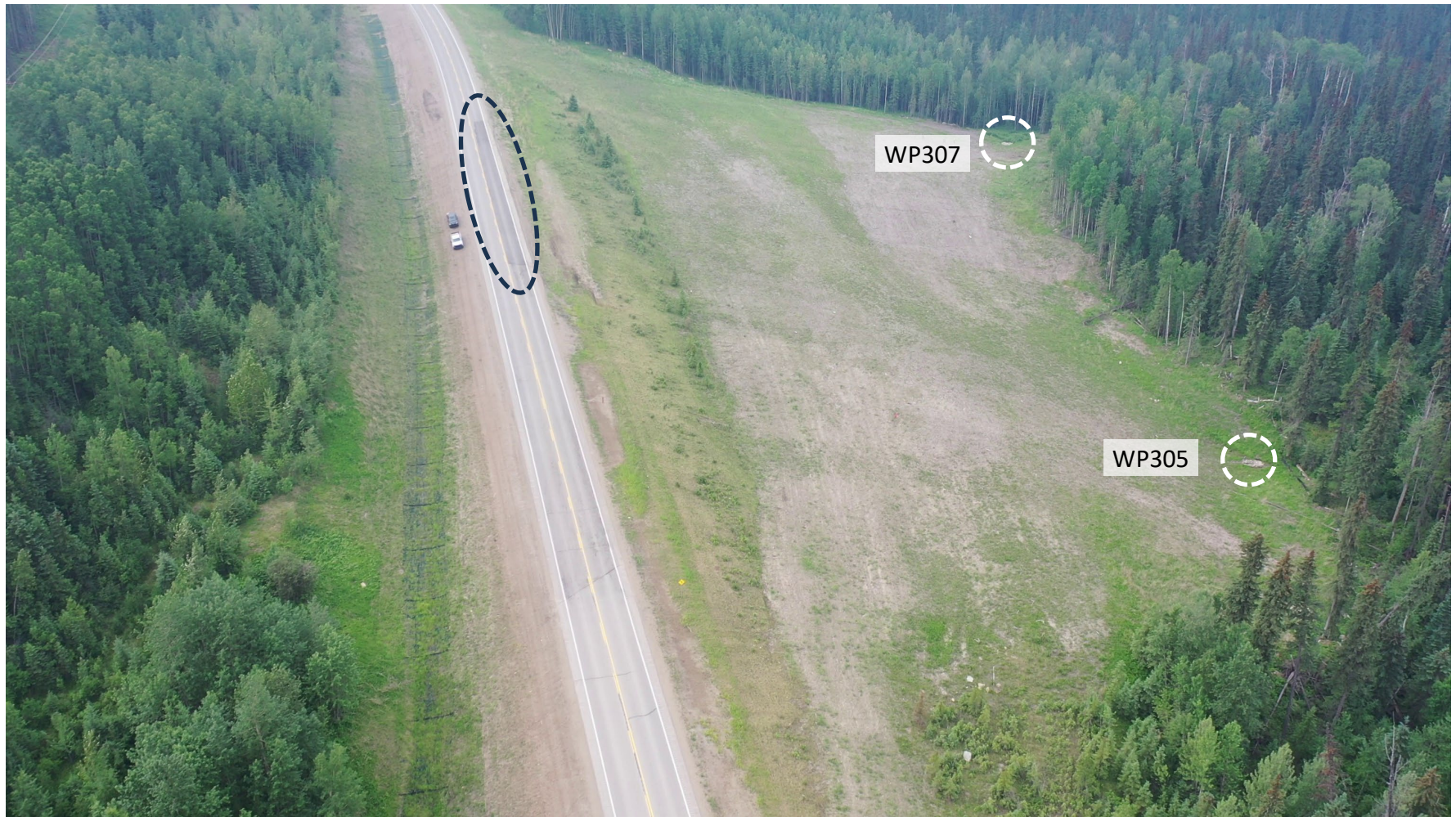
Photo 1 Overview of GP034 site. Note pavement patch placed after 2021 overlay in west (southbound) lane of Hwy 40:38 (circled in black) and drain outlets at WP305 and WP307 (circled in white). Photo taken June 13, 2023, facing southwest.
