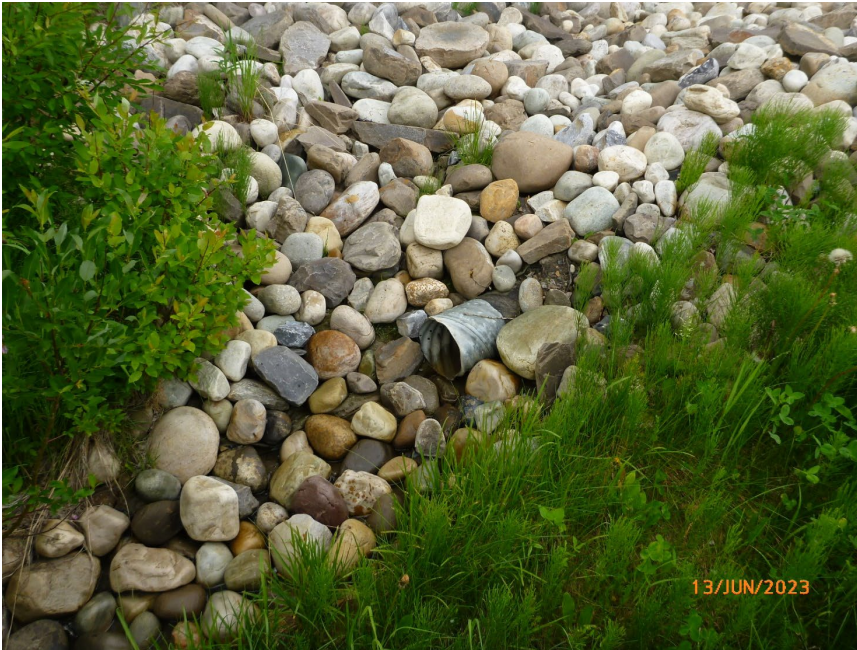
Photo 7 Flowing drain outlet in east (northbound) ditch of Hwy 40:38 at WP308. Photo taken June 13, 2023, facing southeast.
