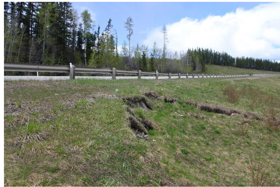
Photo 4. Looking northwest at backscarp nearing the highway.
