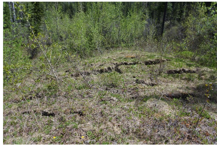
Photo 7. Looking southeast at open tension cracks that were filled with water.
