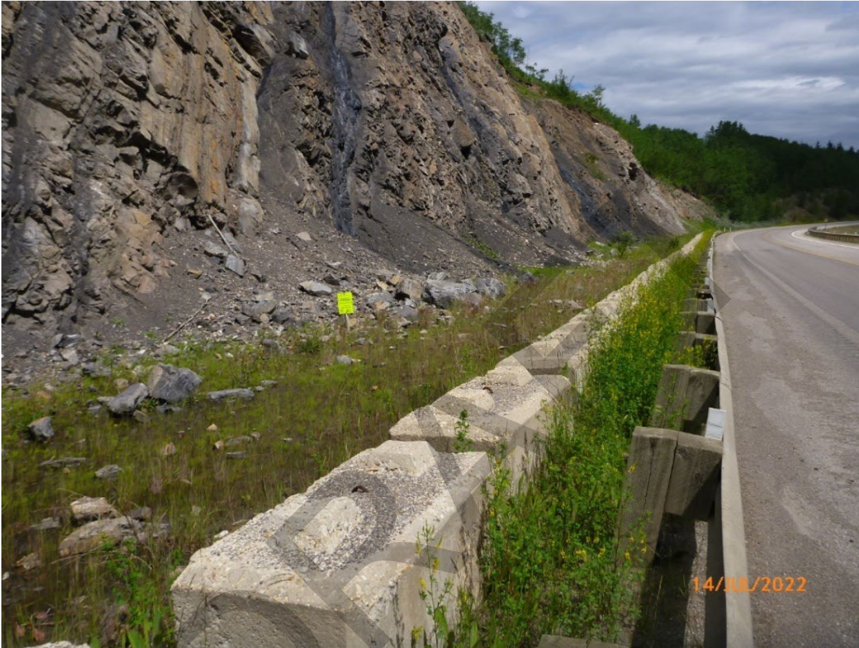
Photo GP036 – 9 Portion of slope with deteriorating lock blocks and guard rail at edge of pavement. Note weathering coal seams, rockfall particles in ditch, and pipeline marker at toe of slope. Photo taken July 14, 2022, facing northeast.
