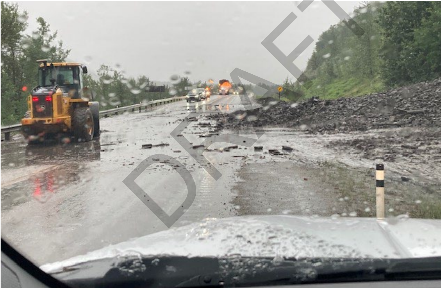
Photo 1 Debris being cleared from highway by front-end loader. Photo taken by Highway Maintenance Contractor (MCI) on June 19, 2023, facing south.
