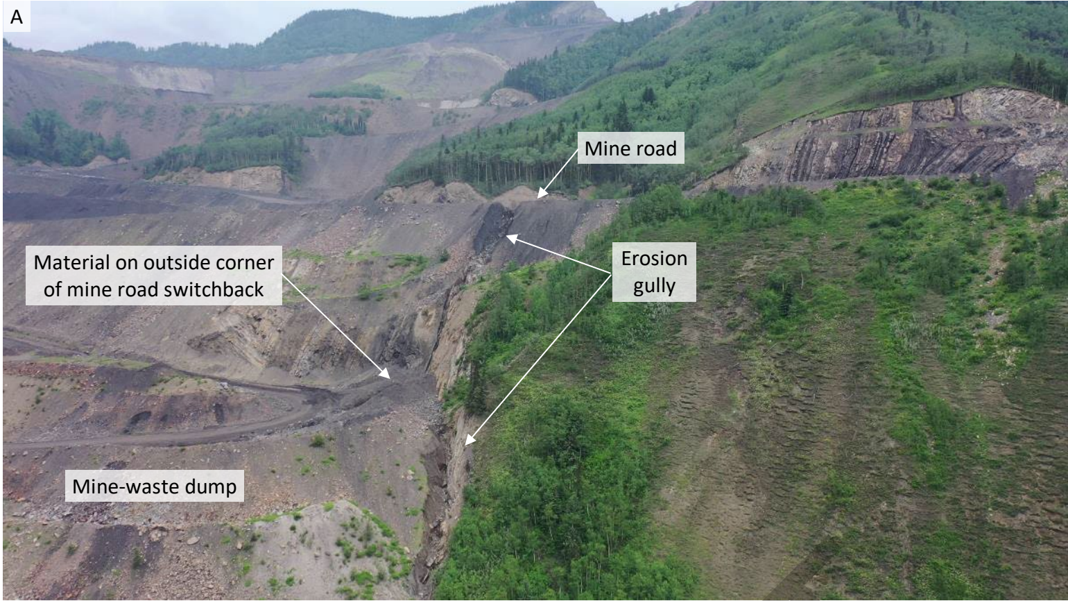
Photo 4 Overview of site. Note erosion gully between north flank and toe of mine-waste dump through some material located on outside corner of mine road switchback, below rockfall fence, and through lower mine road. Also note water flowing from water ponded at northeast corner of waste-rock dump and along highway backslope (indicated with blue arrows), and stockpile of debris material along west highway ditch. Photo taken with UAV on June 22, 2023 facing west and down.
