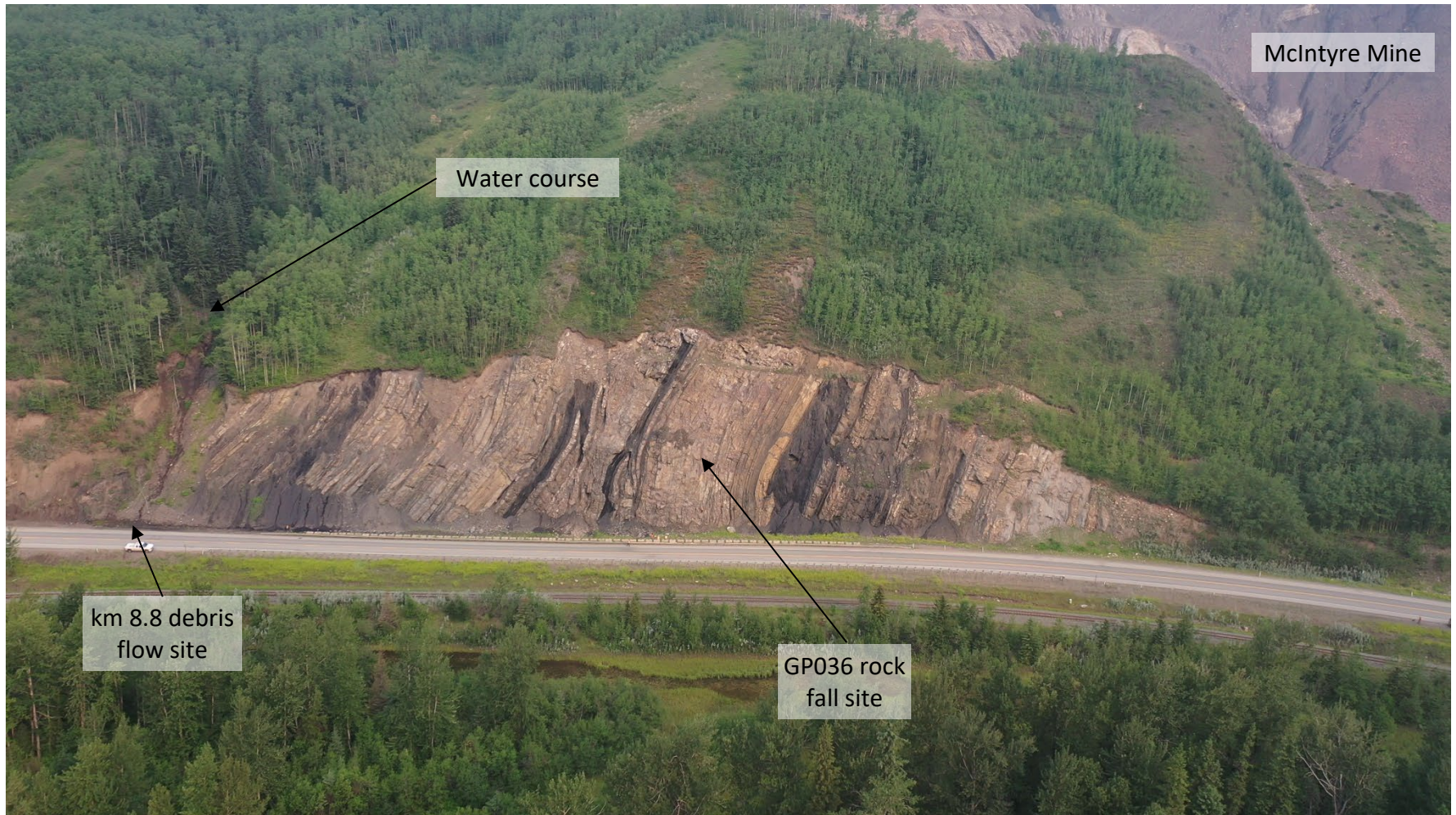
Photo 4 Debris flow location (km 8.8) along backslope on west side of Hwy 40:36. Note water course above debris flow locations. Photo taken June 14, 2022, facing west.
