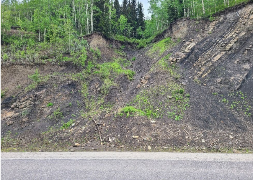
Photo 9 Debris flow at km 12.1 along backslope on west side of Hwy 40:36 just south of GP036 site and WP189. Note erosion gully down debris fan. Photo taken June 14, 2022, facing west.
