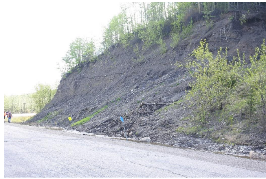
Photo 8. Hwy 40:36 km 10.9 Looking west from the shoulder of the NBL shoulder of Hwy 40:36 at slide mass now within the SBL ditch.
