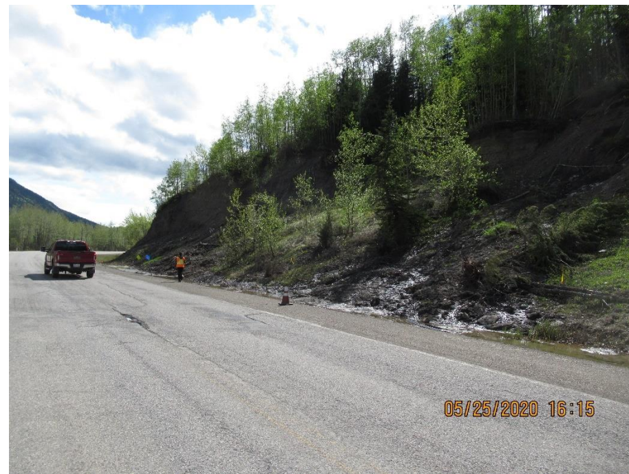
Photo 9. Hwy 40:36 km 10.9 Looking southwest from the near the middle of the Hwy at slide mass.
