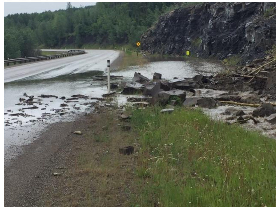
Photo 5. Hwy 40:36 km 8.5 Looking southwest from the shoulder of the EBL of Hwy 40:36 taken by AT on June 14, 2020.
