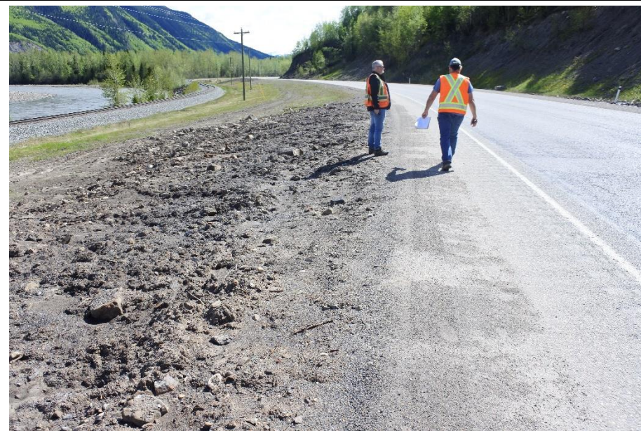
Photo 10. Hwy 40:36 km 10.9 Looking south from the shoulder of the NBL shoulder of Hwy 40:36 where slide debris previously flowed across the highway.
