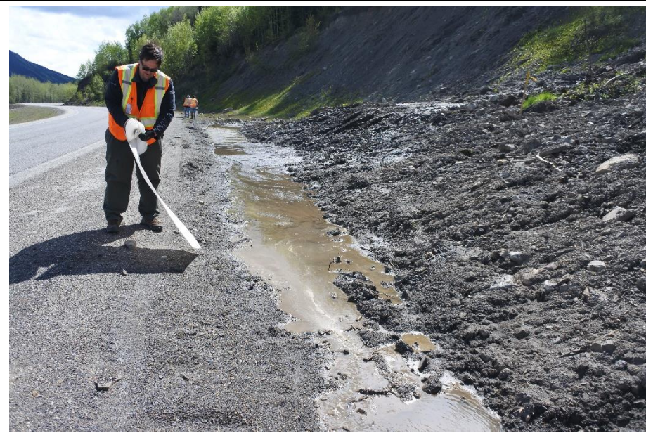
Photo 12. Hwy 40:36 km 11.2 Looking south from the shoulder of the SBL shoulder of Hwy 40:36 debris in ditch and water flowing around debris along highway shoulder.
