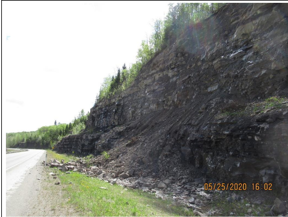
Photo 3. Hwy 40:36 km 8.5 Looking southwest at the backslope face just to the south of Photo 1. Note that there are a couple of smaller zones of recent rockfalls west of the large one.
