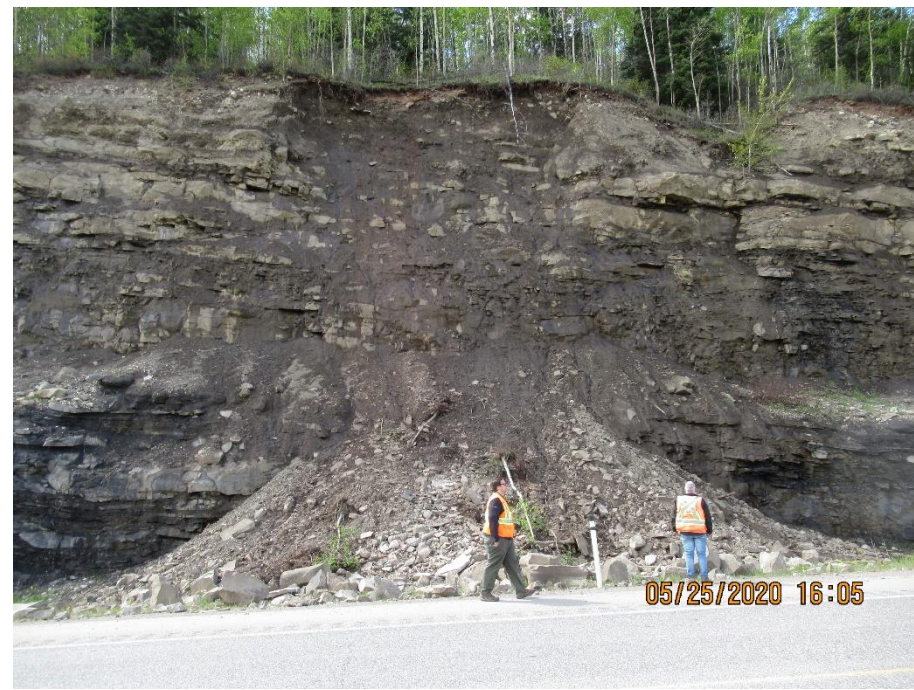
Photo 1. Hwy 40:36 km 8.5 Looking directly at the face of the west hwy rock backslope and overburden/rock fall deposit in the west ditch.
