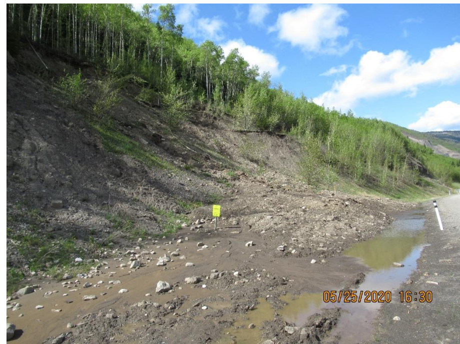
Photo 15. Hwy 40:36 km 11.2 Looking northwest from SBL shoulder at slide mass.
