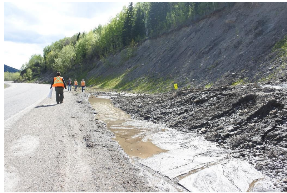
Photo 13. Hwy 40:36 km 11.2 Looking southwest at debris which has slid down into ditch and water is now flowing around it.
