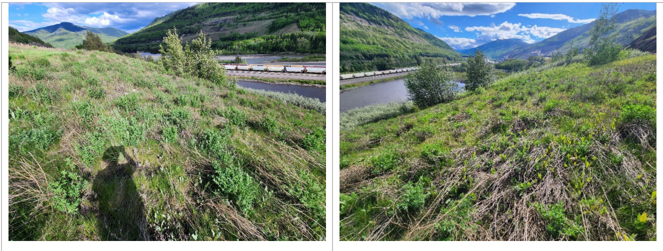
Photo 4 Slope on south side of Hwy 40:36 at middle slide area. Photos taken June 10, 2024, facing southeast and southwest, respectively.
