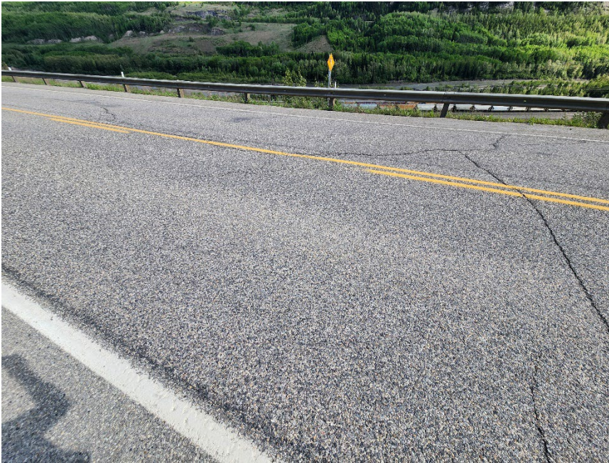
Photo 3 Cracking and dip in pavement surface of Hwy 40:36 at middle slide area. Photo taken June 10, 2024, facing southeast.
