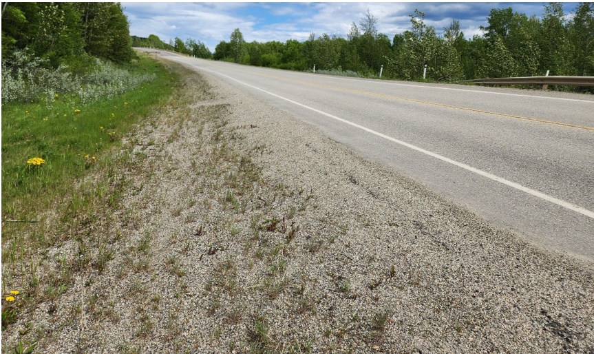
Photo 6 Cracking and settlement across Hwy 40:36 near west end of recent pavement patch at east end of GP007 site. Photos taken June 10, 2024, facing southeast and southwest, respectively.
