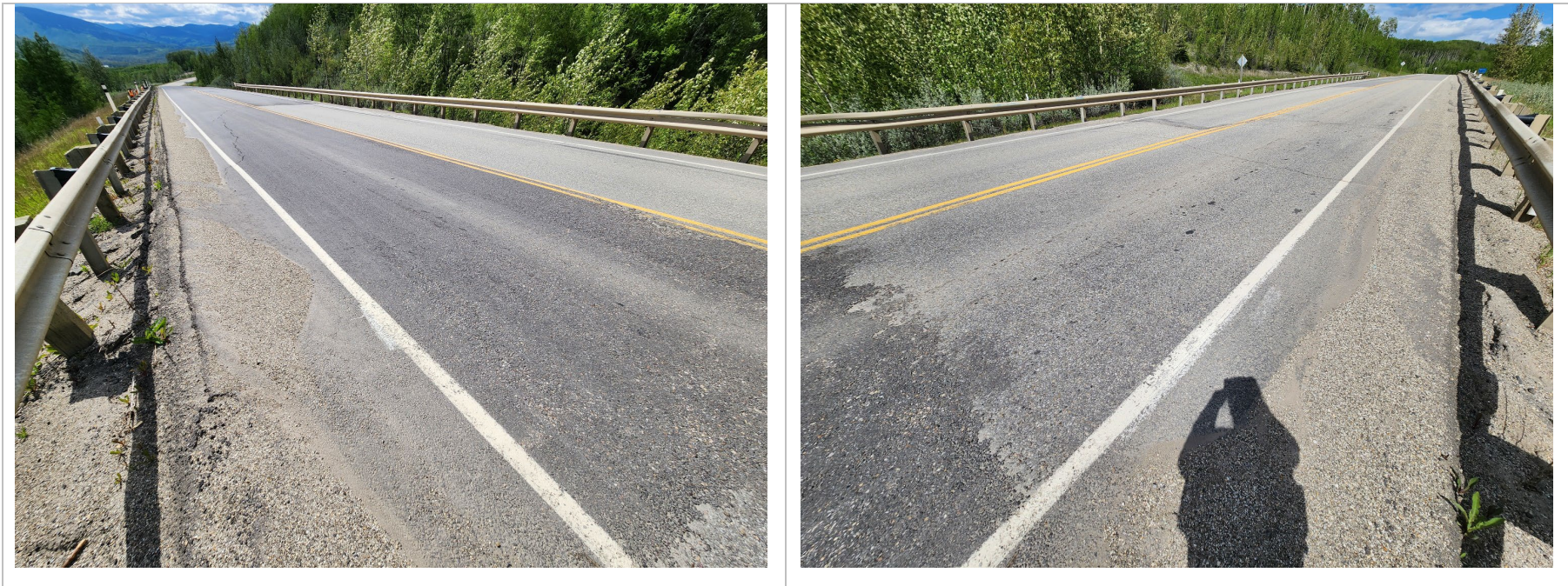
Photo 9 Guardrail on south side of highway at east end of site is low and located far from highway. Photo taken June 10, 2024, facing east.
