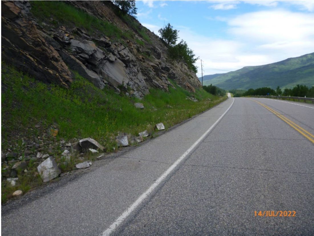
Photo GP053-II – 7 Talus slopes and rock blocks in the ditch. The rock blocks in the ditch appear to get closest to the highway by rolling down the talus slope. Photo taken July 14, 2022, facing northeast.
