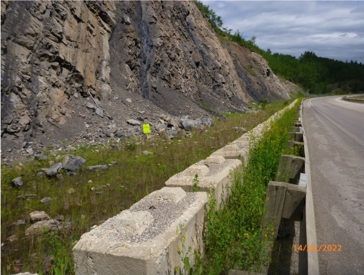
Photo GP036 – 9 Portion of slope with deteriorating lock blocks and guard rail at edge of pavement. Note weathering coal seams, rockfall particles in ditch, and pipeline marker at toe of slope. Photo taken July 14, 2022, facing northeast.
