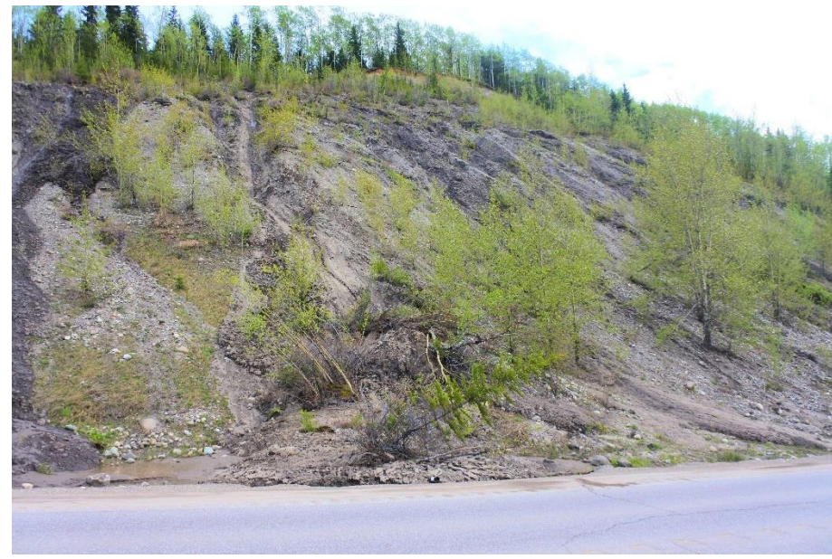
Photo 2. Looking south at shallow landslides/mudslide s and accumulation of debris near base with trees still growing on mass that slid.
