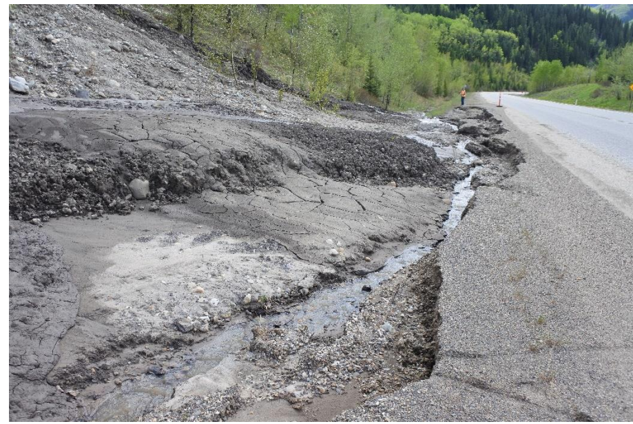
Photo 6. Looking southwest at east ditch further downslope at erosion cutting into the highway shoulder.
