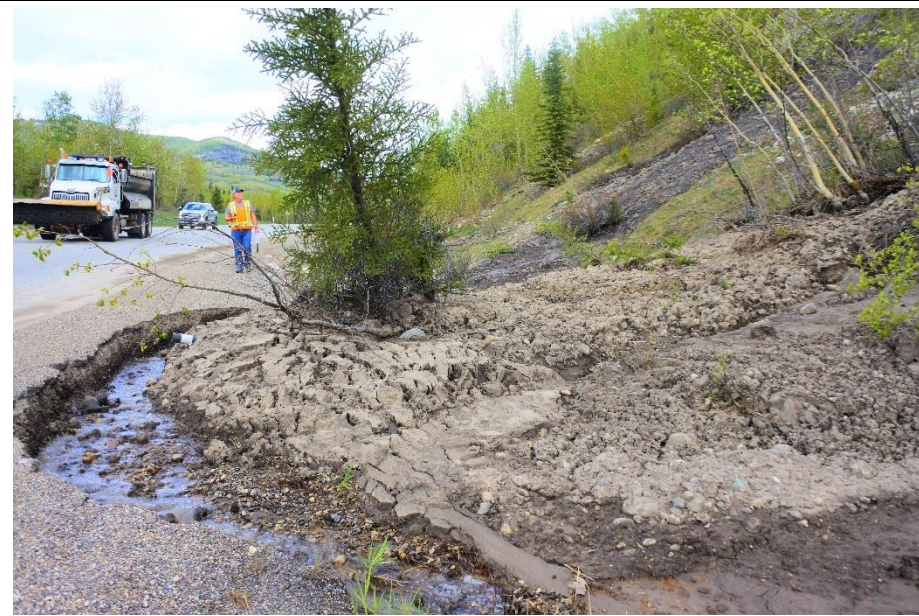
Photo 4. Looking northeast at debris which slid down into east ditch and erosion is cutting it's way down around it.
