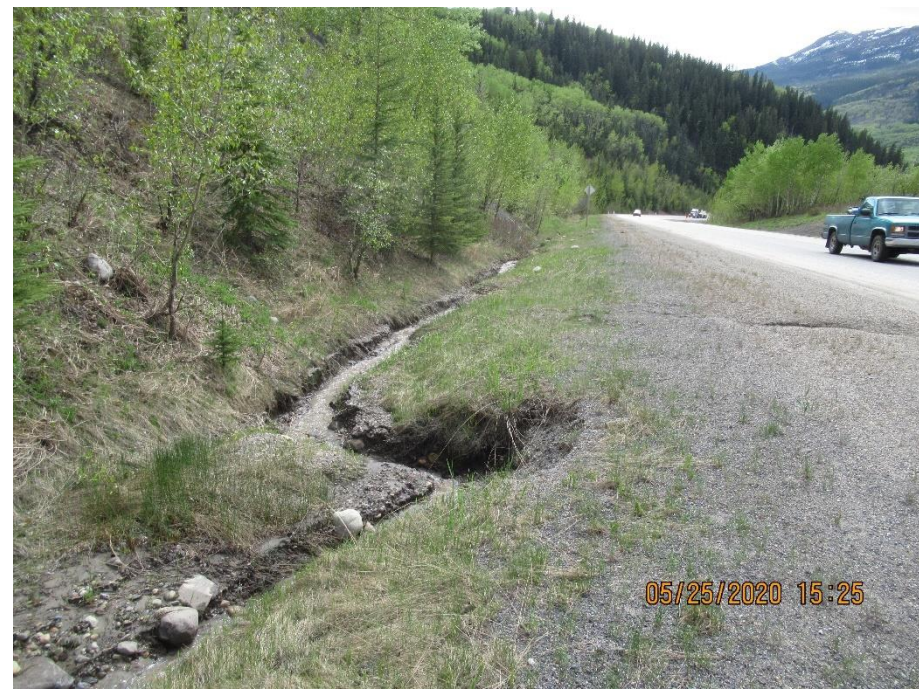
Photo 9. Looking southwest at east ditch at the southmost portion of the site erosion.
