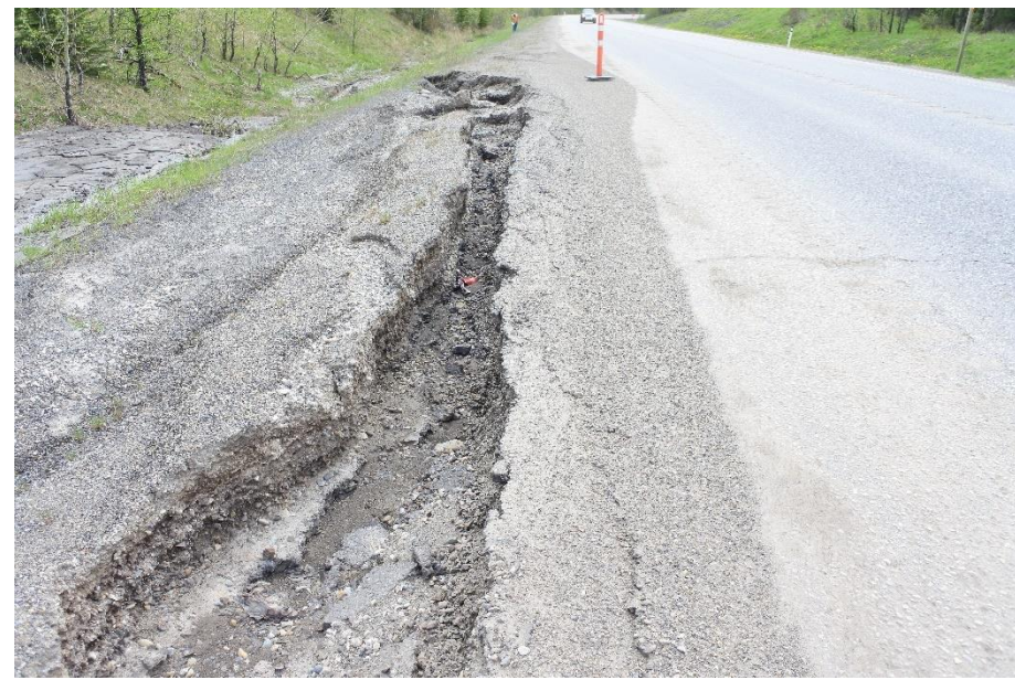
Photo 7. Looking southwest at east ditch further downslope at erosion cutting into the highway shoulder.
