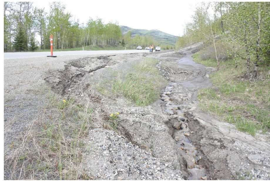
Photo 8. Looking northeast at east ditch further downslope at erosion cutting into the highway shoulder and delineator has been placed.
