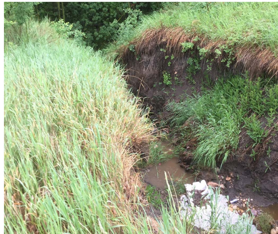
Photo 6. Looking southwest from the crest of the Culquhoun Creek north valley slope along the erosion gully. Some additional erosion and retrogression has occurred since 2014.
