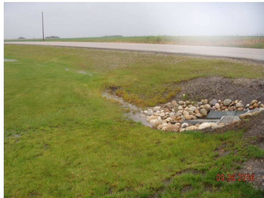
Photo 1. Looking northeast from the private driveway at 130028 Hwy 724 to the inlet of double barreled 900 mm CSP culverts in the SBL ditch.
