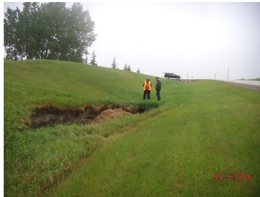
Photo 5. Looking northwest from the sideslope of the SBL of Hwy 724:04 at erosion gully that has formed at the crest of the Culquhoun Creek north valley slope.
