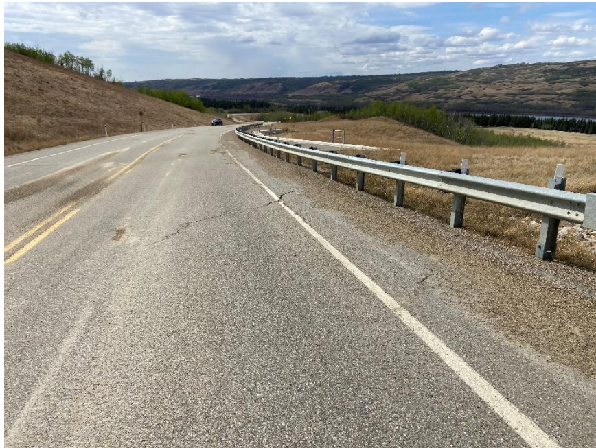
Photo 4. Looking west at diagonal cracks in road pavement.
