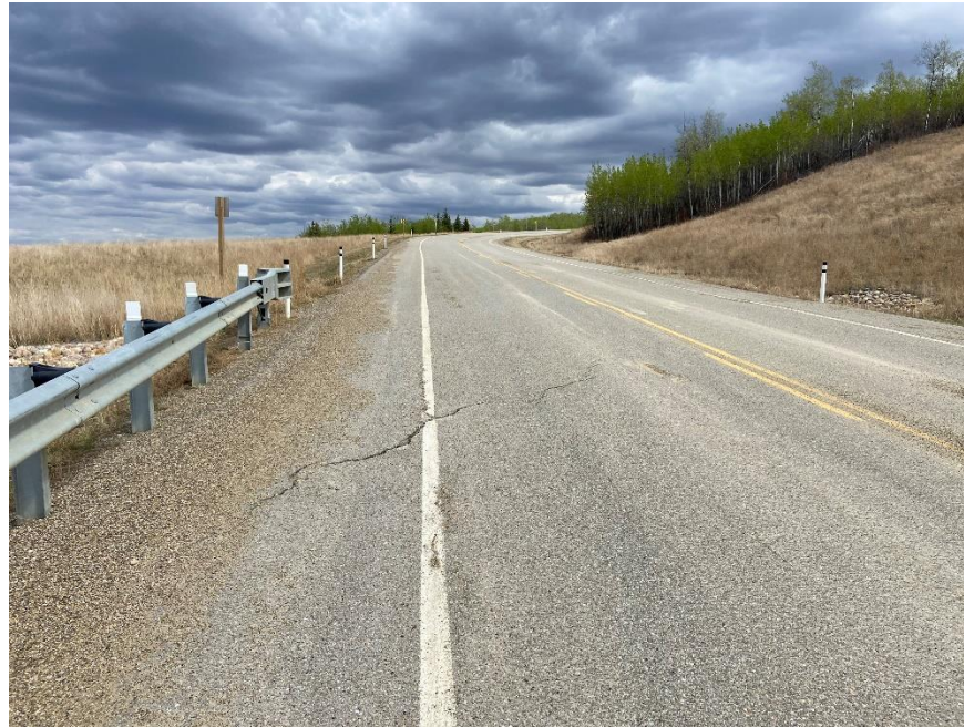
Photo 5a. Looking southeast at diagonal cracks in road pavement.
