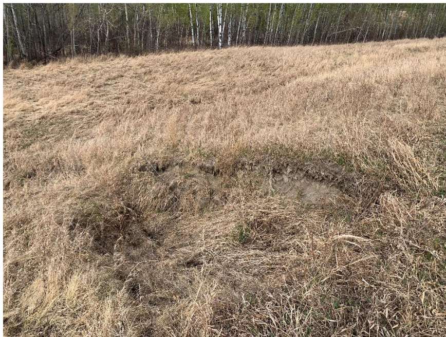
Photo 14. Looking north at eroded/slumping outlet of centreline culvert
