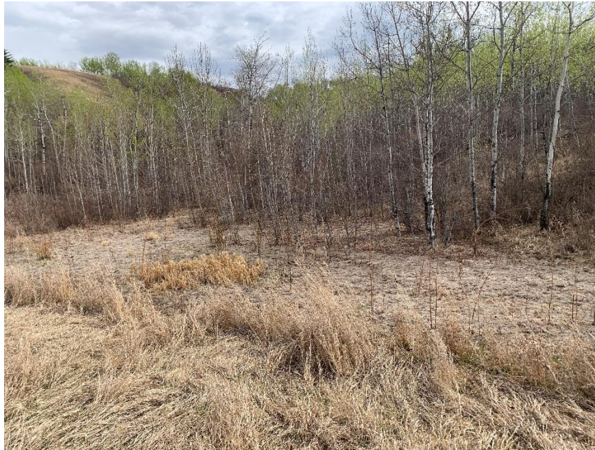
Photo 15. Looking south at the silted-up inlet area of the centreline culvert near Sta. 49+460.
