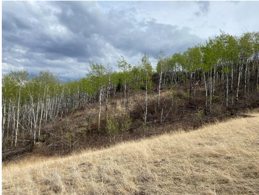
Photo 11. Looking southeast at the active landslide in the bush east of the toe berm.
