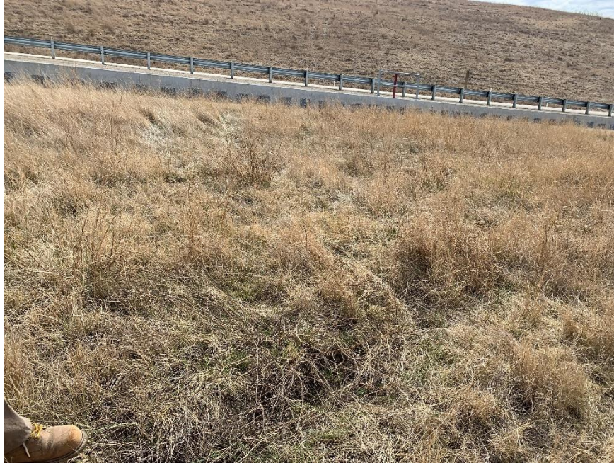
Photo 3. Looking at landslide backscarp crack downslope of pile wall.
