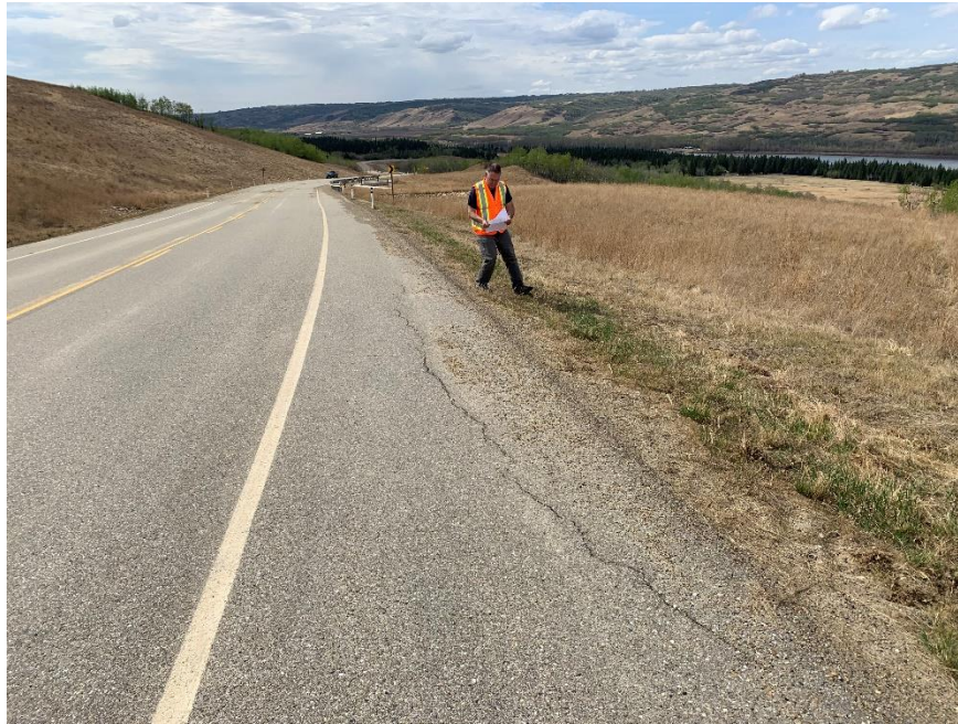
Photo 13. Looking west at arc shaped cracks in highway shoulder.
