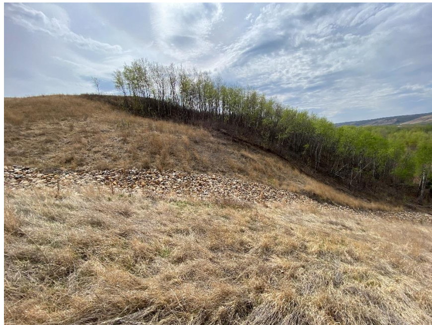
Photo 8. Looking west at slump in cut slope. It hasn't changed since the last inspection.
