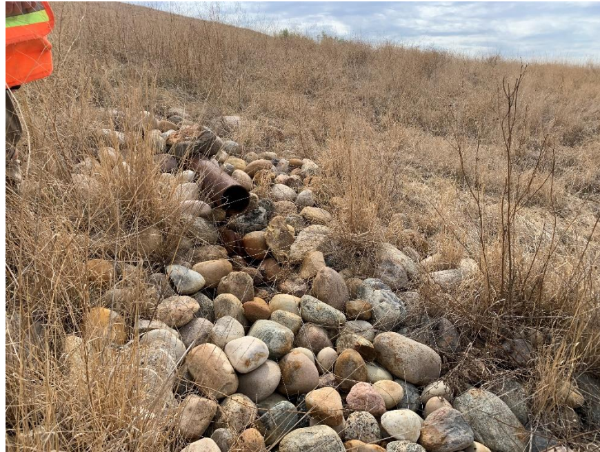
Photo 7. Looking at steady drip from drain pipe.
