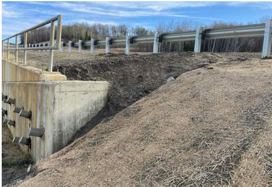
Photo 6 – Looking north at the south end of the pile wall at Site 3. If runoff begins to develop at this area, it will need to be built up with additional clay infill, then topsoiled/seeded/covered.
