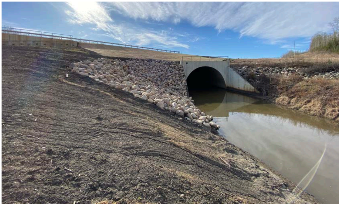
Photo 4 – Looking southeast at the slide repairs and the arch culvert outlet area at Site 3.
