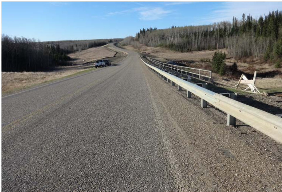
Photo 10 – Looking south along the highway from the north end of the pile wall of Site 3.
