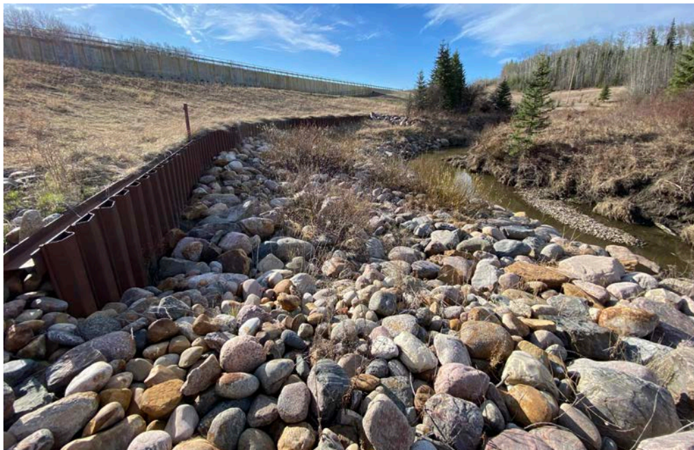
Photo 8 – Looking south along the lower pile wall, riprap, and river at Site 3.
