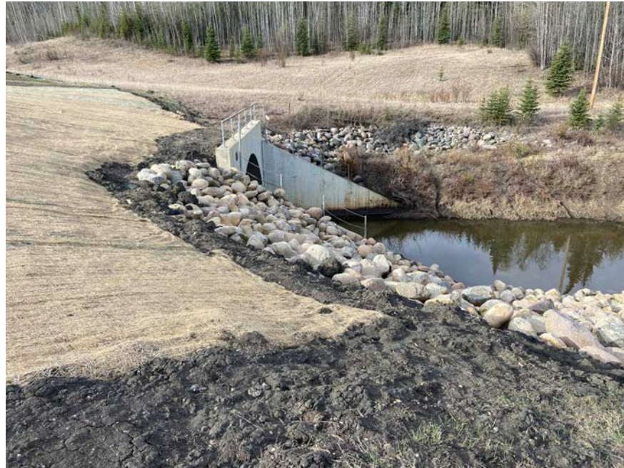
Photo 3 – Looking southwest at the lower slide repairs and arch culvert at Site 3.
