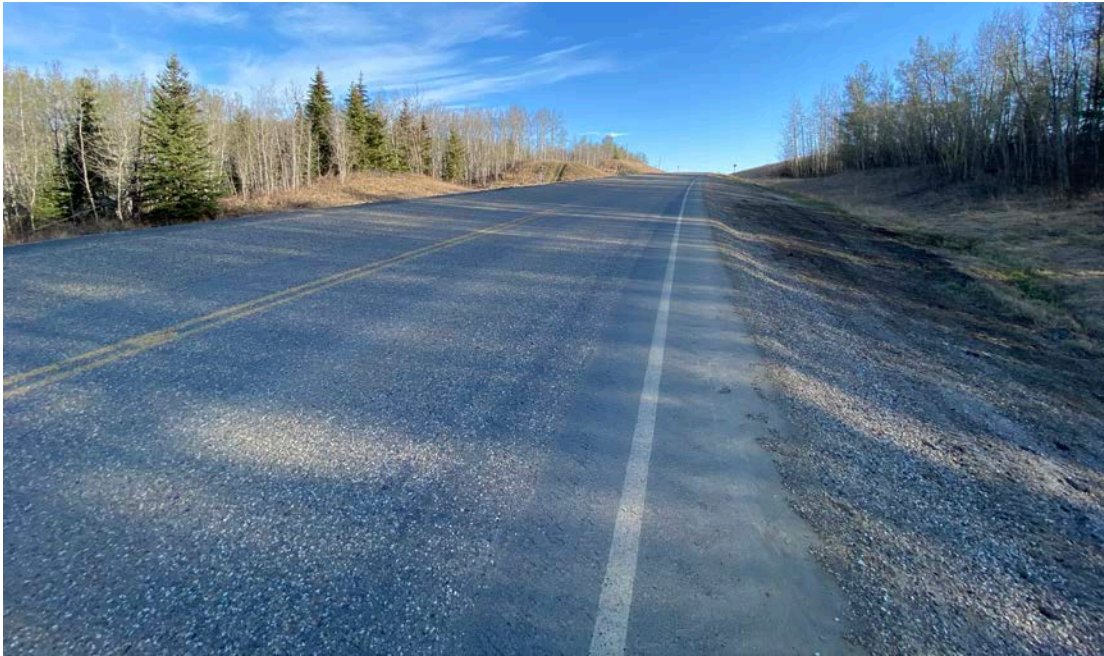
Photo 13 - Looking north along the east highway edge where the slide scarp crosses the highway at Site 6.
