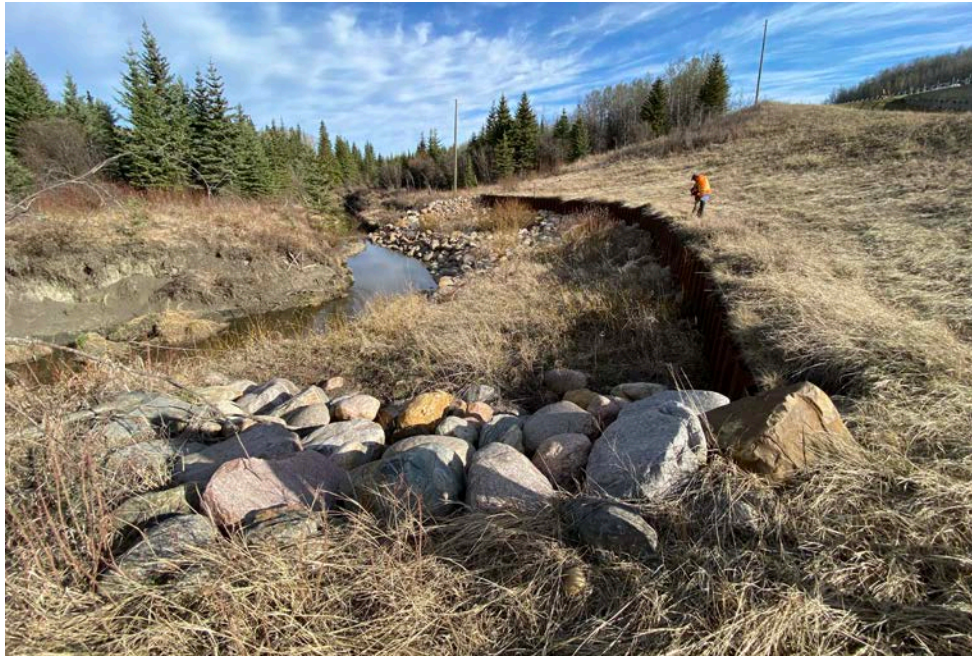
Photo 7 – Looking north at the lower pile wall area at Site 3, the riprap behind it, and the river.
