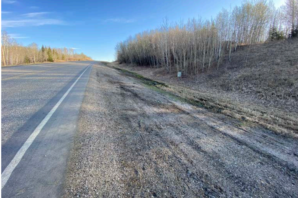
Photo 11 - Looking north along the highway and east ditch from the south end of the scarp of Site 5.
