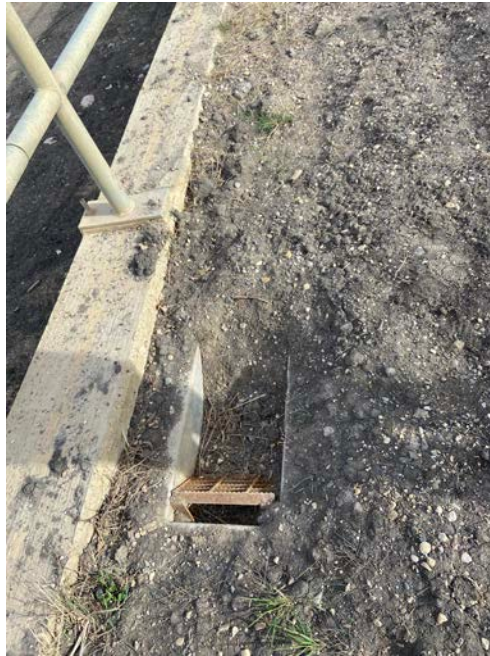
Photo 5 – Looking north at the top of pile wall gutter drain and loose cover plate at site 3. This needs to be cleaned.
