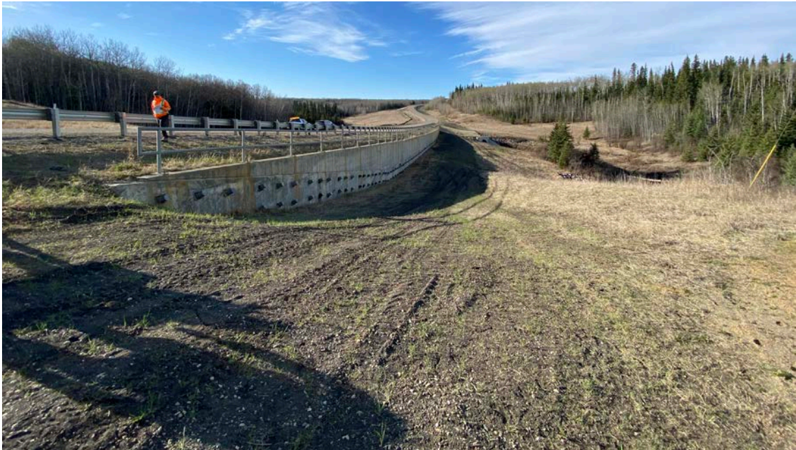
Photo 9 - Looking south along the upper pile wall and downslope embankment at Site 3.
