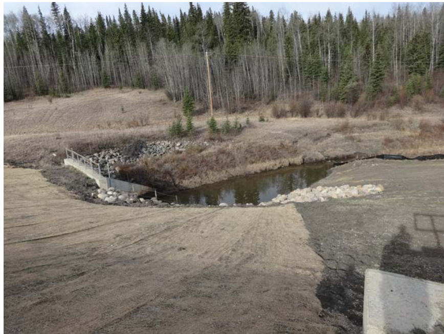
Photo 2 – Looking west at the slide repairs and arch culvert outlet from the south end of the upper pile wall at Site 3. Note the bank slump on the outside bend of the river.
