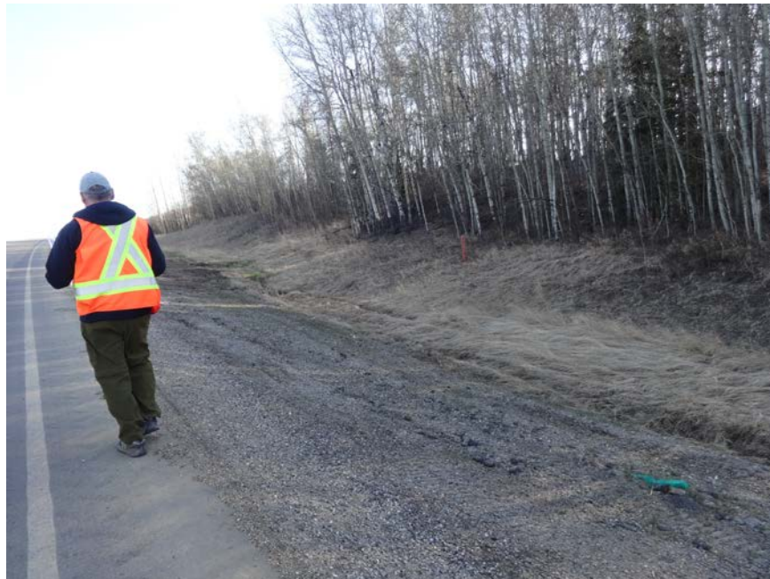
Photo 12 - Looking north along the east ditch at SI 11-3, where the slide scarp runs along the ditch between Sites 5 and 6.
