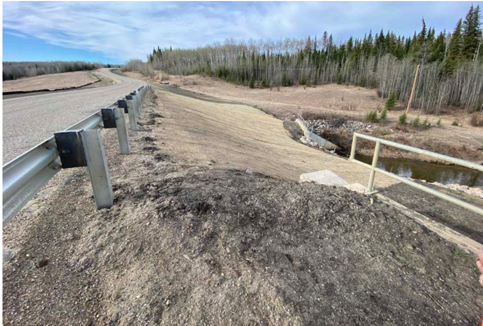
Photo 1 – Looking south along the west highway embankment south of the upper pile wall at the 2023 landslide repairs at Site 3.
